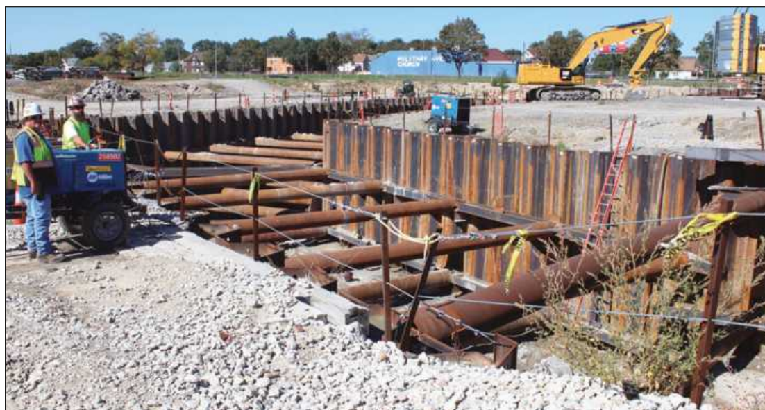
A RE-ROUTED SEWER DRAIN ditch at one of the sites associated with the Gordie Howe Bridge gets checked by (l-r) Jason Duff, a carpenters pile-driving superintendent, and Carpenters Local 687 steward Jeff Ponke. A new sewer drain "siphon" bypass will be installed at the site in Southwest Detroit, in order to bypass underground construction at the new U.S. Point of Entry.
