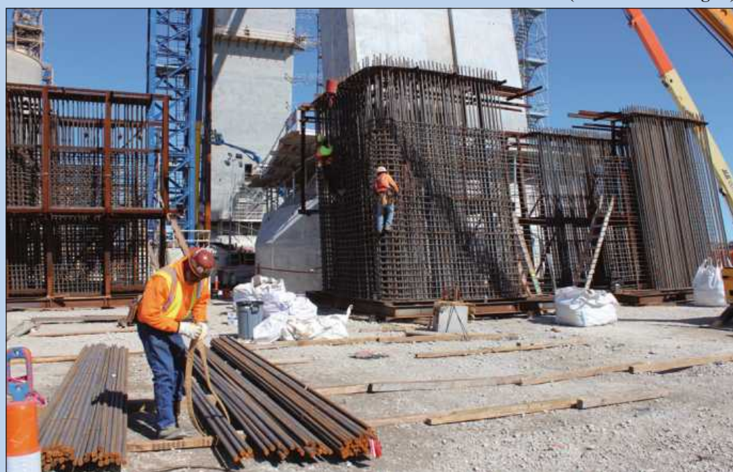
BUNDLING RE-ROD for use in the construction of a “template” form behind him on the U.S.-side tower of the Gordie Howe Bridge is Albert Montgomery of Iron Workers Local 25. He's employed by Black Swamp Steel Co.
