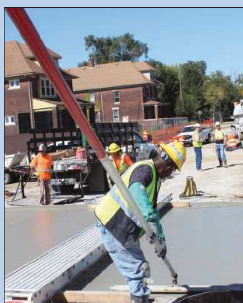
FINISHING THE SURFACE of the Livernois overpass at I-75 is Damon Meriweather of Cement Masons Local 514.
