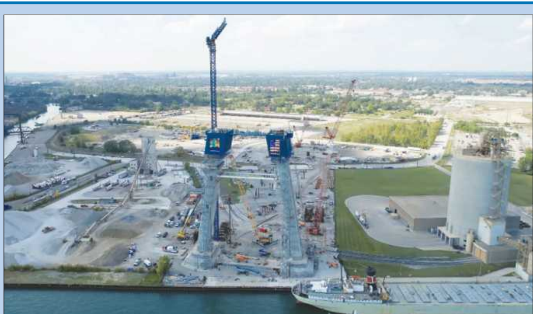
THE CONCRETE TOWERS that will support the U.S. side of the Gordie Howe Bridge to Canada rise in Southwest Detroit. The twin towers, currently 250 feet tall, will nearly triple that height when the project is complete. The 183-foot-tall Lafarge cement silo, the largest in North America when it was completed in 2004, continues operations at right, with the company's ship Alpena shown docked on the Detroit River.
