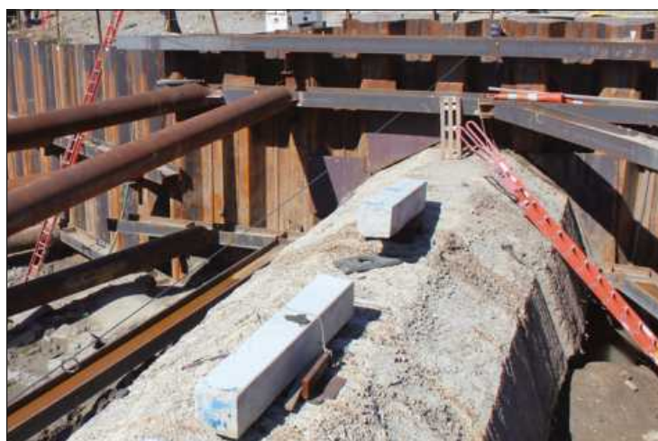
BURIED FOR 102 YEARS, THIS 12-foot diameter concrete-encased sewer pipe still looks good, and it's still leak-free. It will be tapped into and re-routed around the U.S. Point of Entry in an area around Fort Street and Junction in Detroit.
