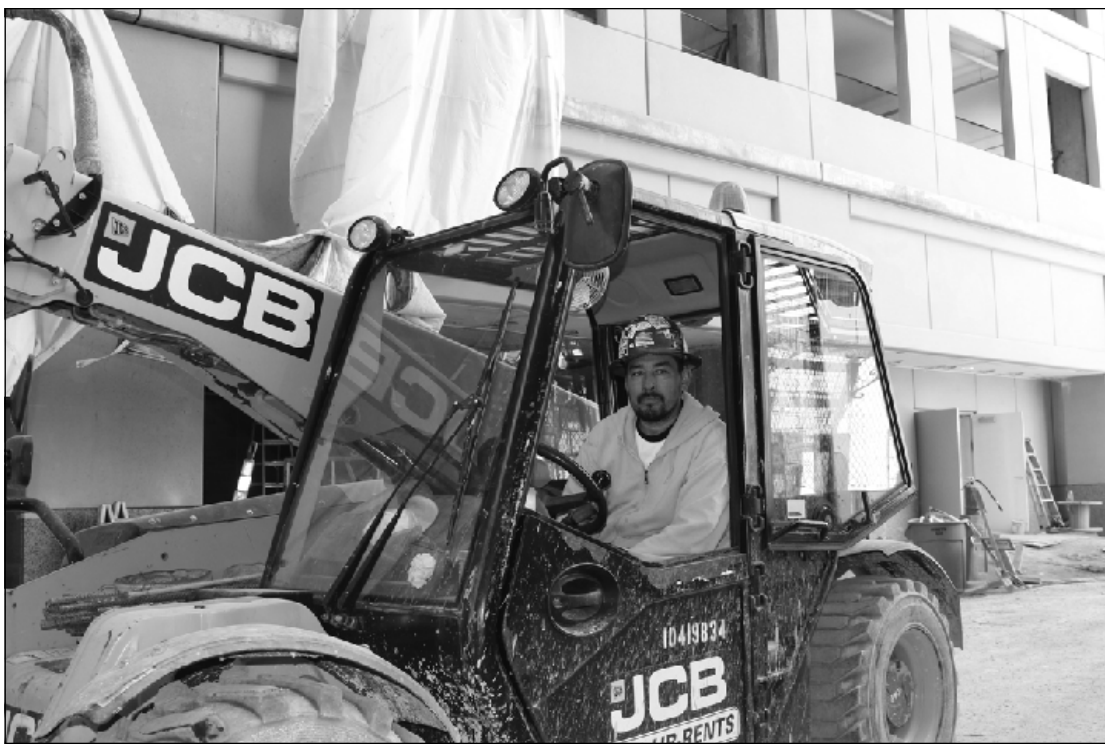
MOVING GLASS PANELS with a JCB Telehandler/loader at the Huntington Bank tower project in Detroit is Al Hernandez of Operating Engineers Local 324. He's employed by Contract Glazing Inc.
