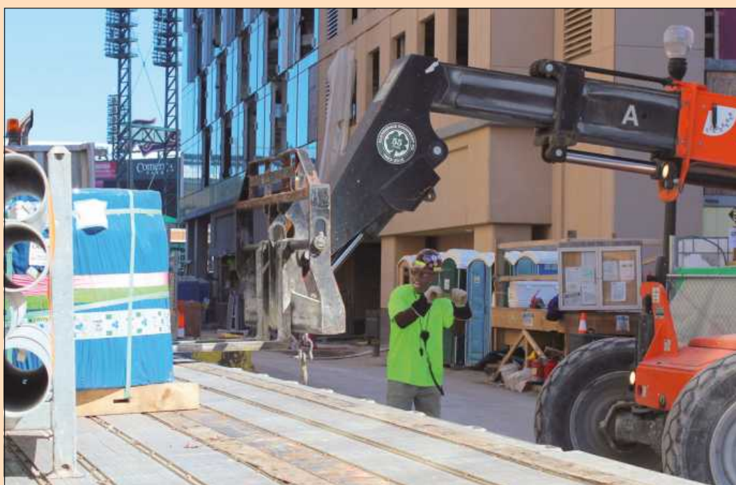
EMBRACING THE ROLE of "expediter" at the Huntington Bank headquarters project in Detroit, Laborers Local 1191 steward Andre Andrews directs a forklift operator offloading material from a flatbed. Working in tight quarters next to the 21-story project along Elizabeth Street in Detroit, "my job is to expedite the deliveries on the ground and keep it running around here," he said.
