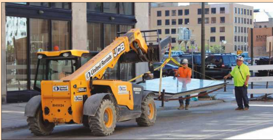
GUIDING A 10x7-FOOT exterior glass panel for a lift to the 15th floor of the Huntington Tower in Detroit are (l-r) Ralph Gaiowski and Kevin Stark of Glaziers and Glassworkers Local 357. They're employed by Contract Glazing Inc.
