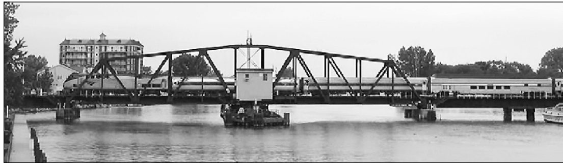
A CENTER PIVOT in the middle of the St. Joseph River provides the primary support for a 1904 rail bridge that is today owned by the CSX railroad. Here the movable span carries an Amtrak train on the Pere Marquette line between Grand Rapids and Chicago. The 231-foot-long truss bridge is typically swung open to allow for the passage of boat traffic on the river.
