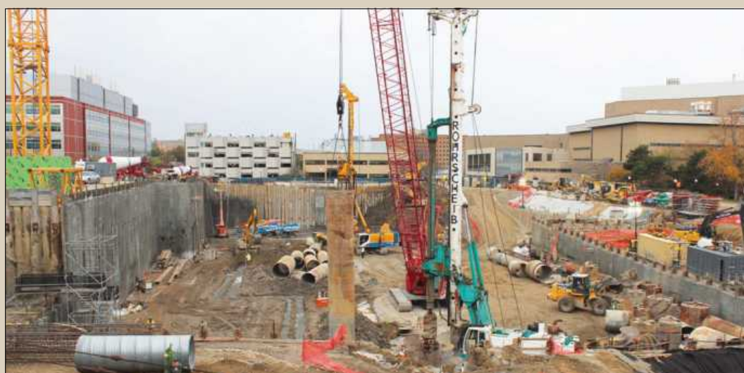
UNDER CONSTRUCTION ON what was largely green space at the University of Michigan Medical Center in Ann Arbor is the foundation work for the new 12-story hospital that will house The Pavilion at University of Michigan Health. At the center, ongoing caisson installation will anchor the building.
