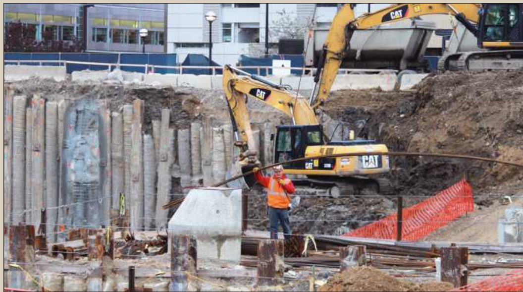
TALKING TO THE SITE'S tower crane operator, rodbuster Brandon Krel directs the movement of a bundle of reinforcing rod. The newly graduated journeyman Iron Workers Local 25 member is working for City ReSteel at the University of Michigan's Clinical Inpatient Tower hospital project in Ann Arbor.
