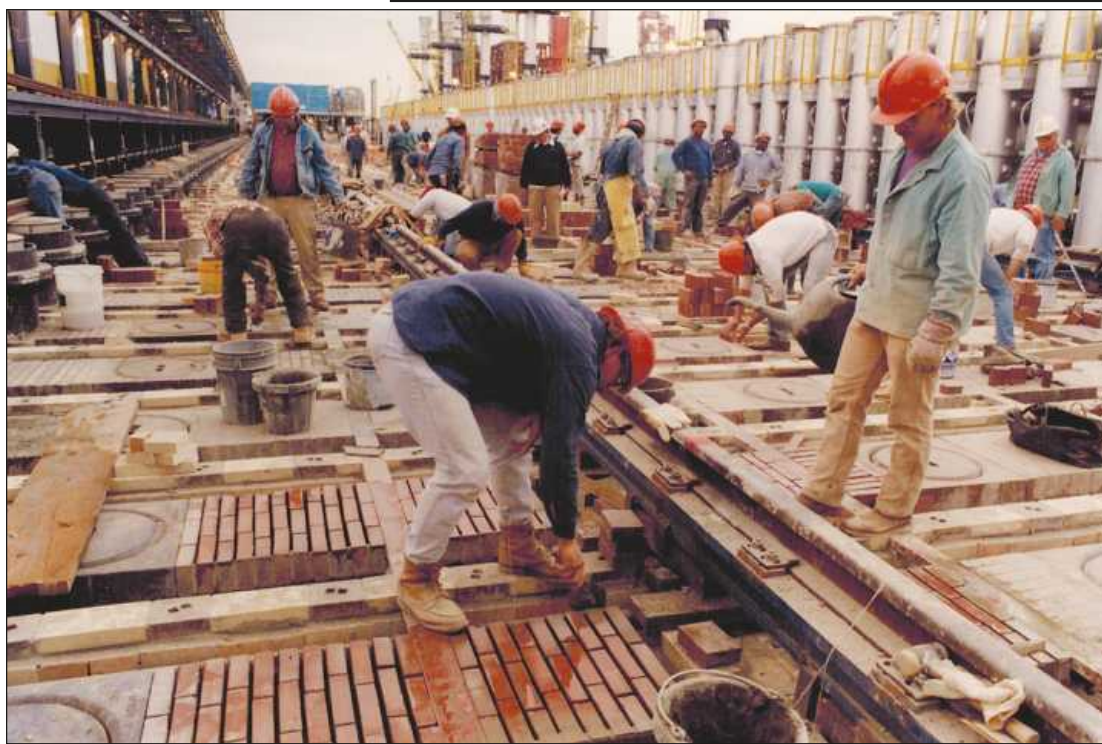
IN THIS NOVEMBER 1992 photo, one of the largest jobs ever for Detroit-area bricklayers was wrapping up—construction of a $320 million, 85-oven coke battery on Zug Island. This photo shows Chad Hopson grouting brick, while Bruce Gergel pours water on the brick to cool it, since the ovens below had already been fired. Thousands of brick were laid as part of the construction of the massive oven, now operated by DTE Energy. Tradesman file photo
