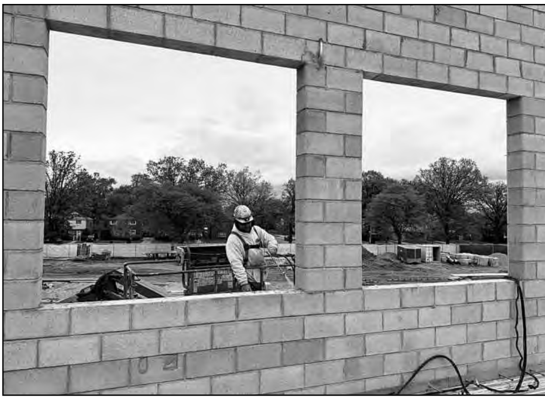
SETTING UP A VAPOR BARRIER on an a wall at the new Cody High School project in Detroit is Rob Keller of Bricklayers and Allied Craftworkers Local 2. He's employed by Industrial Services.
