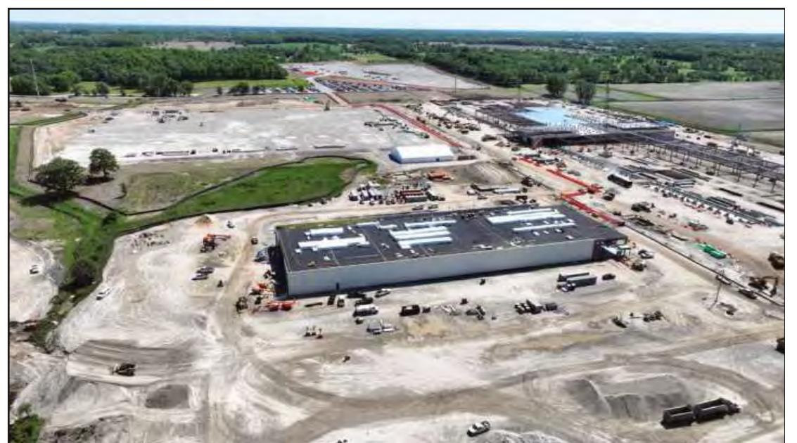
SET ON 255 ACRES in Saline Twp. in Washtenaw County, construction of the Stargate Michigan Data Center is already employing 700 building trades workers. The project is being managed by Walbridge, which ranked No. 26 in the nation by revenue on the ENR's annual contractor rankings. At $46 billion to $56 billion, it will be the largest single investment in Michigan history.
