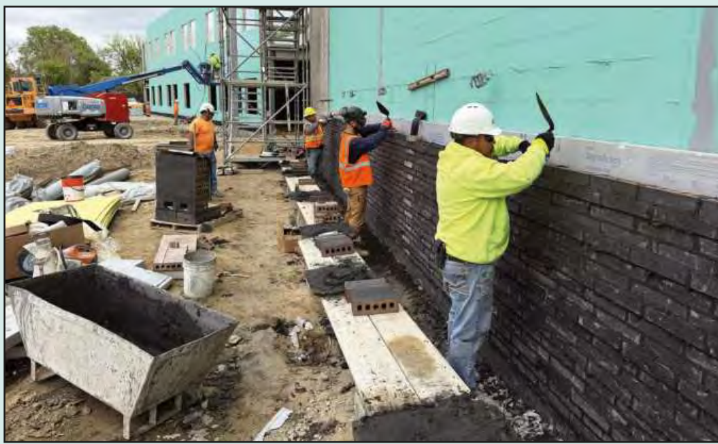
LAYING A BRICK WALL at the new Cody High School project in Detroit are Bricklayers and Allied Craftworkers Local 2 masons Adrian Martinez, Matthew Woods, Armando Alvarado and Marco Garay. They're employed by Baker Construction.
