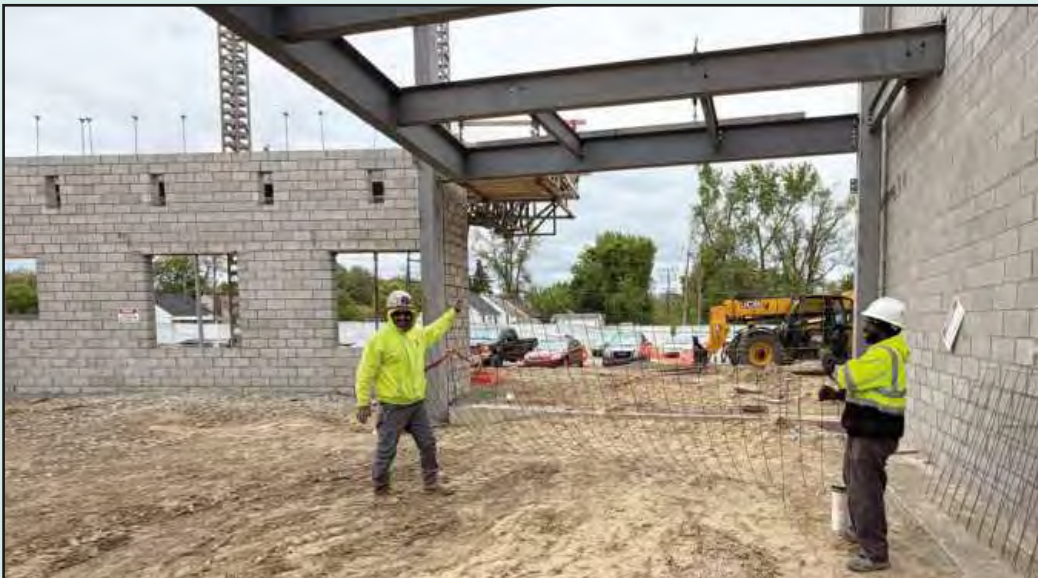
MANEUVERING wire mesh to set in concrete at the Cody High School project in Detroit are (l-r) John Rizzo of Cement Masons 514 and Dion Coleman of Laborers Local 1075. They're employed by J.J. Barney Construction.
