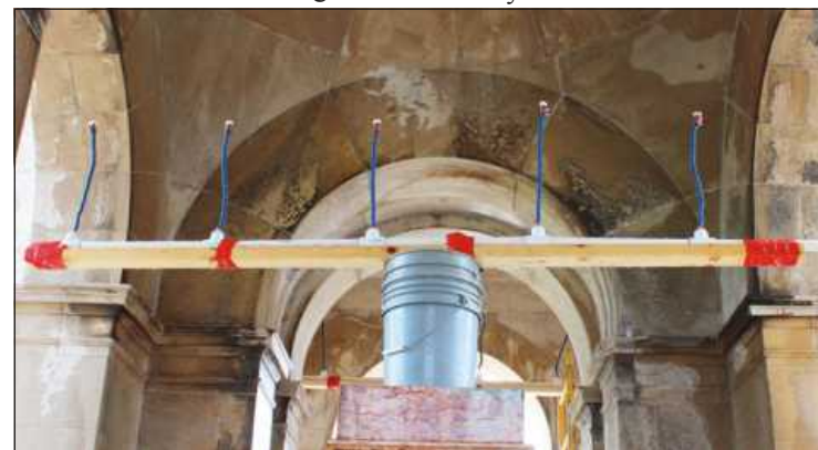
A SET AND FORGET system of nozzles fashioned by Ram Construction Services shoots water into the ceiling of the interior of the Hurlbut Gate, and can clean the limestone for hours at a time without supervision.
