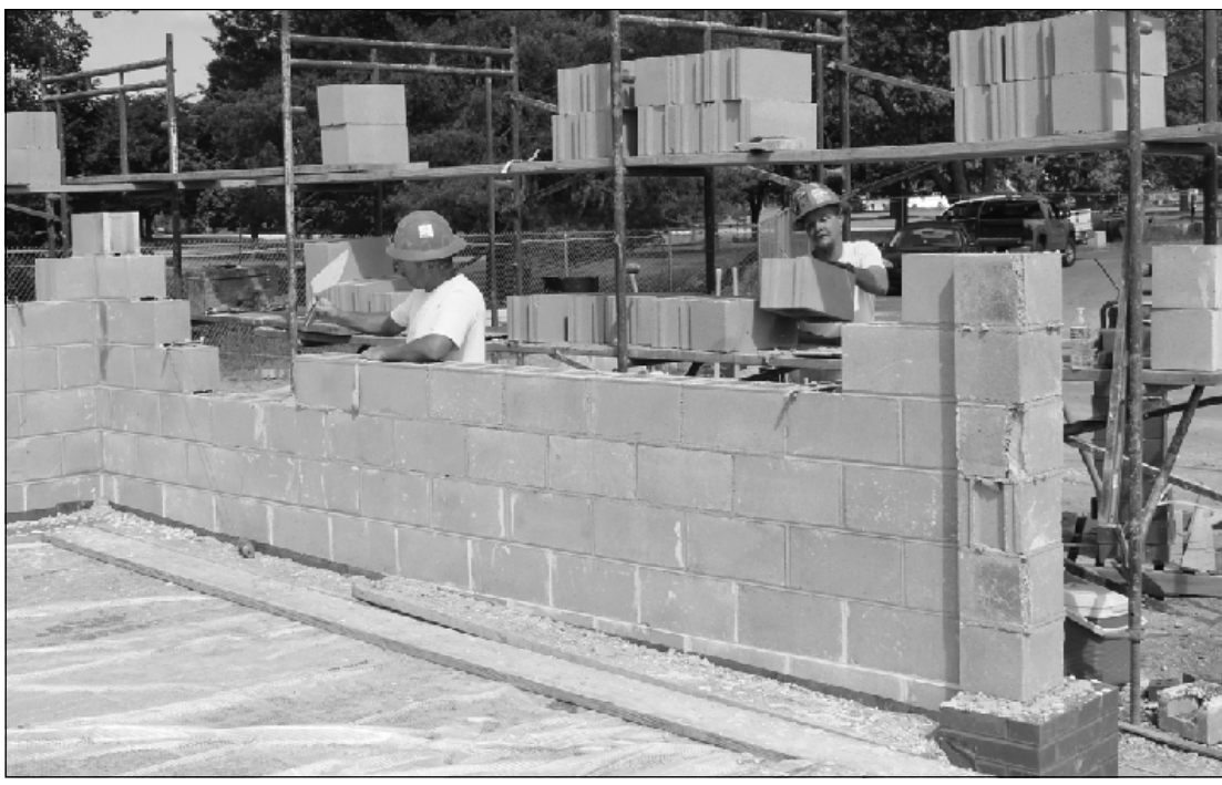
BUILDING A BLOCK wall to enclose dumpsters at the Caro Psychiatric Hospital site are (l-r) Troy Tripp of Bricklayers and Allied Craftworkers Local 2 and Matt Denay of Laborers Local 1098. They're employed by Boettcher Masonry.
