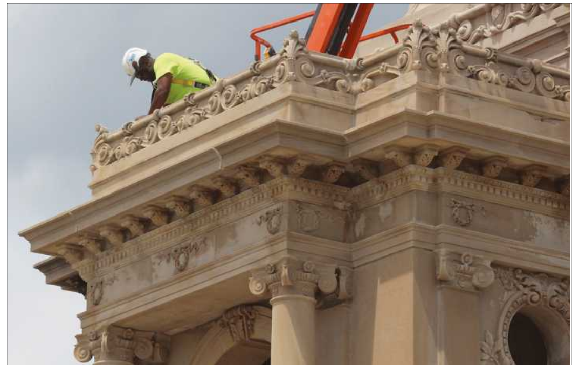
BRICKLAYERS AND ALLIED Craftworkers Local 2 apprentice Theodore Ravetta works on the limestone in the upper reaches of the ornate Hurlbut Gate. He's employed by Ram Construction Services.
