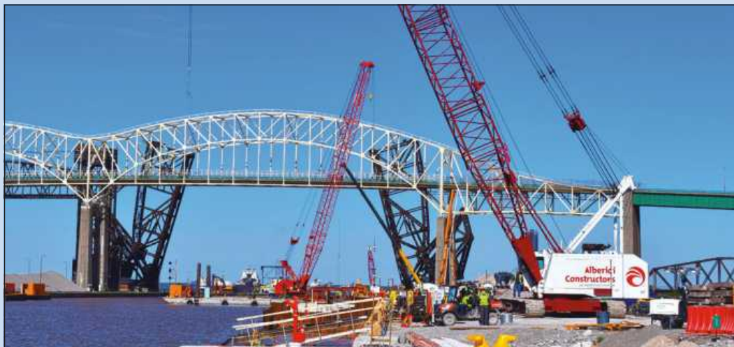
WITH THE FIRST PHASE channel deepening complete at the Soo Locks, the trades turn their attention to the second phase — rehabilitating the upstream approach walls. That phase of the project started last year and is being undertaken by Kokosing-Alberici. "That's rehabbing the walls leading to the lock," said U.S. Army Corps of Engineers Project Engineer Kristina Schnettler, to Operating Engineers Local 324, "because those walls are over 100 years old and in disrepair."
