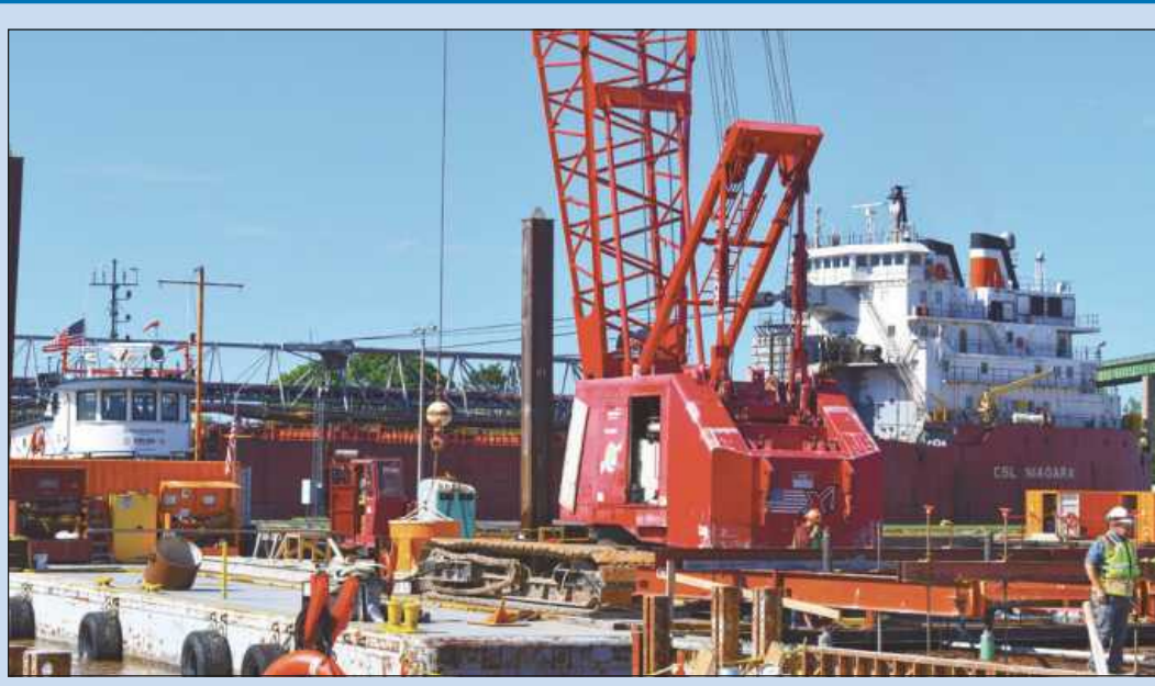
THE BULK CARRYING freighter CSL Niagara rises through the Soo Locks in front of a Local 324 crane operator at the controls of a Manitowac 4000W. The second phase of the construction of a new lock in Sault Ste. Marie has been under way for the past year under the contracting team Kokosing-Alberici LLC.
