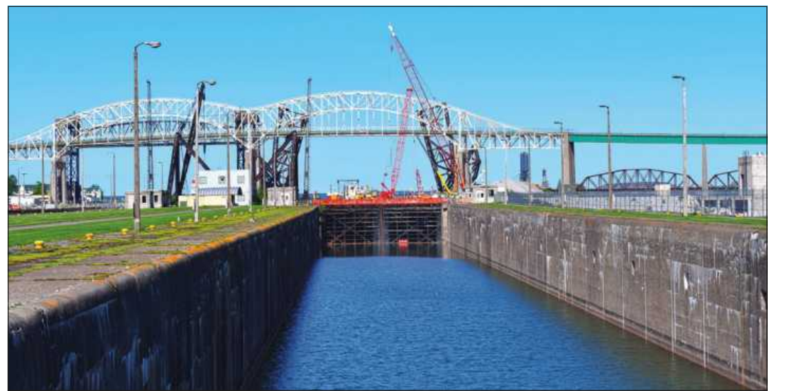
THE SOO LOCKS is hosting tons of heavy equipment in recent months, with more than 30 Operating Engineers Local 324 members on the job. Here we see a lock in operation with the International Bridge in the background. Photo credit: Dan McKernan/Operating Engineers Local 324
