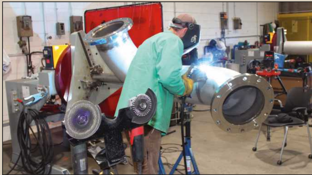
WELDING A 10-INCH stainless pipe for a methane piping project in Michigan at the Shouldice shop in Battle Creek is Jim Griffiths of Plumbers and Pipe Fitters Local 333.
