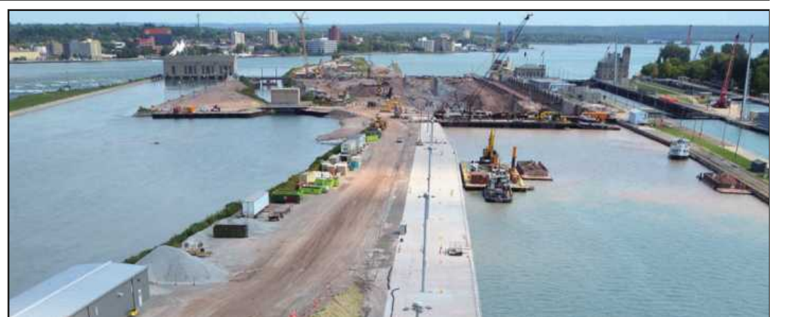
CONSTRUCTION OF MASSIVE new upstream concrete approach walls at the Soo Locks was the main task on this year's agenda for the U.S. Army Corps of Engineers, and it was mission accomplished. Phase 2 work focused on rehabilitating the upstream approach walls, in the center of the photo, to guide vessels into the new Soo lock and allow vessels to moor on the wall.
