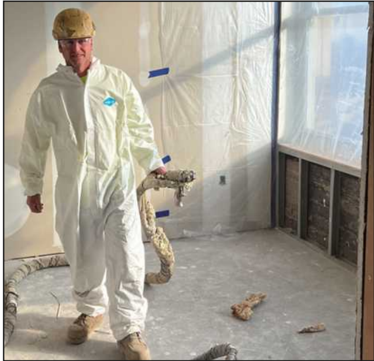
SETTING UP THE APPLICATION of insulating spray foam on 18th-floor walls of the 150 Bagley project is Eric Soave of Heat and Frost Insulators Local 25. He's employed by Stony Creek Services.
