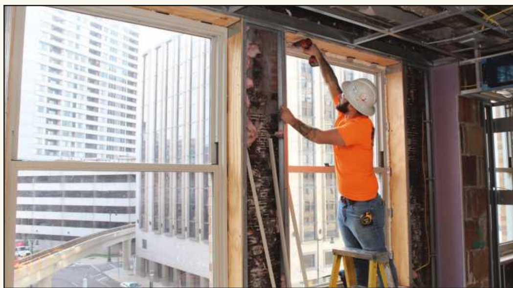
SETTING BOX TRIM on a fourth floor window at the Residences @ 150 Bagley project in Detroit is Evan Boyajian of Glaziers and Glassworkers Local 357. He's employed by Universal Glass.
