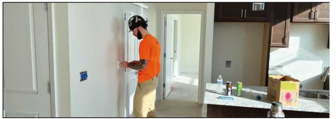
WIRING AN ELECTRICAL box in a 14th floor apartment at the 150 Bagley project in Detroit is Frank Licavoli of IBEW Local 58. He's employed by Edgewood Electric.
