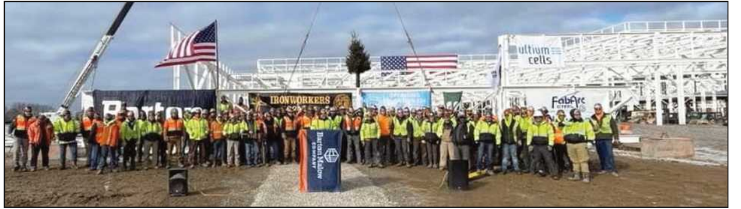
MEMBERS OF IRON WORKERS Local 25 and Operating Engineers Local 324 employed by Barton Malow commemorate the topping out of the GMLG Ultium Battery Plant in Lansing on Feb. 24.
