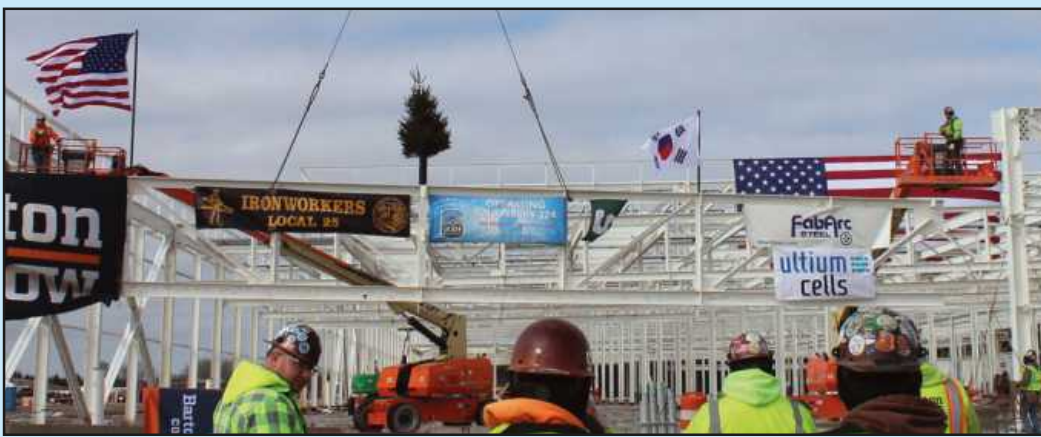
IRON WORKERS Local 25 connectors Brett Fath and Nick Place set the final truss into place at the Ultium Cells Lansing Plant, with the traditional topping-out evergreen, flag and banners along for the ride. Barton Malow is managing the project and self-performing the steel work.
