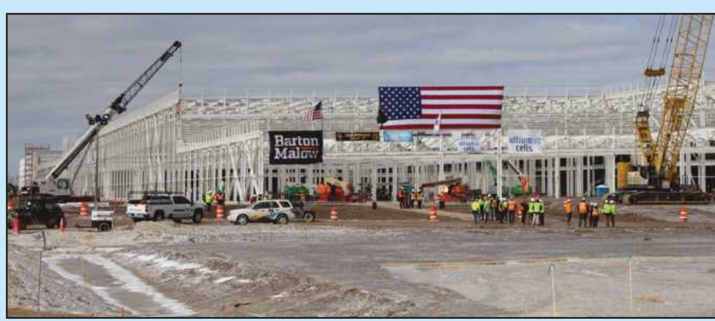
THE LAST SECTION OF STRUCTURAL steel, a truss, is shown as set on Feb. 24 at the Ultium Cells Lansing Plant after most of the attendees at the ceremony dispersed. Construction continues under project manager Barton Malow at the massive 2.8 million-square-foot plant, which will produce electric vehicle batteries for GM.
