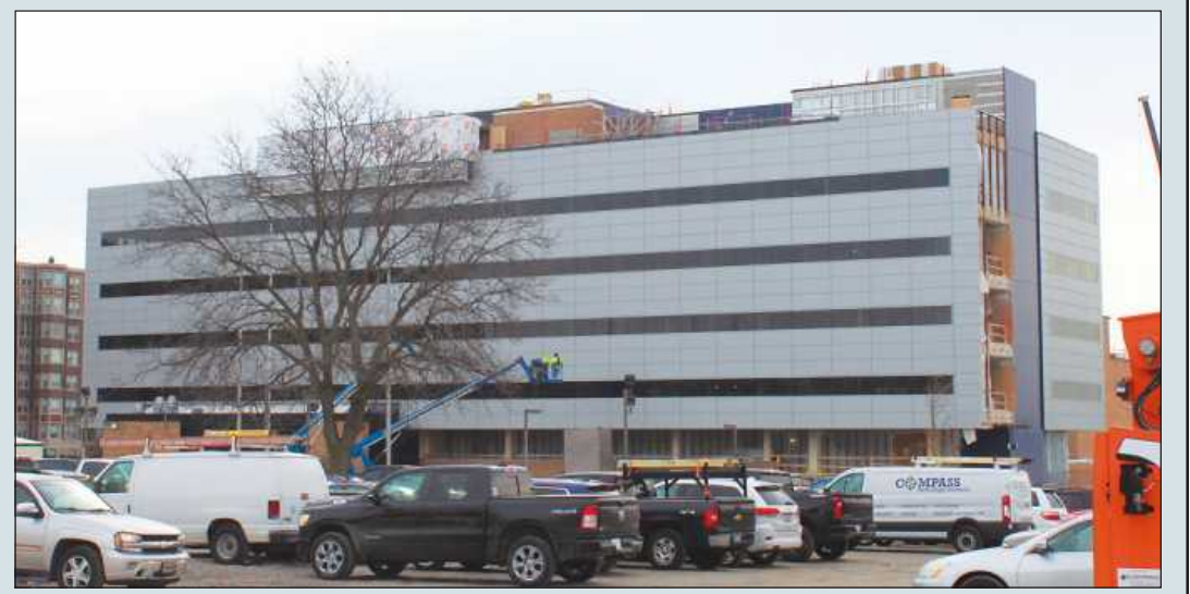
THE SIX-STORY headquarters for the United Auto Workers, aka "Solidarity House," is undergoing repairs by trades workers after a third-floor fire. Completed in 1951 along East Jefferson on Detroit's riverfront, the building encompasses more than 165,000-square-feet of space, and underwents multiple subsequent additions and mechanical renovations over the years.
