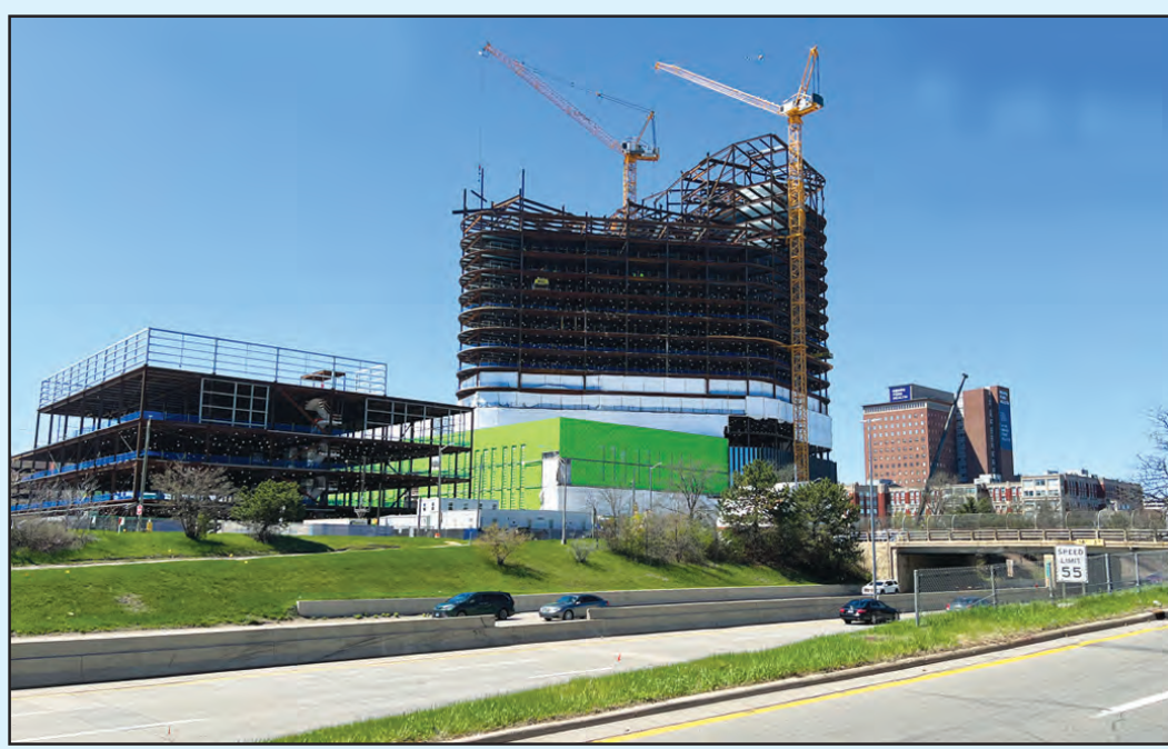
SEEN FROM ACROSS the Lodge Freeway in Detroit, the most prominent part of Henry Ford Health's Destination Grand is the new 20-story patient tower that's under construction. Leading the project are Barton Malow, Turner Construction and Dixon Construction Services. The red brick tower at the right is a 17-story, 1955 addition to the original Henry Ford Hospital. Both facilities will face each other across West Grand Boulevard.
