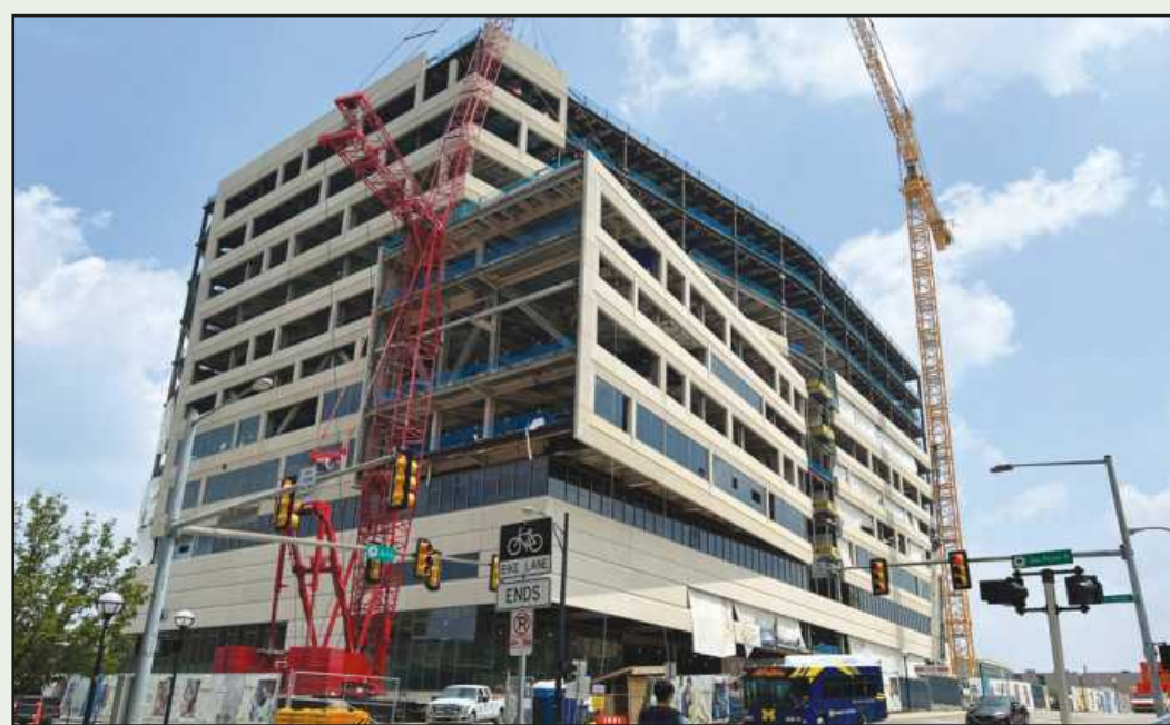
Michigan Medicine's Health Care Pavilion in Ann Arbor is about halfway through a four-year construction process, which will yield a complex, state-of-the-art hospital.
