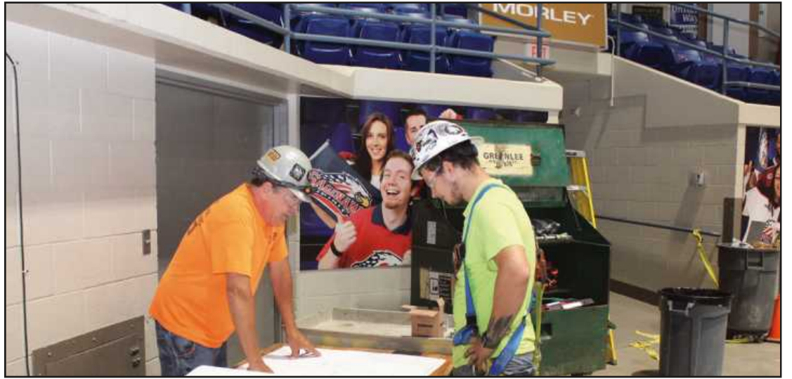
LOOKING AT PLANS for new electrical works at the Dow Events Center Arena in Saginaw are (l-r) Floyd Wildman and Jason Wilson of IBEW Local 557. They're employed by Nelson Electric.
