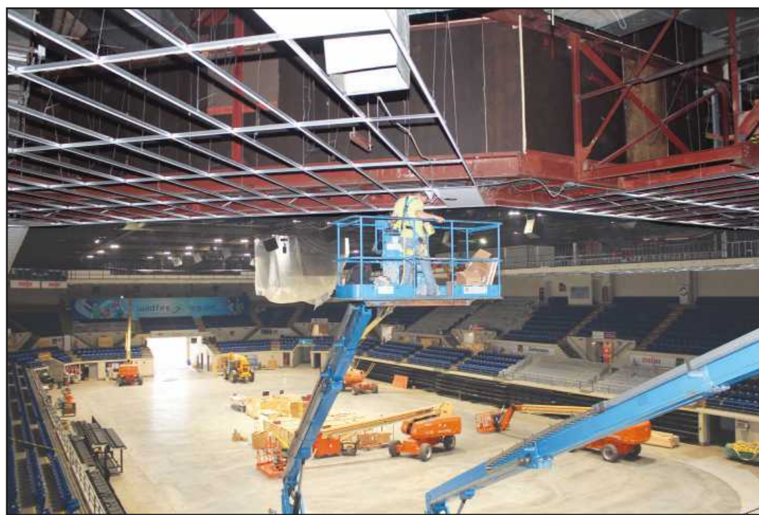
SETTING WIRING for new lights in the upper reaches of the Dow Events Center Arena in Saginaw is Jason Wilson of IBEW Local 557. He's employed by Nelson Electric.
