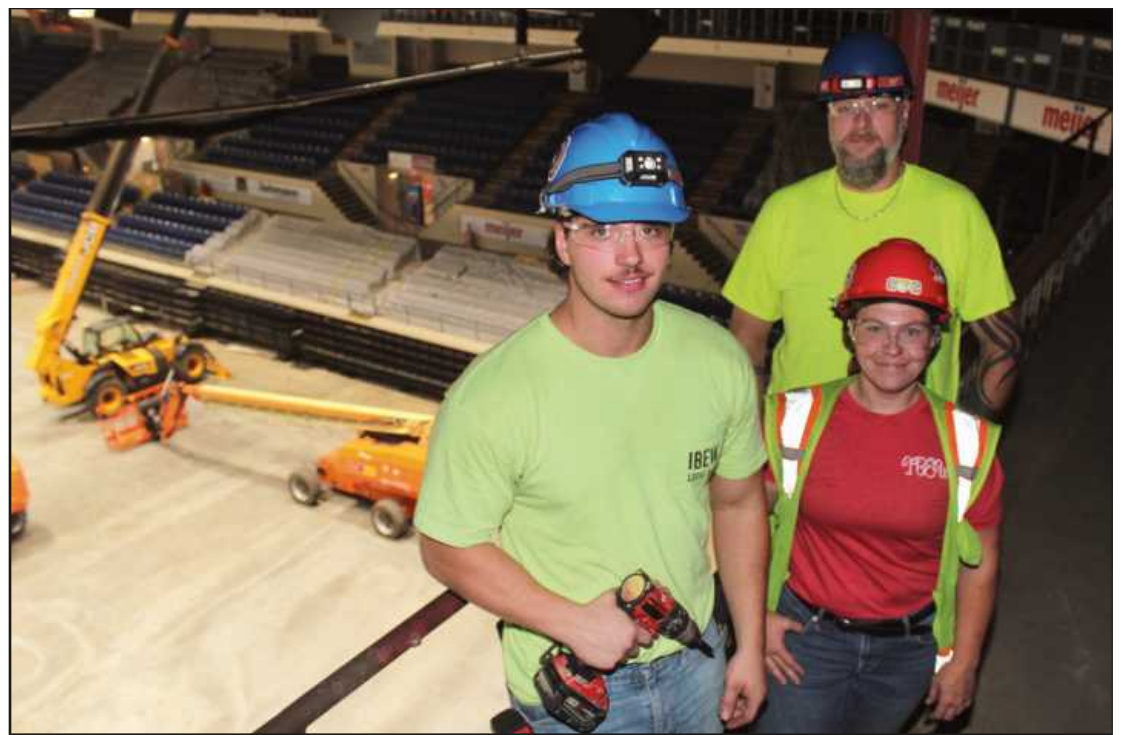
BACKED BY journeyman Chris Wright, first-year apprentice Jake Schultz and fifth-year apprentice Breanna DePottay work in the upper reaches of the Dow Event Center Arena in Saginaw. The IBEW Local 557 members are employed by Nelson Electric.
