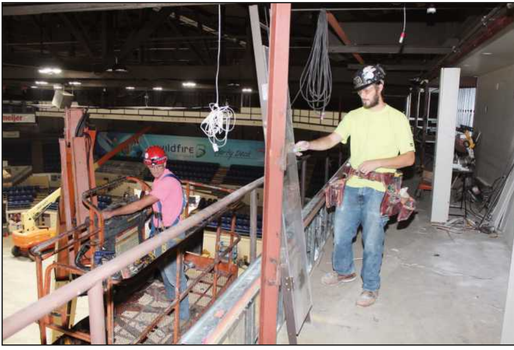
INSTALLING DRYWALL panels in the upper reaches of the Dow Events Center Arena in Saginaw are Darrick Morley and James Severn of Michigan Regional Carpenters Council Local 706. They're employed by Tri City Acoustical.
