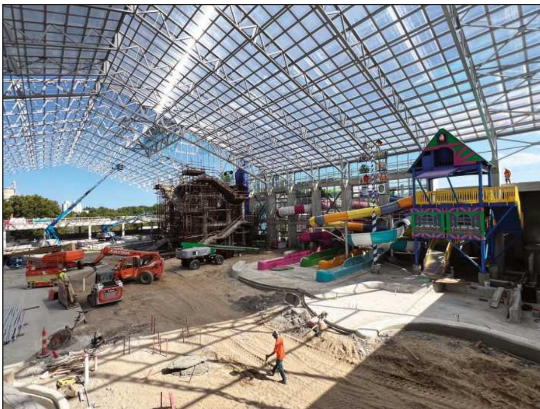
THE NEW WATERPARK under construction at the Bavarian Inn in Frankenmuth. R.C. Hendrick and Son is managing the $90 million project, which is expected to make Michigan's "Little Bavaria" an even bigger draw for tourists to Saginaw County.
