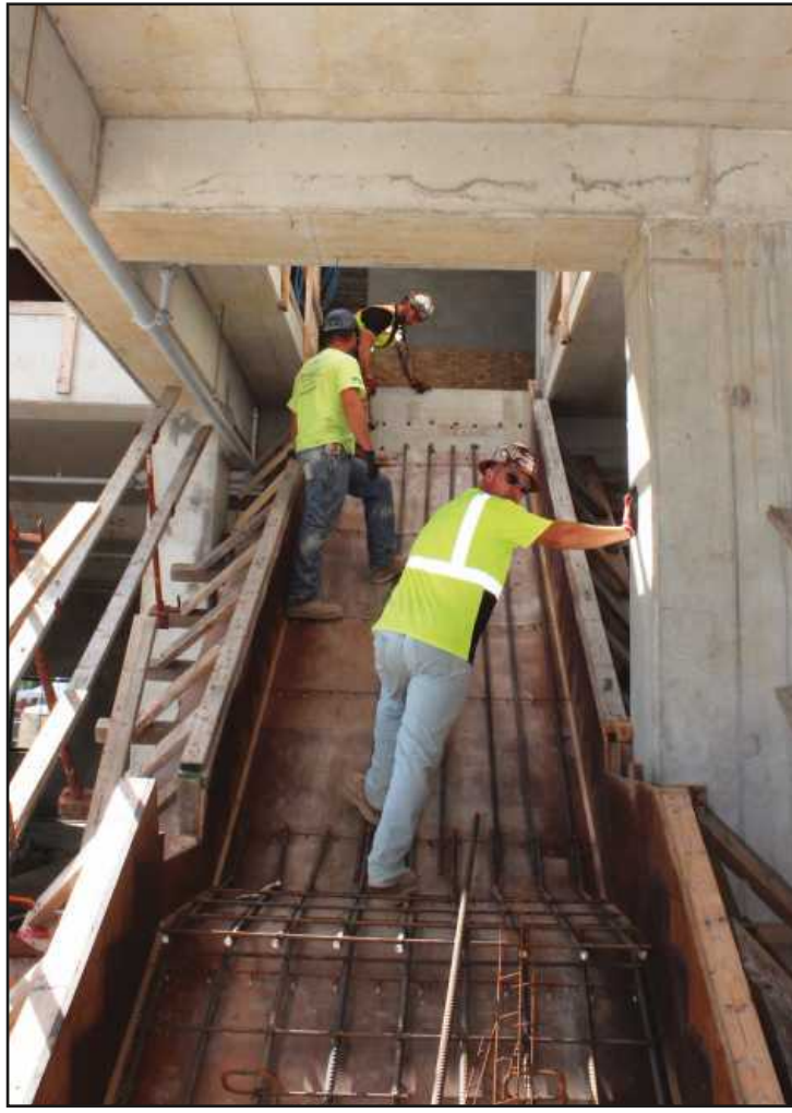
SETTING REINFORCING ROD for a stairway to the mezzanine deck at the Bavarian Inn waterpark project in Frankenmuth are Local 25 rodbusters Andrew Lyons, Brett Wicke and Adam Peterson. They’re employed by City ReSteel.
