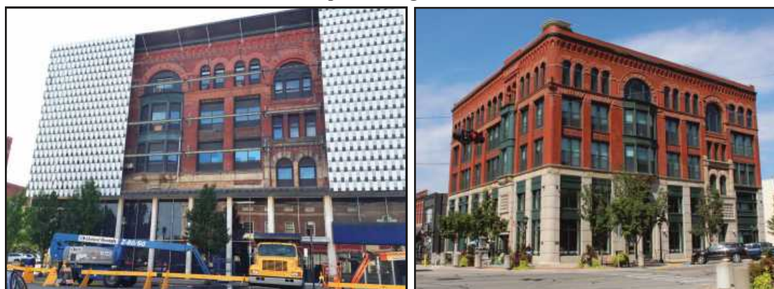
THE CHEESE GRATER siding is partially removed, at left, from the Crapo Building in 2018. At right is a summer 2024 photo of the restored building at Washington and Center avenues.
