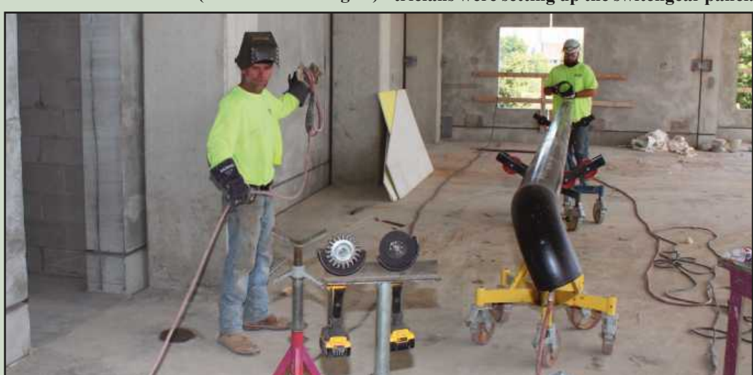
SETTING UP A WELD on a 6-inch Schedule 40 pipe at the Bavarian Inn waterpark project are (l-r) B.J. Elder and Nicholas Vanooteghem. The Plumbers and Steamfitters Local 85 members are employed by Remer Plumbing and Heating.
