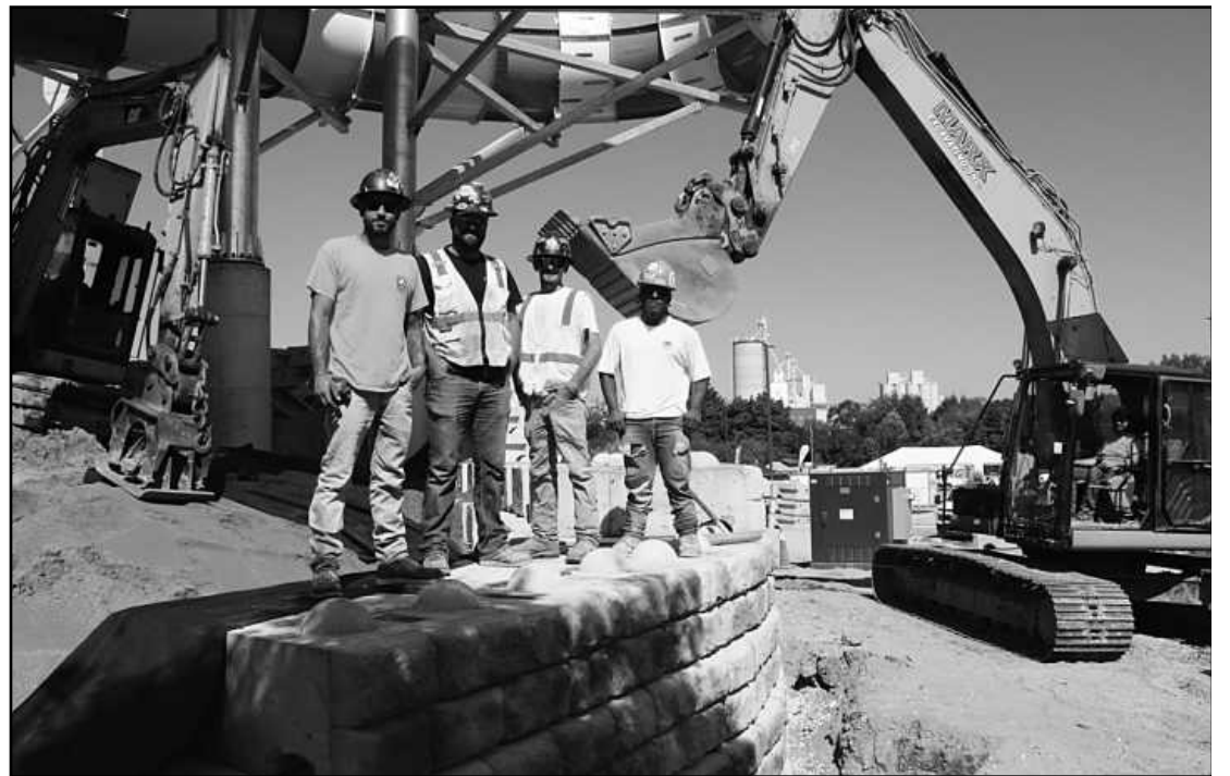
NICE, SOLID RETAINING WALL – It was erected at the Barvarian Inn waterpark by this ground of laborers and operators. Atop the wall are Nate Fulgencio (Laborers Local 1075); Corey Cuthbertson (Operating Engineers Local 324); Tyler Kanyo (Laborers Local 1098), and Anthony Askey (Local 1098). In the excavator is Trevor Johnson of Local 324.
