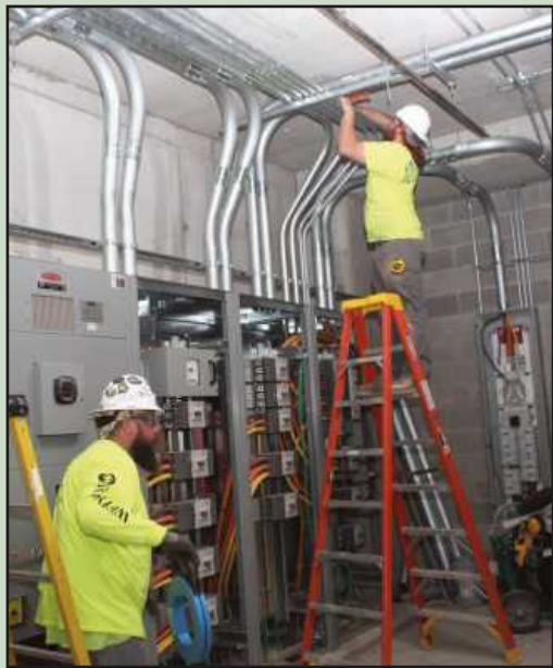
PULLING WIRE AND installing conduit in space next to the operating Bavarian Inn in Frankenmuth are electricians (l-r) Kevin Denton and Benjamin Bauman. Employed by Weinstein Electric, the IBEW Local 557 electricians were setting up the switchgear panel.
