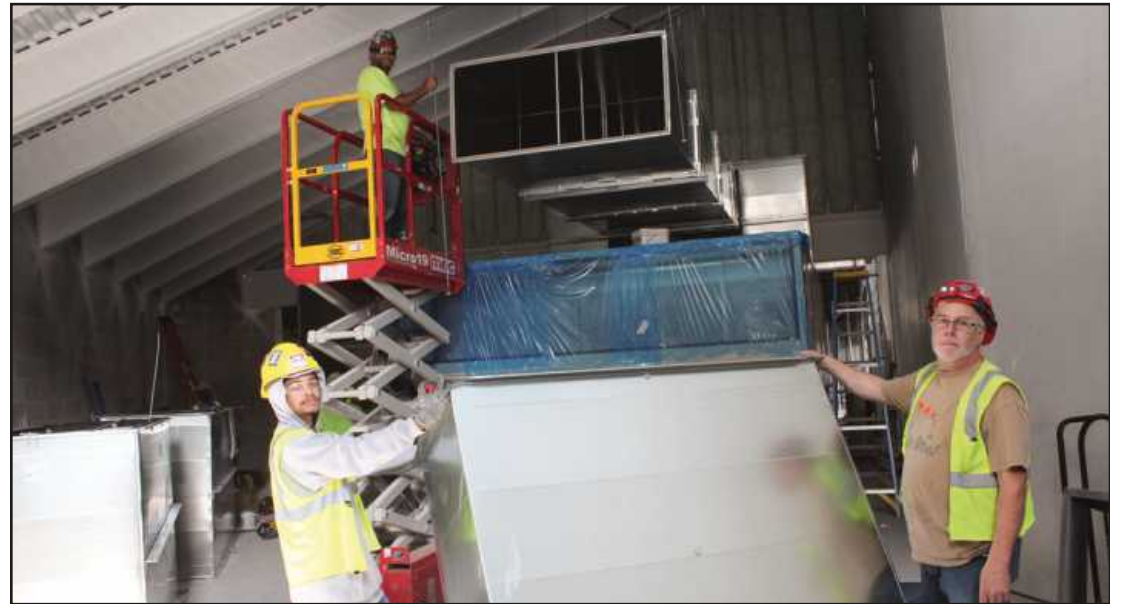
READY TO MOVE A supply duct into place at the Bavarian Inn waterpark in Frankenmuth are a trio of Sheet Metal Workers Local 7 members. They include (l-r) Tristan Douglas and Jon Pritchard, below, and Kevin Isberg on the lift. They're employed by U.S. Sheet Metal.
