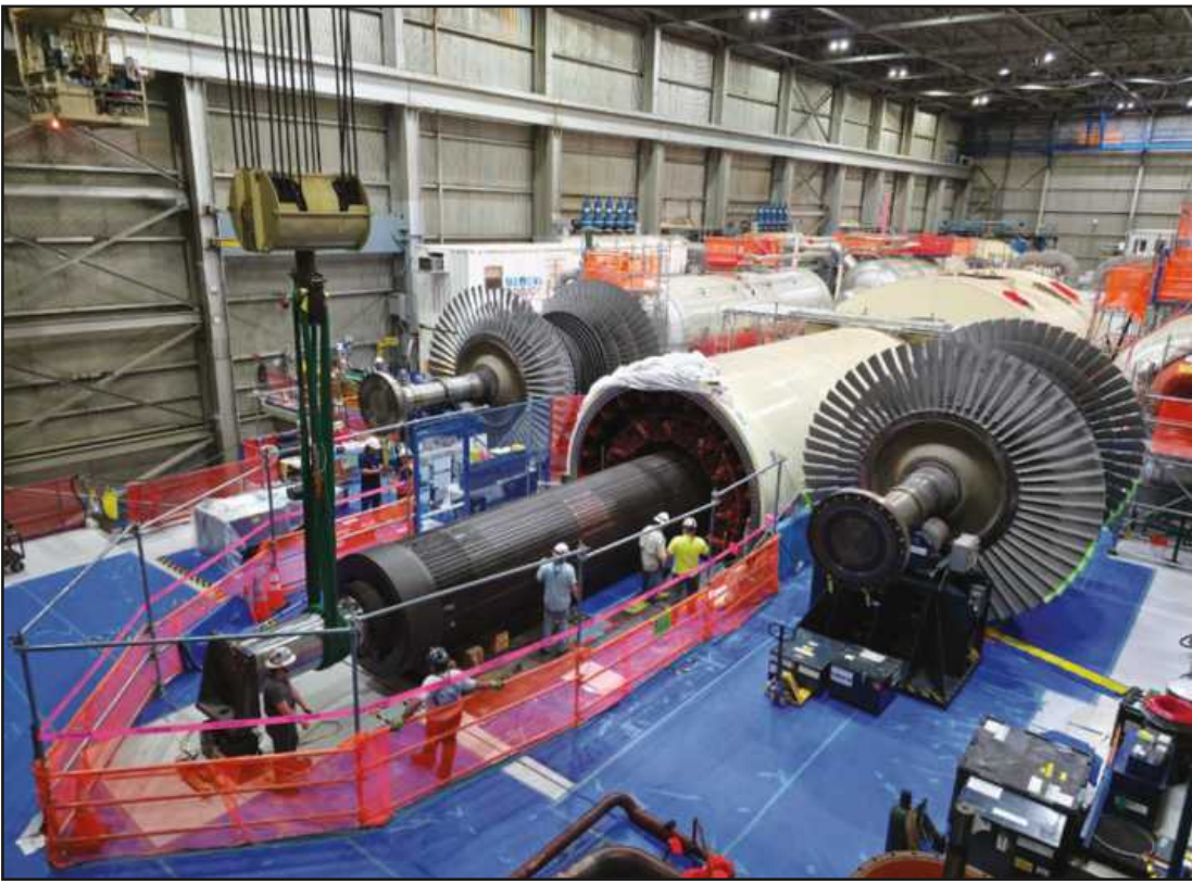
TURBINE ROTOR inspection takes place at the Palisades Nuclear Power Plant.
