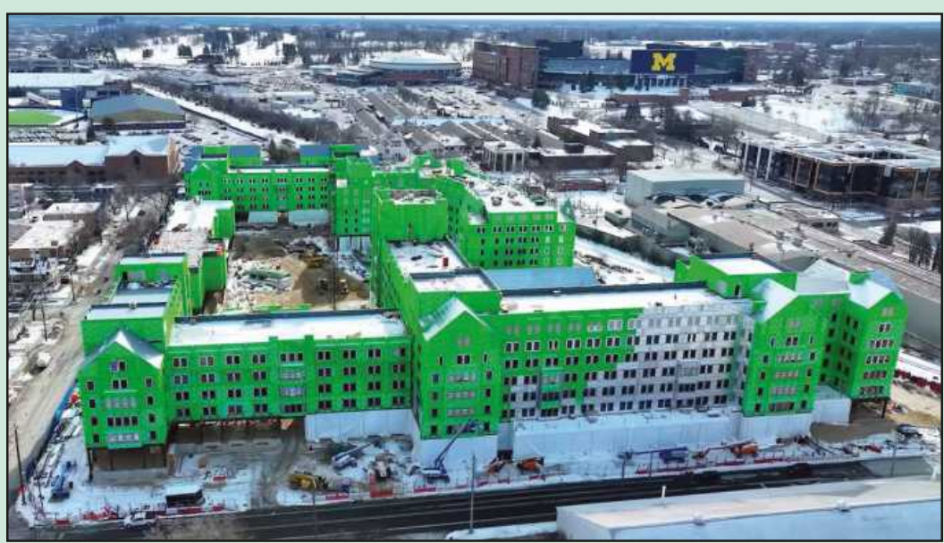
FIVE BUILDINGS comprise the $631 million Central Campus Residential Development at the University of Michigan in Ann Arbor. U-M is going big to address the chronic lack of undergraduate residential space on campus.
