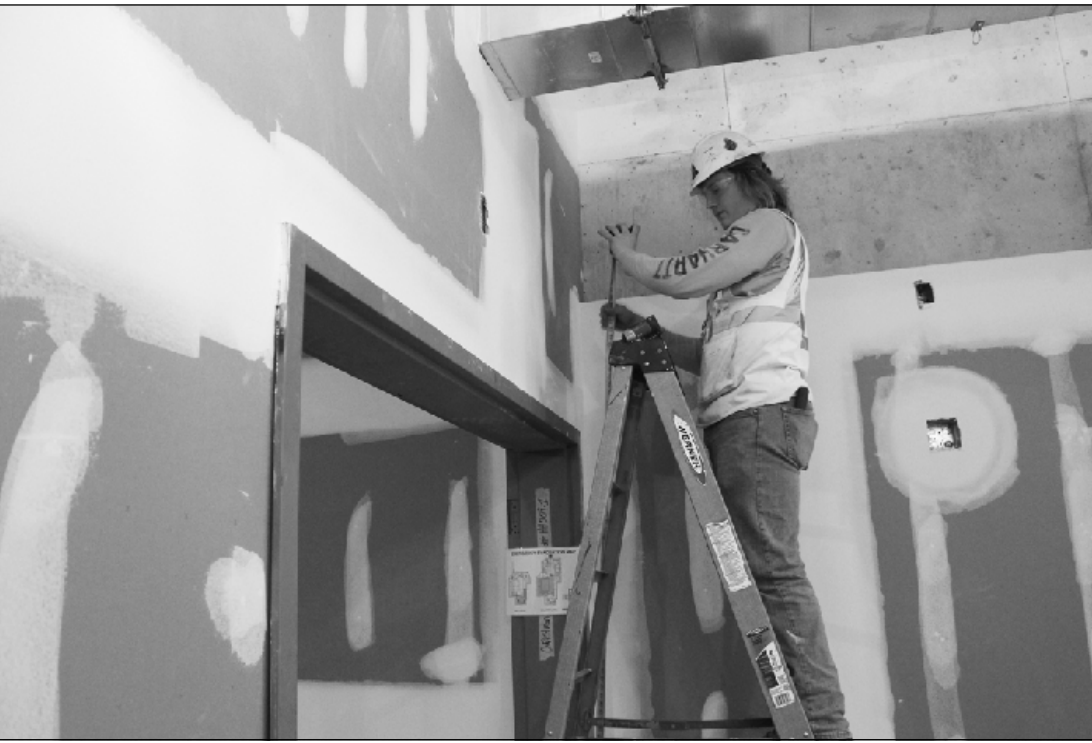
AT WORK AT the Heritage Hall project at the Michigan Capitol Building in Lansing is Summit Electric employee Devin Kora of IBEW Local 665.
