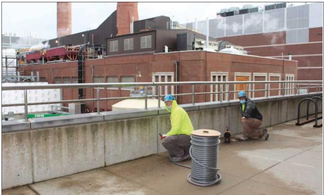
THE UNIVERSITY OF MICHIGAN Central Power Plant is the backdrop for two masons waterproofing joints on an elevated walkway on the Ann Arbor campus. At work are Bob Richmond and Paul Cyrus of Bricklayers and Allied Craftworkers Local 2. They're employed by Pullman Services.
