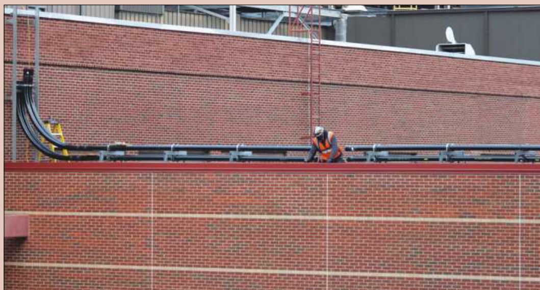
MEASURING FOR CONDUIT installation at the U-M Central Power Plant is Brett Shaner of IBEW Local 252. He's employed by Huron Valley Electric.
