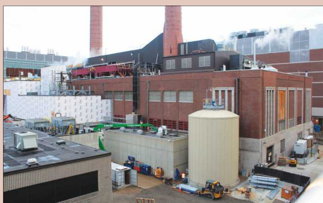
A 12,000-SQUARE-FOOT addition to the University of Michigan's Central Power Plant, the white structure, at left, will house a new 15-megawatt combustion turbine. The new turbine will increase capacity to generate more energy and move the university halfway toward its goal of reducing total emissions for the Ann Arbor campus by 25 percent by the year 2025.
