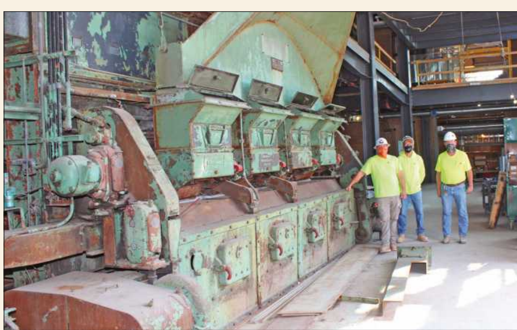
WE ASKED THIS GROUP of electricians at the end of their shift to stand next to an original "boiler skin" inside the former Shaw Lane Power Plant on the Michigan State University campus. A portion of the first-floor boiler works, dating to when the plant was in service from 1947-75, will be retained as part of the plant's renovation and expansion. The IBEW Local 665 electricians include (l-r) Allen Lepard, Mitch Frankovich and Tom Densmore. They're employed by Hayes Electric.
