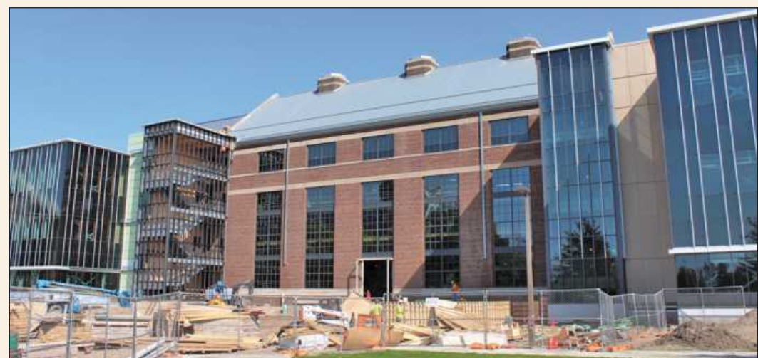
FLANKED BY ITS NORTH AND SOUTH annex additions, the original brick 1947 Shaw Lane coal-burning power plant on the Michigan State University campus in East Lansing is undergoing an unlikely, and remarkable renovation into a STEM (Science, Technology, Engineering and Math) hub for the school.
