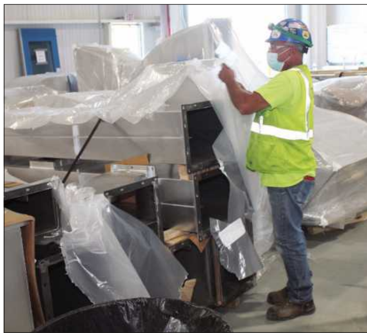
TAKING THE WRAPS off ductwork at the FCA Mack Avenue project is Randy Nagle of Sheet Metal Workers Local 7. He's employed by Giffen.
