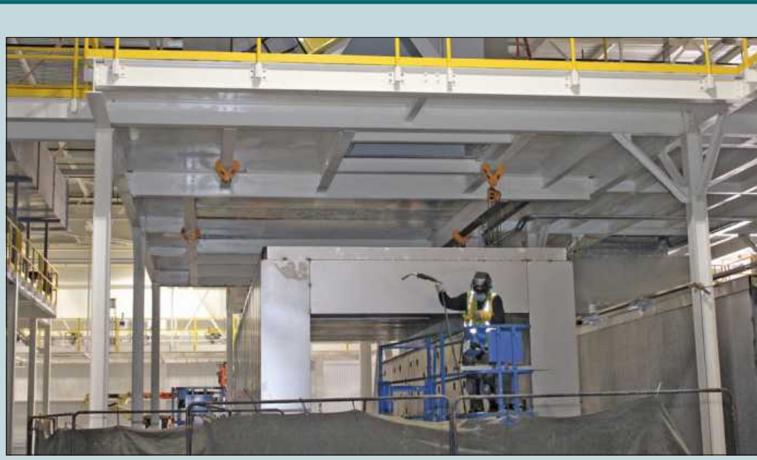
AT WORK ON A LIFT installing an over in the FCA Mack Avenue paint shop in Detroit is Antonio Ramirez of Sheet Metal Workers Local 292. He's employed by Giffin.
