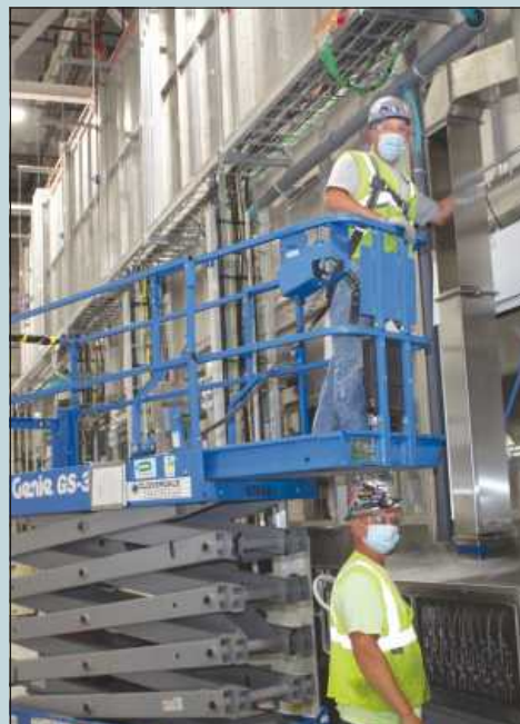
WORKING ON A PAINT LINE at the FCA Mack Avenue plant are (on the lift) Ed Hyvonen of Pipe Fitters 636 and Art Laginess of Plumbers Local 98. They're employed by John E. Green.
