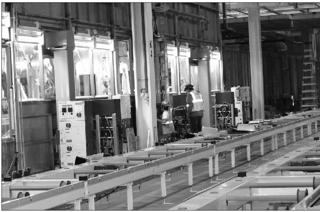
WORKING ON THE PAINT LINE on the second level of the FCA Mack Avenue Plant renovation in Detroit are Plumbers Local 98 members Mike Jantamrian and Jeff Cheresko. They're employed by John E. Green.
