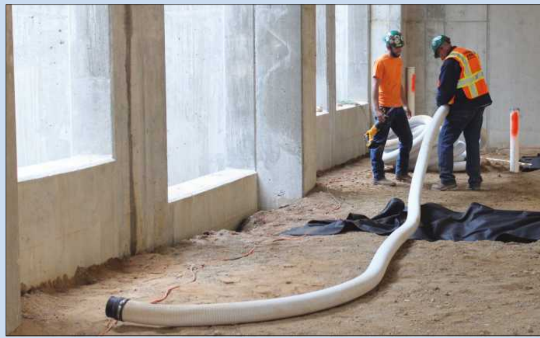
SETTING UP A PERFORATED drain tile for installation at Owosso Memorial Hospital are (l-r) Isaac Stearns and Dan Stearns of Plumbers and Pipe Fitters Local 370. They’re employed by Johnson and Wood.
