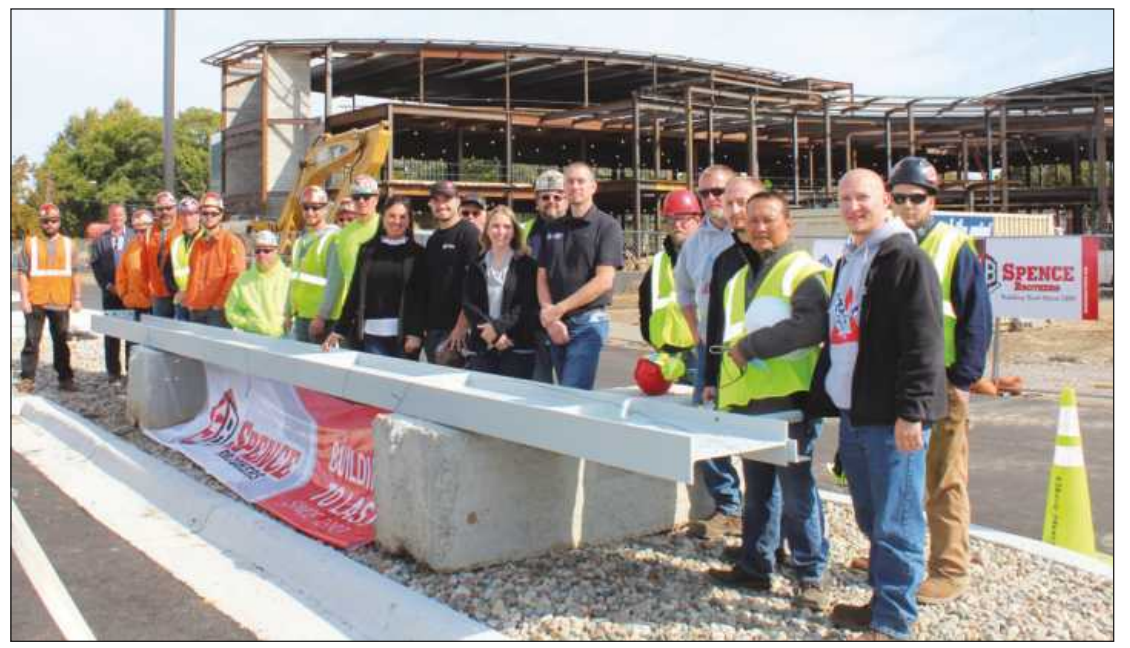
STAFF AT OWOSSO Memorial Hospital, Spence Brothers, Tri-Steel and Iron Workers Local 25 members stand behind the final structural steel beam before it's placed at the health care facility's new Memorial Healthcare Institute for Neurosciences and Multiple Sclerosis, and its orthopedic practice, Mid-Michigan Orthopedics.
