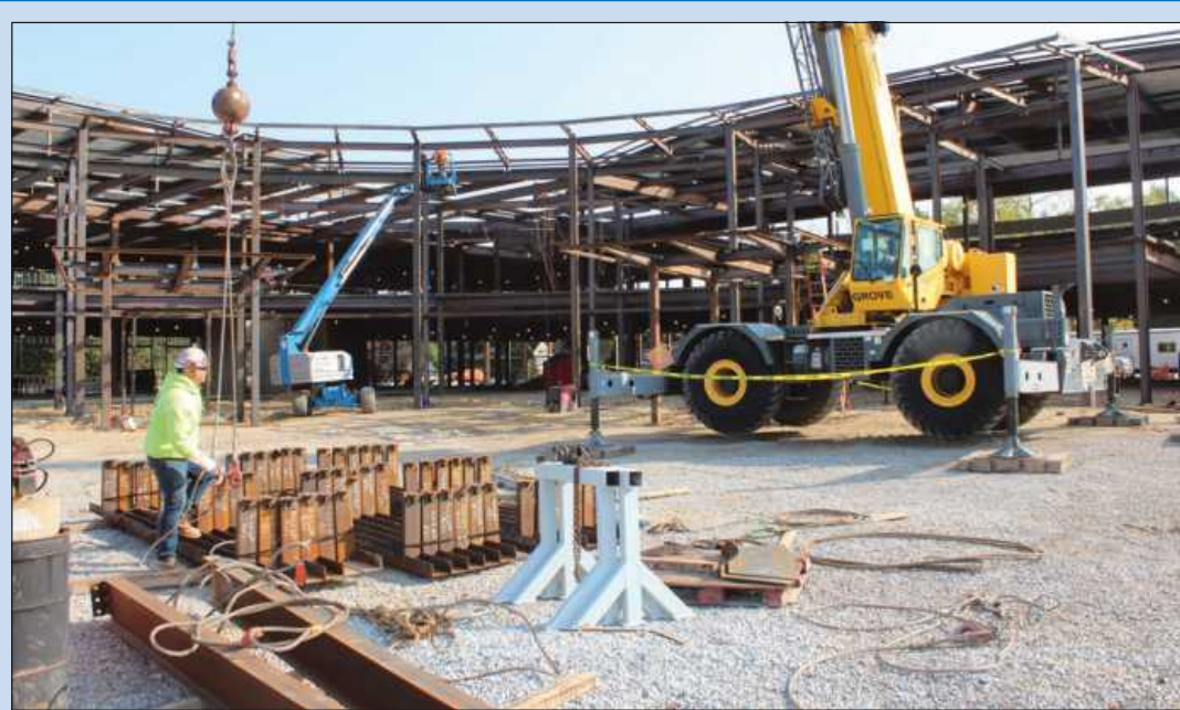
MOVING IRON at the Owosso Memorial Hospital project are Dave Nelson of Iron Workers Local 25, working with crane operator Dave Haggerty of Operating Engineers Local 324. They’re employed by Tri-Steel.
