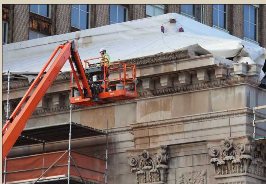
DENTIL MOLDING in the upper reaches of the Michigan Central Station's former Waiting Room gets the attention of a BAC Local 2 mason working for Ram Construction Services.
