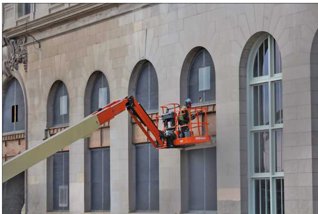
REHABILITATION OF WINDOW frames proceeds on the east side of Michigan Central Station. Ford is replacing all of the windows at the train station with historically accurate replicas – even though new, non-historically-accurate windows were installed just a few years ago by the previous owner.
