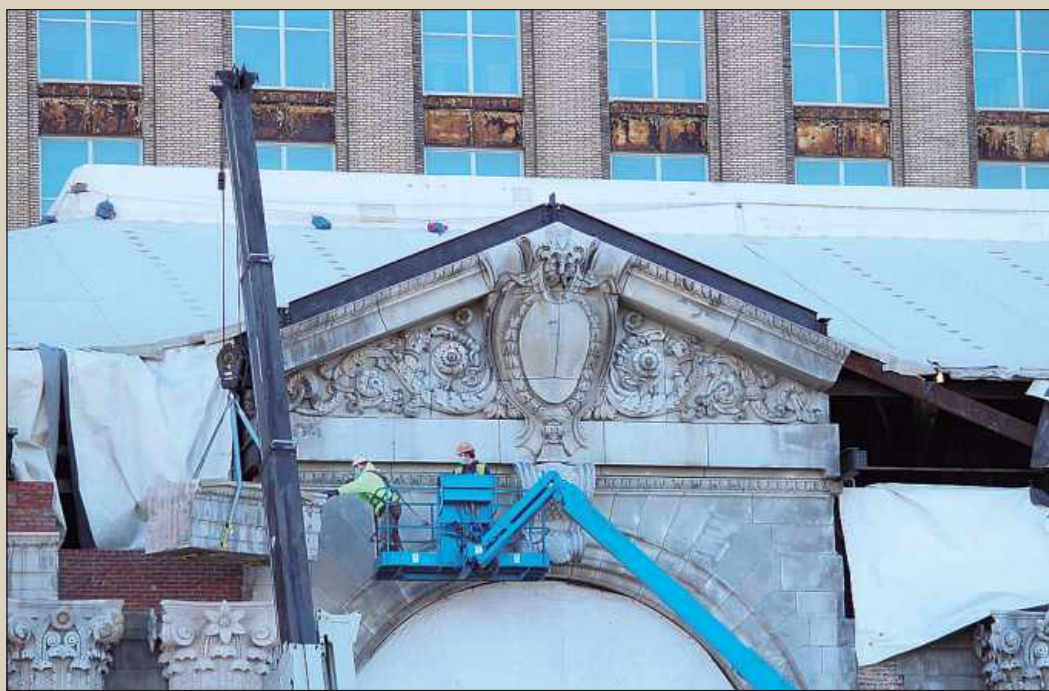
BRICKLAYERS AND ALLIED Craftworkers Local 2 members employed by Ram Construction Services set a replicated section of a capital piece atop a column in front of the Michigan Central Station. The replicated limestone section was manufactured by Capital Stoneworks.
