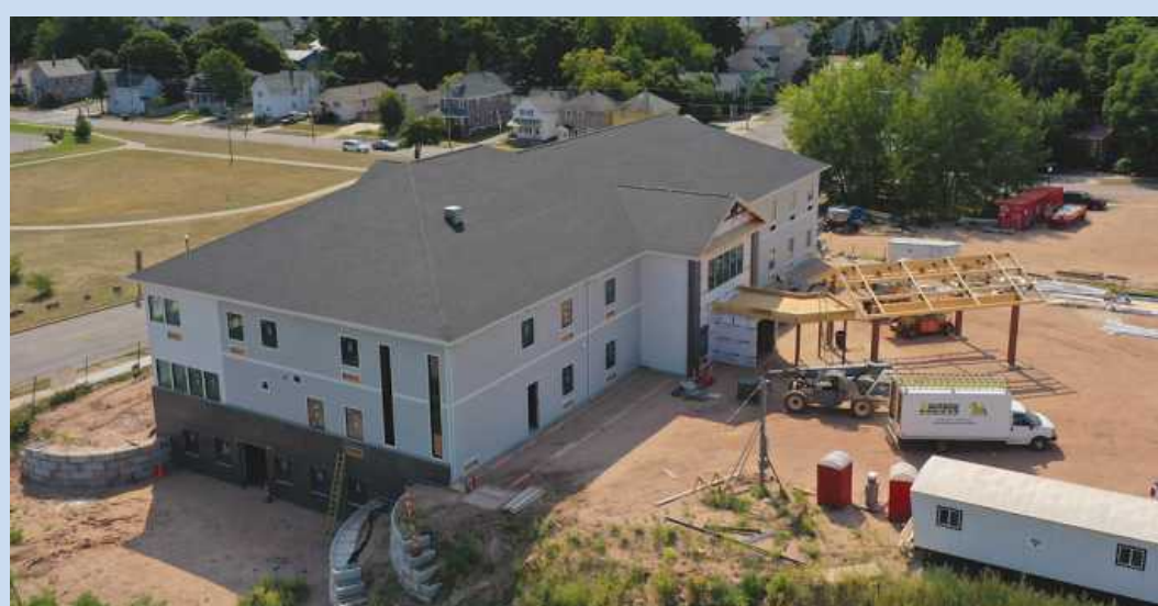
THE STEVE MARIUCCI Family Beacon House in Marquette, located next to the UP Health System-Marquette Hospital, will be a reasonable-cost option for patients' families visiting from afar. Closner Construction is managing the project, which is expected to wrap up next month.
