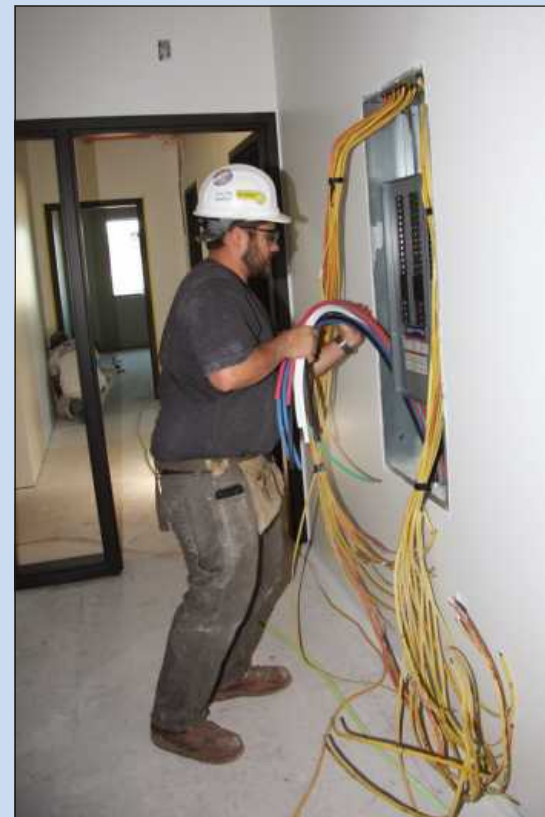
WRANGLING WIRE at the Beacon House project is Alex Jones of IBEW Local 906. He's employed by JP Electric Professionals. Photo by: Jack Deo
