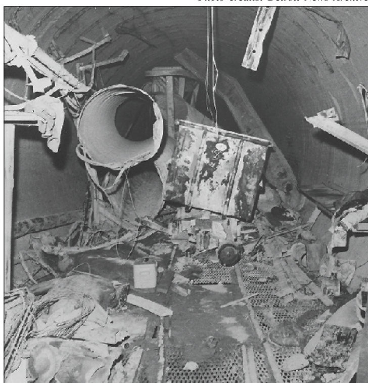
THE MANGLED MESS inside the Port Huron water tunnel after the explosion. The blast claimed 22 lives.
