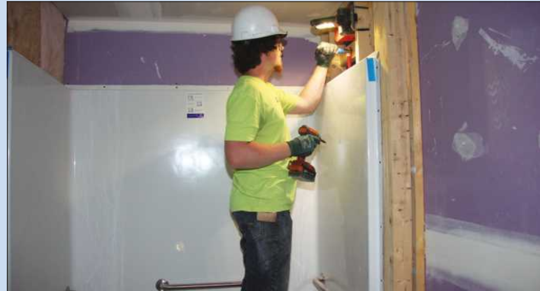
SETTING THE SHOWER plumbing in a guest room at the Beacon House is Austin Durand of Plumbers and Pipe Fitters Local 111. He's employed by Dressler Mechanical. Photo by: Jack Deo
