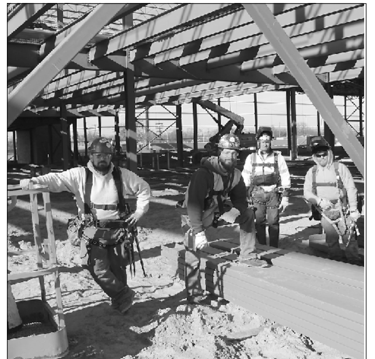
WAASKED Iron Workers Ryan Lorenzon, Tristan O'Day, Chris Bowman and Bob Jones to pause what they were doing for a group photo, while putting up the iron at the Michigan Regional Council of Carpenters and Millwrights building in Detroit. The Local 25 members are working for B & A Steel.
