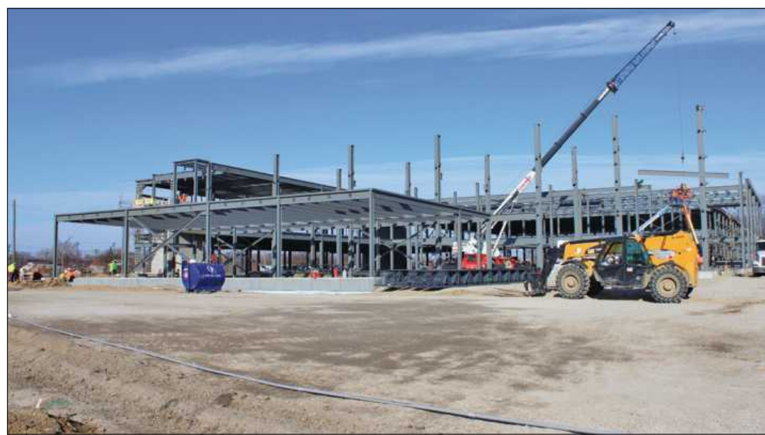
THE MICHIGAN Regional Council of Carpenters and Millwrights is undertaking construction of a new 144,000-square-foot training center and offices for union administration on Detroit's west side. It will consolidate the union's operations in Southeast Michigan.
