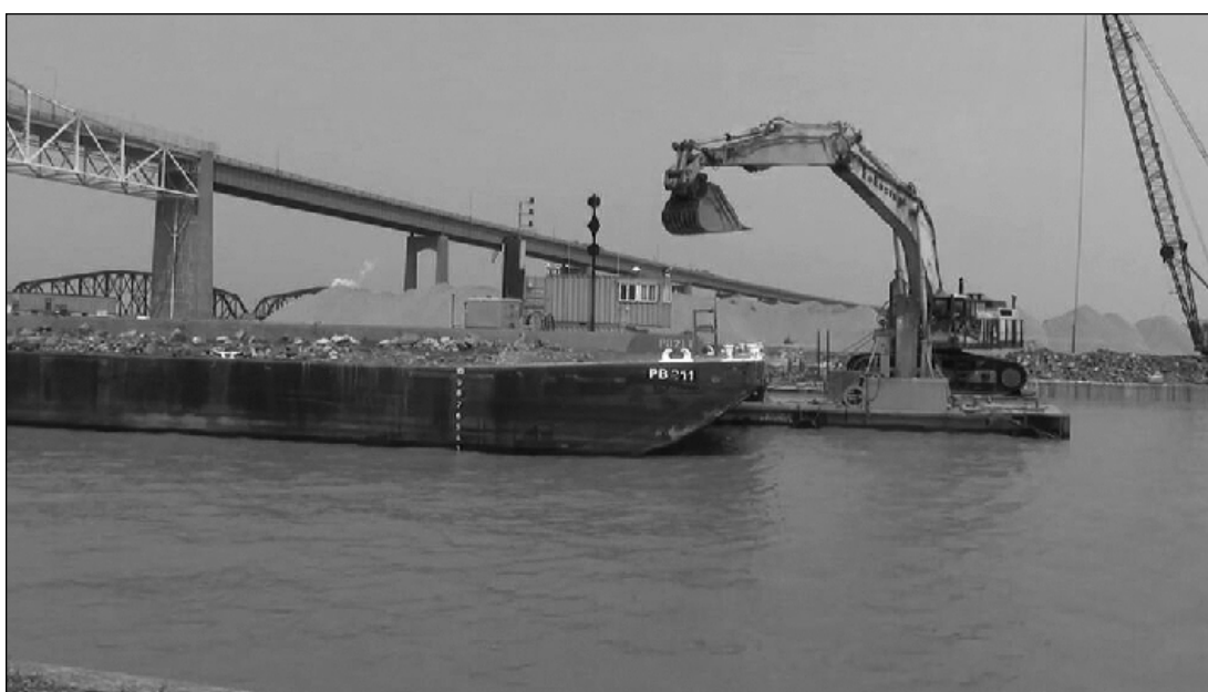
THE MULTI-YEAR expansion of the Soo Locks in Sault Ste. Marie, which will continue in the spring, is proceeding under a National Infrastructure Alliance agreement involving four unions. A key federal contract for the management of the future $1.5 billion construction of the new, twinned Poe Lock has yet to be signed, but is expected to be union-friendly under the new PLA rules. Photo credit: Up North Live
