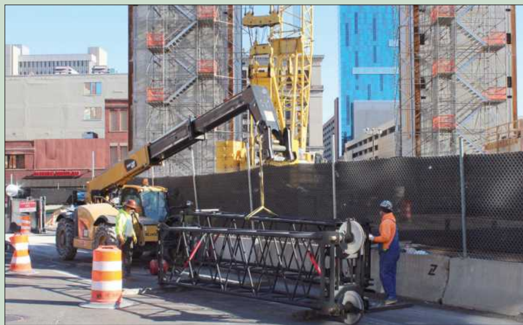
UNPACKING A 90-TON crane for use at the Exchange Building site in Detroit are Jason King and Jimmie Kerr of Operating Engineers Local 324. They're employed by Connelly Crane.
