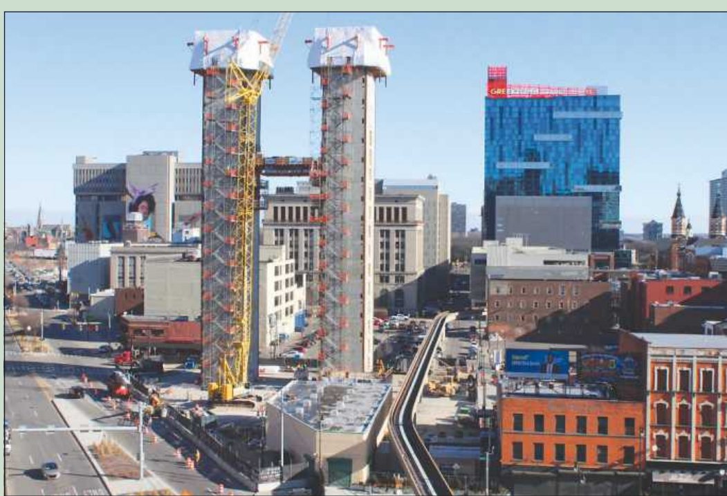
DUAL CONCRETE TOWERS will form the backbone of the new Exchange Building in Detroit. The tower's 16 floors will be built on the ground and then jacked into place, so the floors will be built from the top down.
