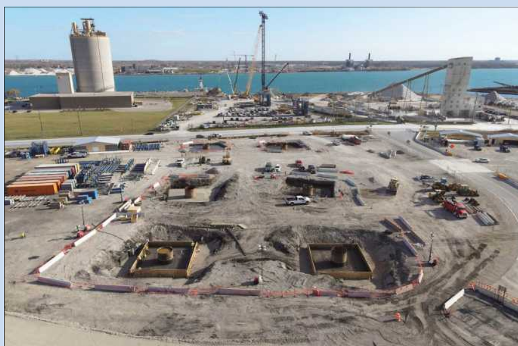
ANCHORAGE POINTS for the foundation that will support the tower on the Detroit side of the Gordie Howe International Bridge are placed along the Detroit River. The span will come ashore overhead at the Lafarge North America's riverfront aggregates plant, just north of Zug Island.
