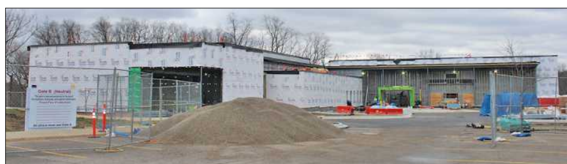
THE UNIVERSITY of Michigan's new Dance Building, shown under construction on the school's North Campus.
