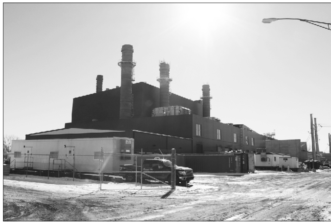
THE 250-MEGAWATT Delta Energy Park natural gas-fired power plant is going up on the grounds of the Lansing Board of Water and Light’s Erickson Station in Delta Twp.
