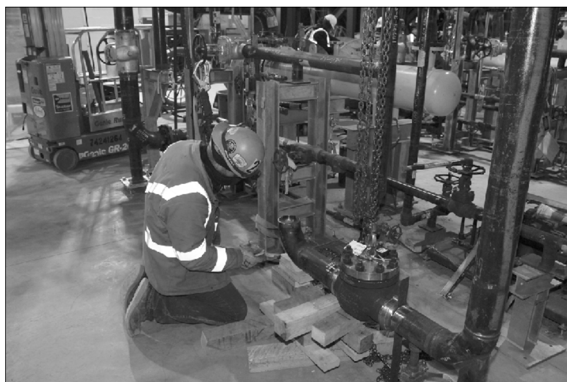
TAKING THE MEASURE of a pipe at the Delta Energy Park in Delta Township is Dave Hardaker of Plumbers and Pipefitters Local 190. He’s employed by Scheck Mechanical.
