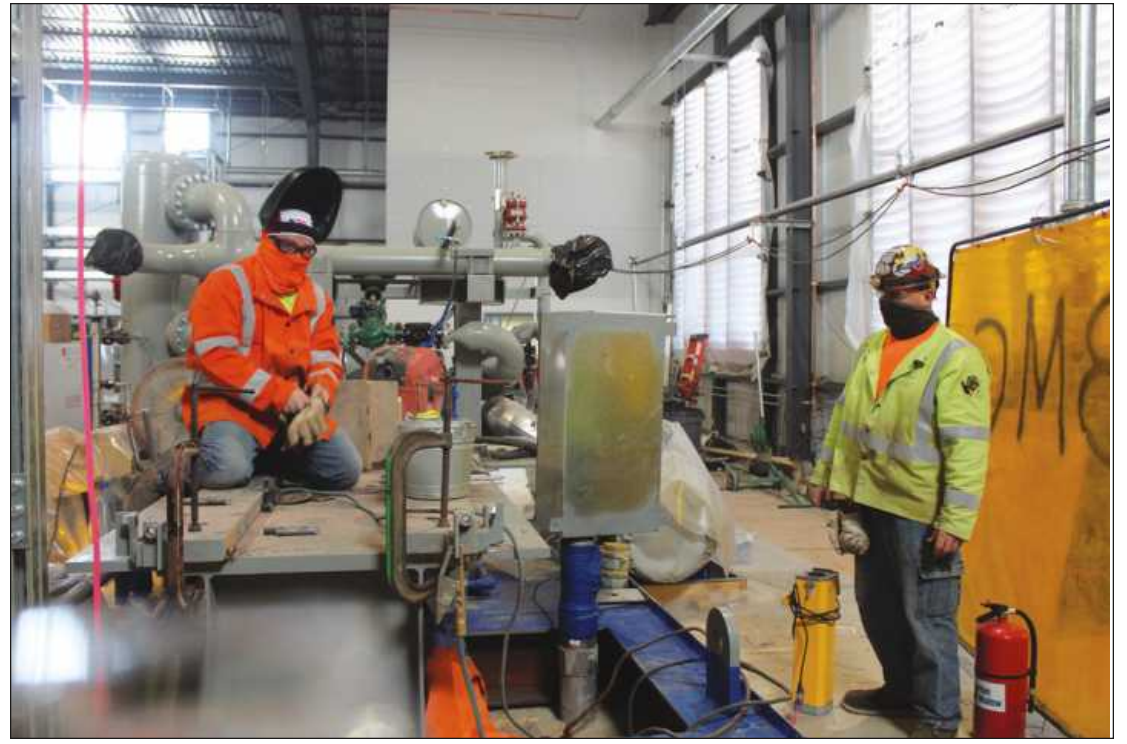
WORKING ON A PLATFORM for a compressor pump at the Lansing Board of Water and Light's new Delta Energy Park are Rick Kehoe of Iron Workers 25 and Matt Kern of Millwrights Local 1102. They're employed by Barton Malow.
