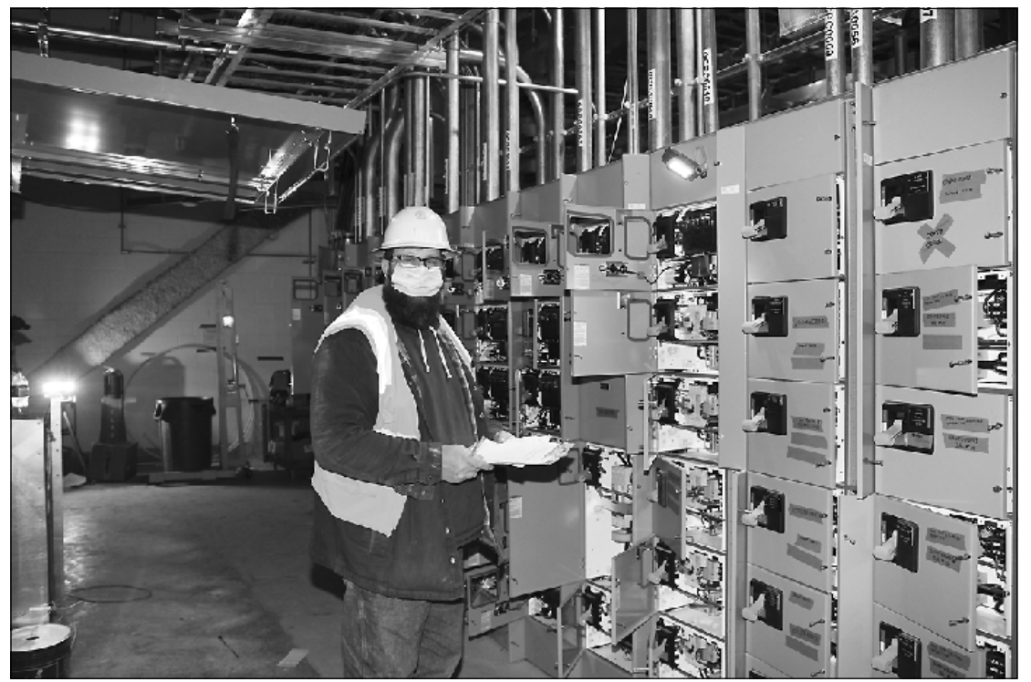
CHECKING OUT a 480-volt panel while working at the Lansing Board of Water and Light's Delta Energy Park power plant is Larry New of IBEW Local 58. He's employed by Utilities Instrumentation Service.
