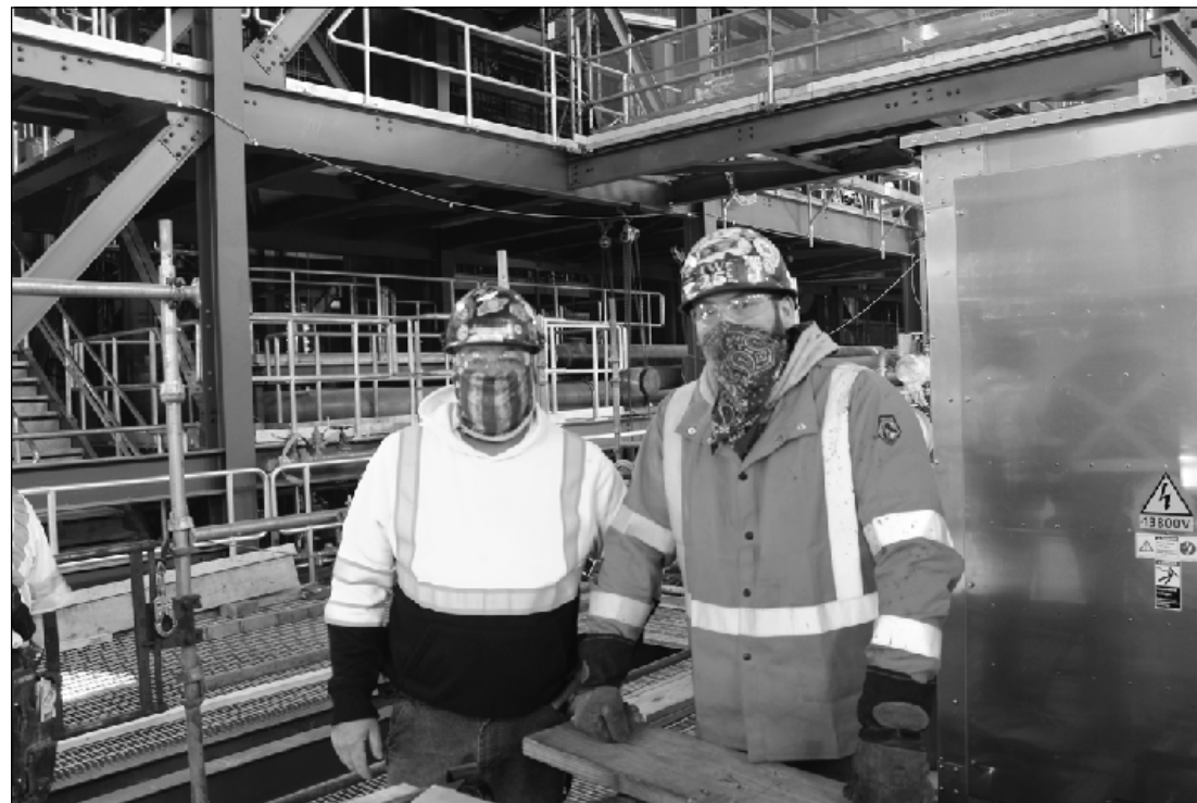
AT WORK AT THE Lansing Board of Water and Light’s Delta plant are Iron Workers Brad Coons and Tim Thomas of Local 25. They’re employed by Barton Malow.
