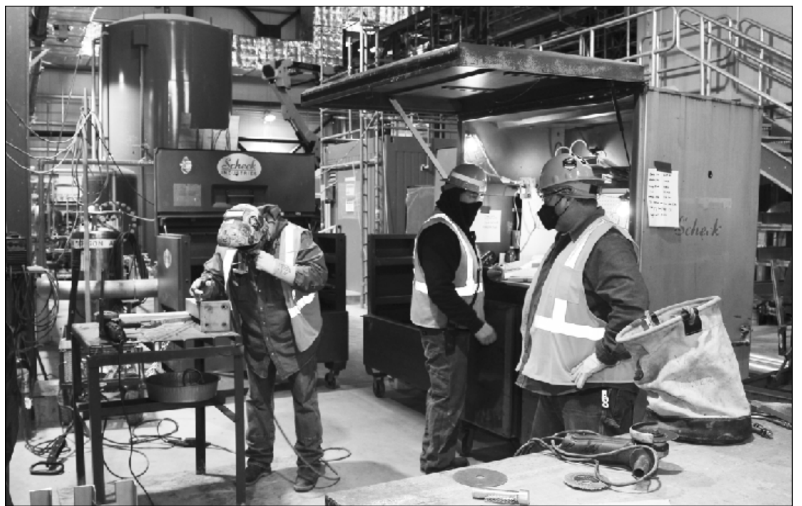
AT WORK BUILDING the new Lansing of Board of Water and Light Delta Energy Plant are pipe trades workers (l-r) Jason McDiarmid, John Ortiz (Plumbers and Pipe Fitters Local 174) and Mark Hutchinson (UA Local 118, Kenosha, Wis.). They're employed by Scheck Mechanical.
