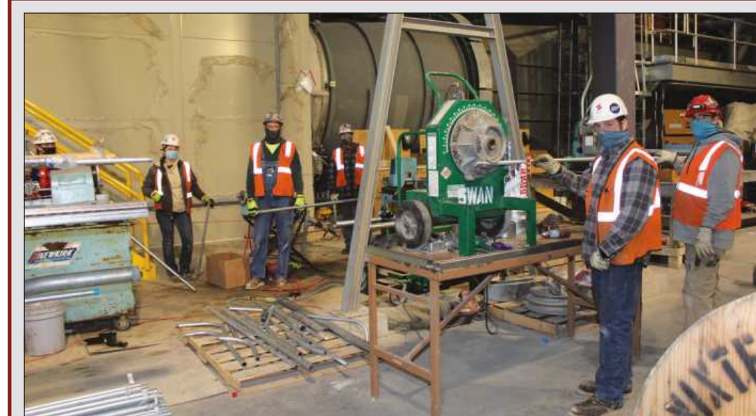
THIS GROUP OF ELECTRICIANS stopped what they were doing to have their picture taken at the Lansing Board of Water and Light's Delta Energy Park power plant. The IBEW members include (l-r) Vanessa North (Local 665); Hanna Harrington (Local 275); Howard Revard (Local 557); Barry Bock (Local 692); Scott Sovo (Local 557); William Alberts (Local 557) and Justin Kaczor (Local 557). Employed by Newkirk Electric and Swan Electric, the team was working on cutting and bending and conduit for the plant.
