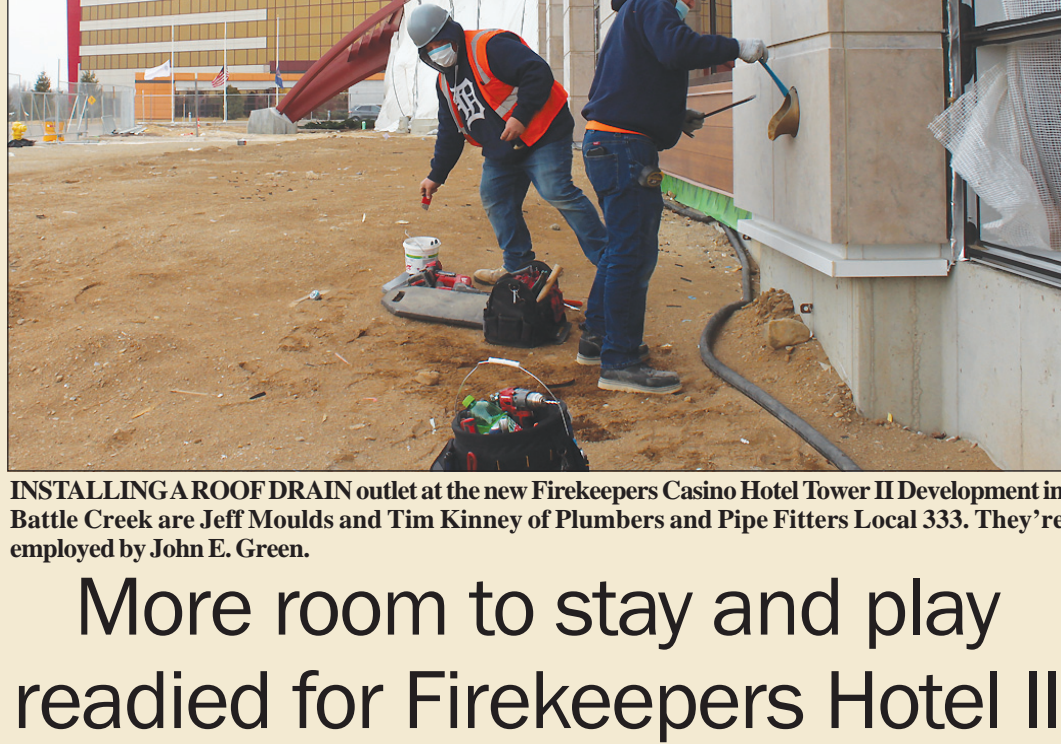
INSTALLING A ROOF DRAIN outlet at the new Firekeepers Casino Hotel Tower II Development in Battle Creek are Jeff Moulds and Tim Kinney of Plumbers and Pipe Fitters Local 333. They're employed by John E. Green.
