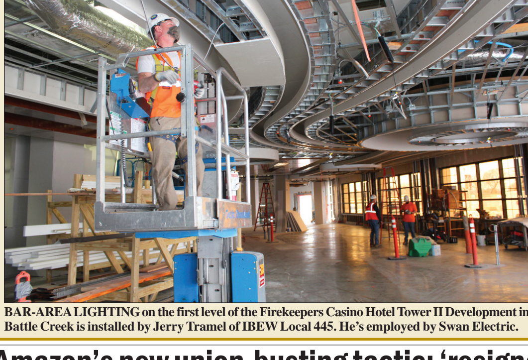
BAR-AREA LIGHTING on the first level of the Firekeepers Casino Hotel Tower II Development in Battle Creek is installed by Jerry Tramel of IBEW Local 445. He's employed by Swan Electric.
