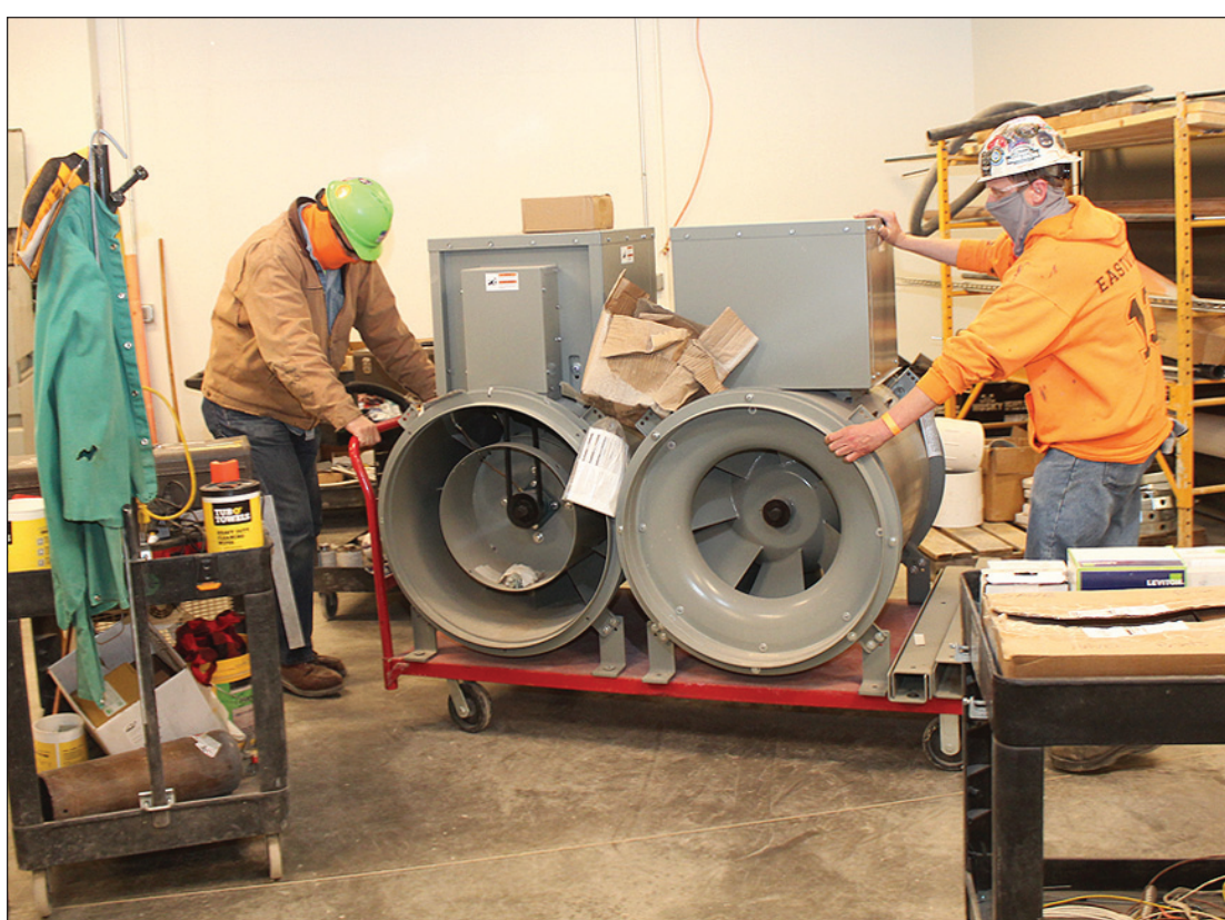
ON A ROLL MOVING HVAC barrels for CO2 exhaust at the Firekeepers Hotel II project in Battle Creek are (l-r) foreman Scott Hebron and Brett Abbruzzese of Sheet Metal Workers Local 7. They're employed by Applegate.
