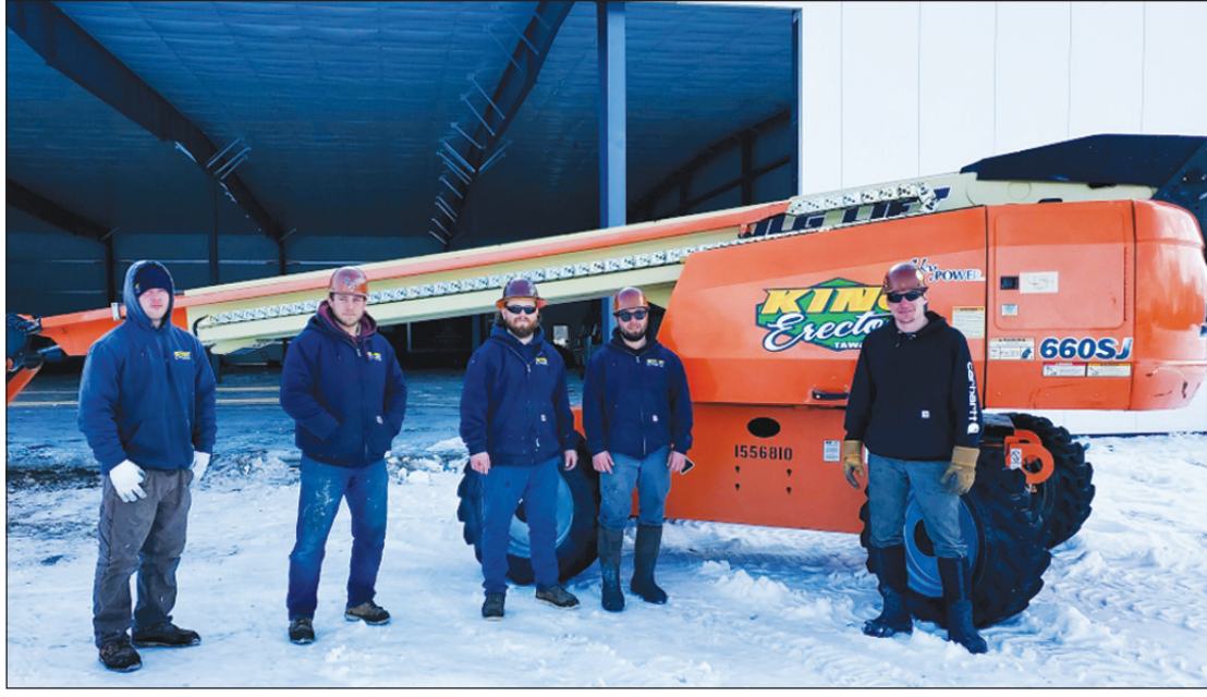
CONSTRUCTION OF A MARIJUANA growing facility in Jackson is sprouting nicely, thanks in part to a crew of Iron Workers Local 25 members employed by King Erectors. The Local 25 crew shown here (l-r) include Matt Reid, Jeremy Ross, Noah Woodruff, Lenny LaLiberty and Devin Polak. Local 25 Business Rep. Marc Crance notes that they never missed an hour on the job all winter erecting pre-engineering buildings at the site. Florida-based Objectiv Growth is building a 71,500 square-foot marijuana and growth facility at the site, a $19 million in capital investment.
