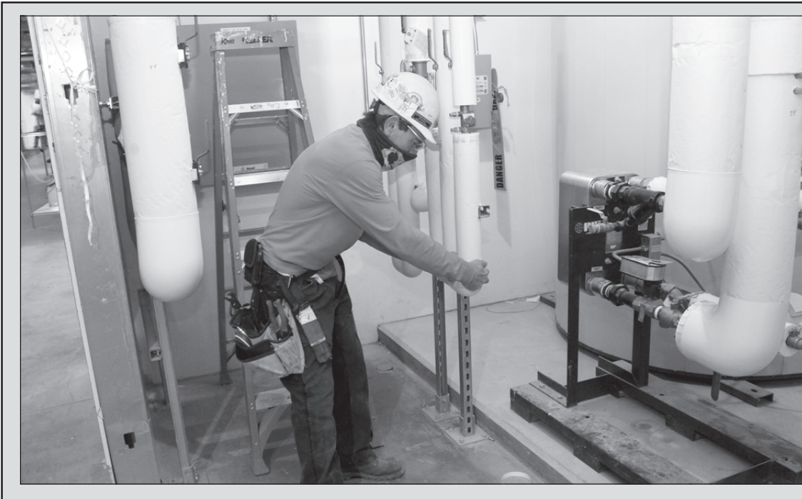
PLACING A NEAT PVC jacket around piping at the Firekeepers Casino Hotel Tower II Development in Battle Creek is Josh Bower of Heat and Frost Insulators Local 47. He's employed by 3MI.
