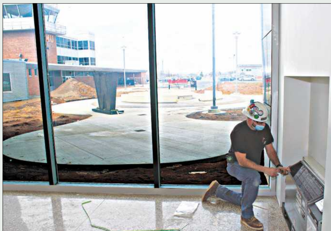
MALL CITY MECHANICAL foreman Matt Hatfield of Plumbers and Pipe Fitters Local 333 works on a cabinet heater unit near the main entrance of the new terminal building at Battle Creek's Kellogg Airport.
