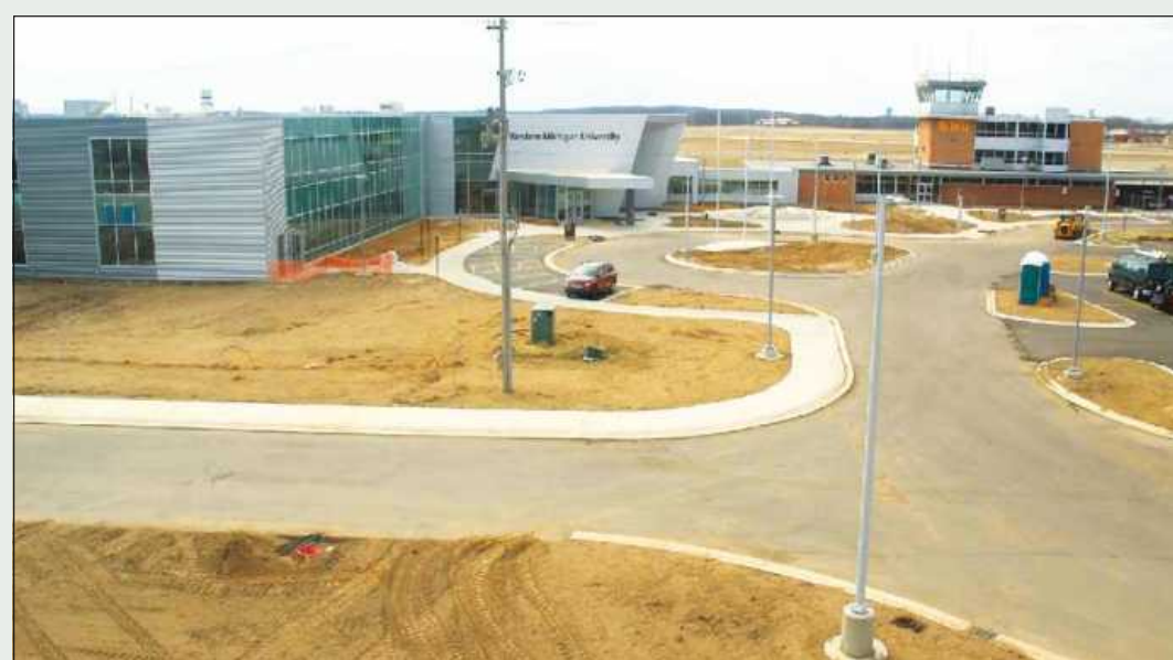
WESTERN MICHIGAN UNIVERSITY's Aviation School is renovating and expanding their facilities at Battle Creek's Kellogg Airport. The existing brick building and control tower, at right, are being supplemented by new facilities, at left, that will allow the program to enhance and expand its educational offerings.
