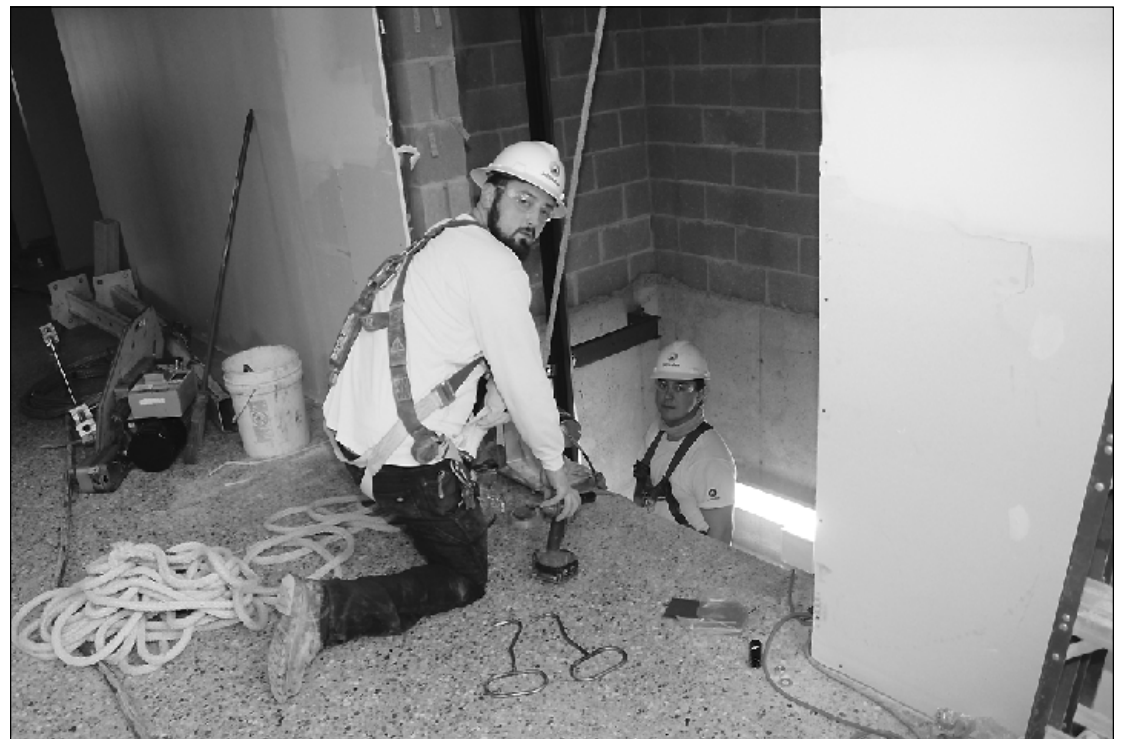
AT WORK AT Battle Creek's Kellogg Airport are (l-r) Local 85 elevator constructors Devin Richmond and Andrew Pawlowski. They're employed by Schindler Elevator.
