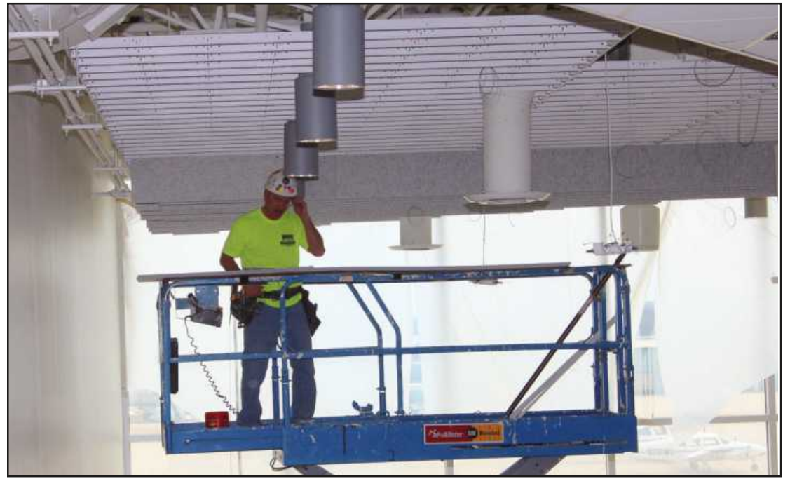
INSTALLING SOLID BAFFLES in the addition to the Battle Creek Kellogg Airport is Rod Eberhard of Carpenters Local 525. He's employed by Cooke Jackson.
