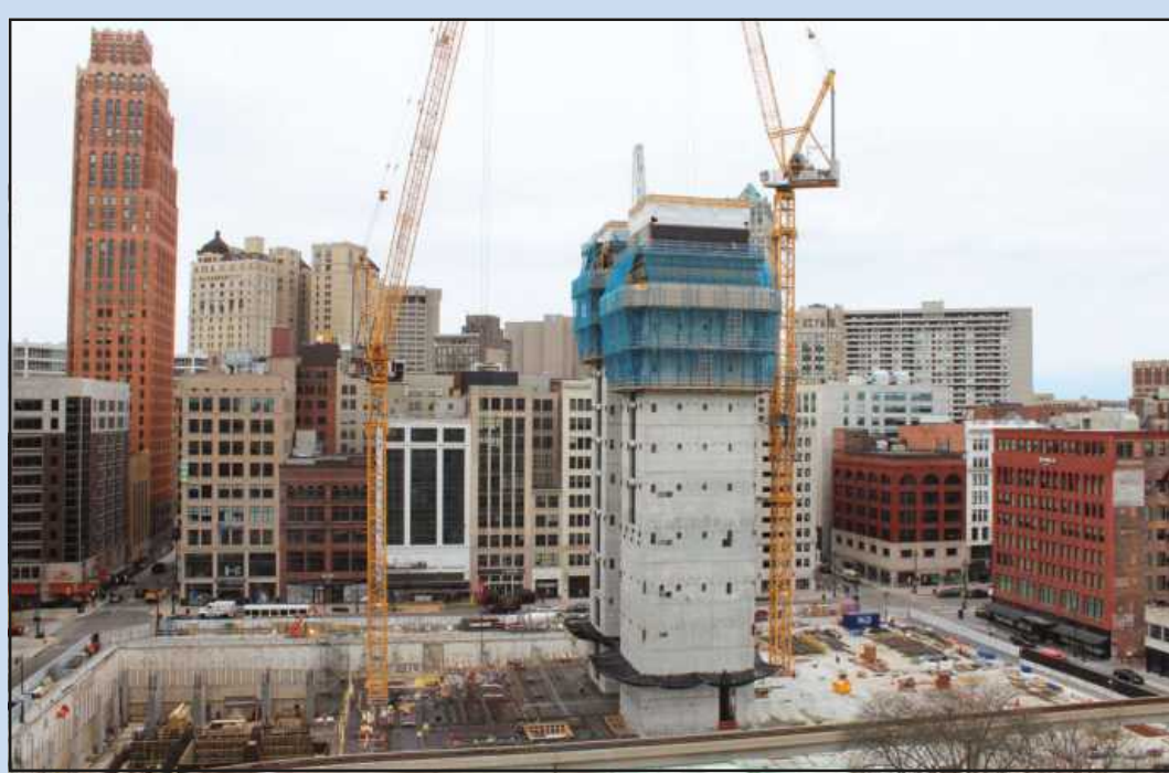
THE BLOCK-LONG, former site of the Hudson's department store in Detroit is being redeveloped into a plot of land that will host the state's second-tallest building. The $909 million Bedrock-Detroit development will start seeing steel erection this summer, but is currently distinguished by a rising pair of concrete towers that will contain elevators.
