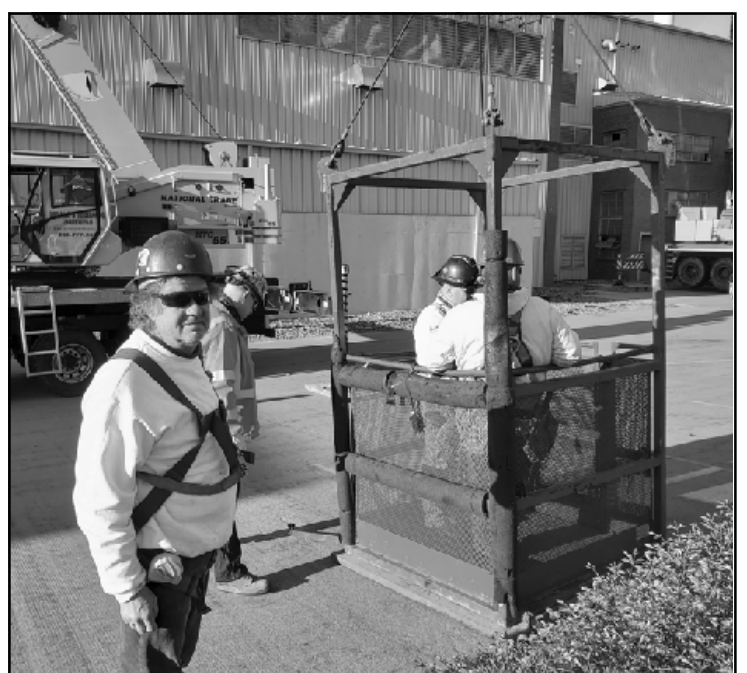
CHECKING RIGGING ON the man-basket at the Knauf project are Local 25 iron workers Greg Hartford, Gino Burk, Craig Pettel, and Rich Carter. They're employed by Schweitzer Co., Battle Creek.
