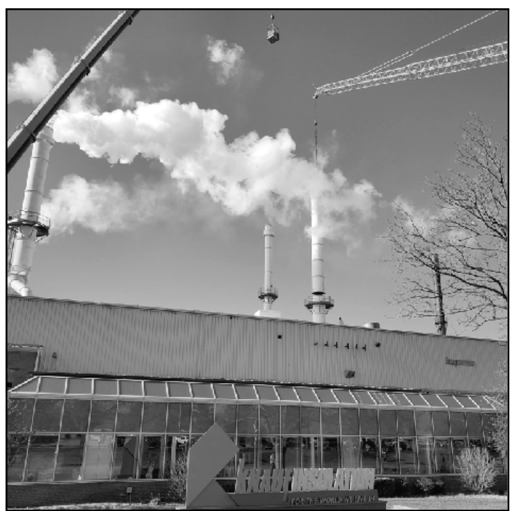
THE EXISTING STACK is separated during the renovation at the Knopf-Albion plant. Photos by Marc Crance
