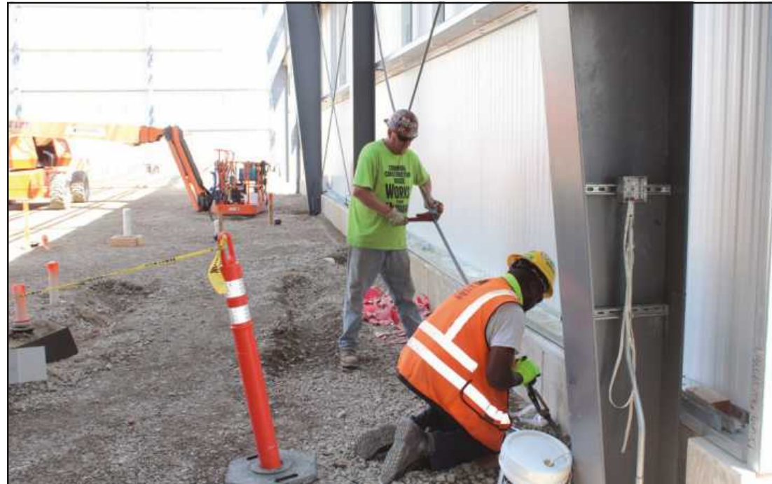
TENSIONING CABLES on a wall at the Dakkota-Kettering project in Detroit are iron workers David Urchick and Stephen Gavin. They're employed by Midwest Steel.
