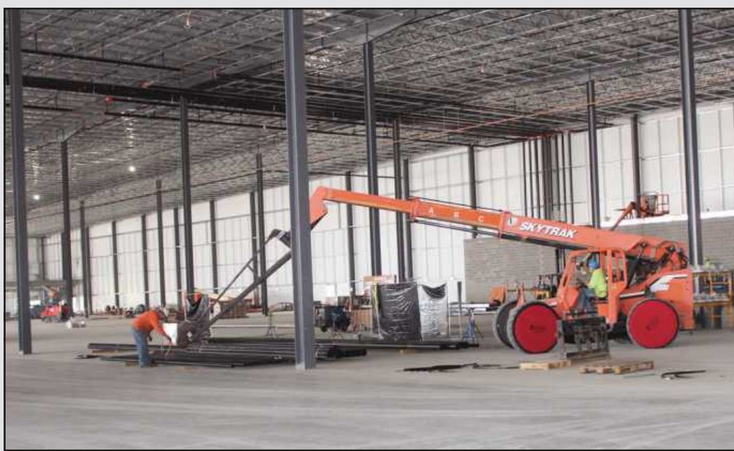
TEAMING UP TO MOVE a bundle of three-inch gas pipe at the Dakkota-Kettering project are Paul Wisniewski of Plumbers 98 (employed by Guideline) and Jacob Fraley of Operating Engineers Local 324.
