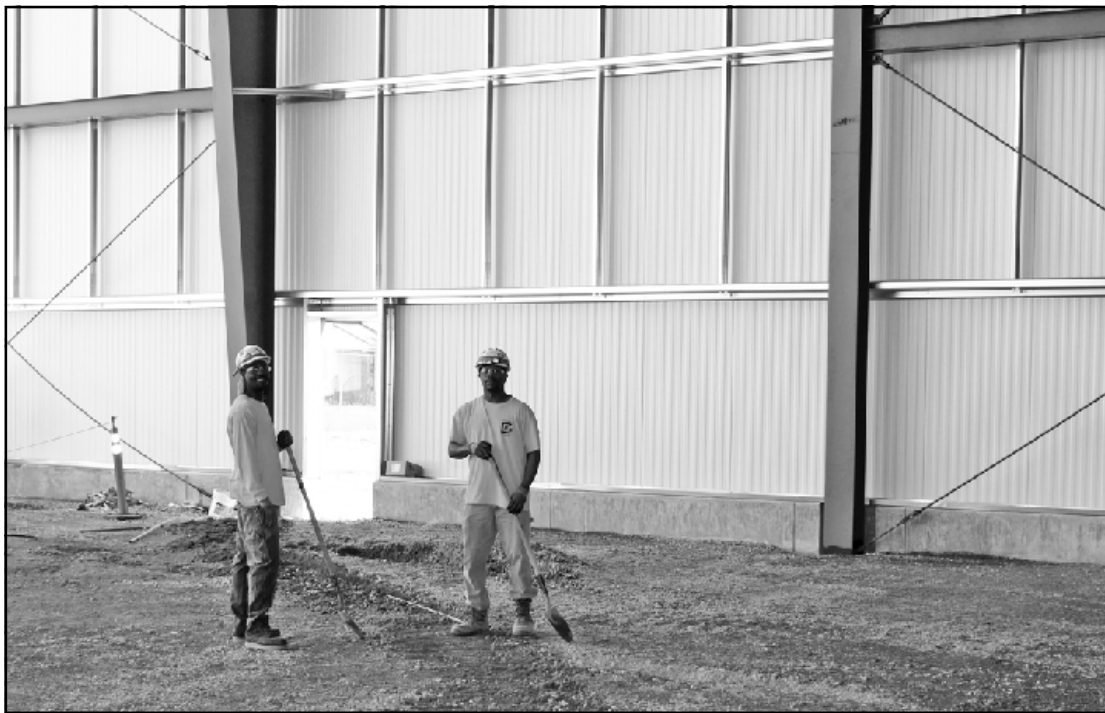
BURYING CONDUIT they placed in the unfinished floor of the Dakkota-Kettering project in Detroit are Derand Favors and Leonard Robinson of IBEW Local 58. They're employed by Triangle Electric.
