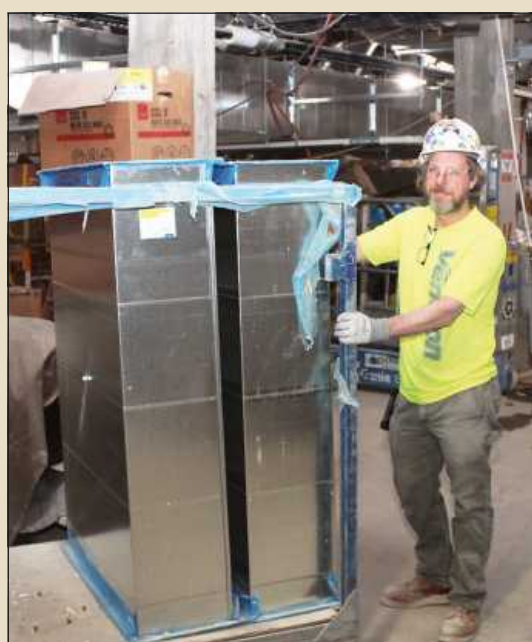
SECTIONS OF DUCT get a ride on the basement level of the train station, from Kevin McDonald of Sheetmetal Workers Local 80. He's employed by Ventcon.
