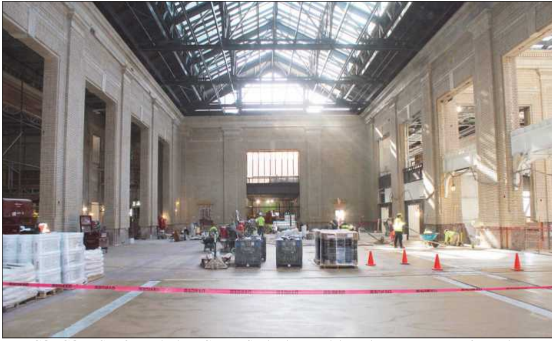
THE CONCOURSE of the Michigan Central Station in Detroit is getting a new terrazzo floor, with work done by Bricklayers and Allied Craftworkers Local 2 masons employed by Michielutti Brothers Inc.
