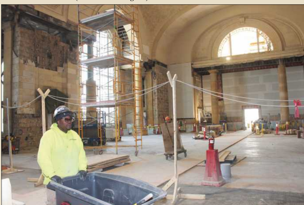
MOVING REFUSE materials through the former main waiting room at the Michigan Central Station project is laborer Sammy Peaster of Local 1191. He's employed by Brinker.
