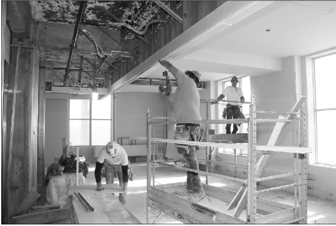
AT WORK ON THE THIRD FLOOR of the Michigan Central Station project in Detroit are Carpenters Jairo Pina, Jaime Perez and David Sanchez. The Michigan Regional Carpenters Council Local 687 members are employed by Dencco.
