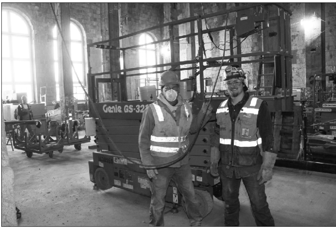
DOWN FROM THEIR LIFT , pipe fitters Pete Ivory and Justin Goretzki stopped for a photo in late April while working in what was originally a restaurant at the Michigan Central Station project in Detroit. The Local 636 members are employed by John E. Green.
