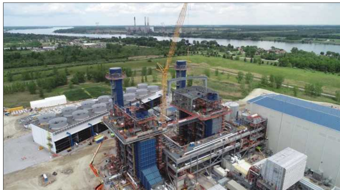
DTE ENERGY'S Blue Water Energy Center is shown under construction on the grounds of the utility's Belle River plant in East China Twp. Photo credit: Commercial Contracting Corp.
