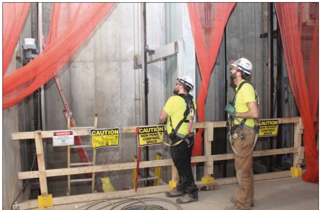
AWAITING THE DROP of a cable in an elevator shaft at the Michigan Central Station project in Detroit are Jason Dembeck and Chris Grider of Elevator Constructors Local 36. They're employed by Kone.
