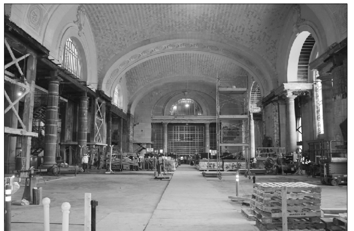
THE FORMER WAITING ROOM of the Michigan Central Station is shown under renovation, part of a project that's seeing the entire 18-story building in Detroit being restored. The project is led by construction manager Christman Brinker.
