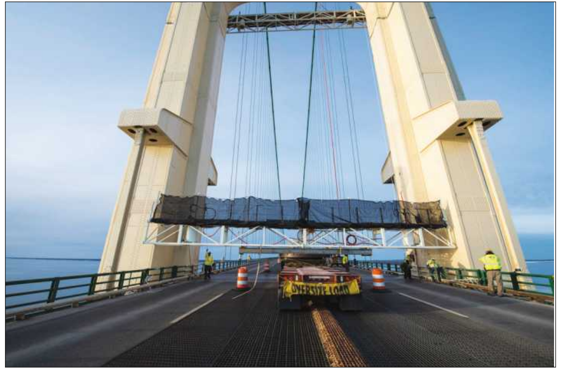
CONVENTIONAL SCAFFOLDING was used by Seaway Painting workers to paint lower parts of the 552-foot-tall Mackinac Bridge towers.
