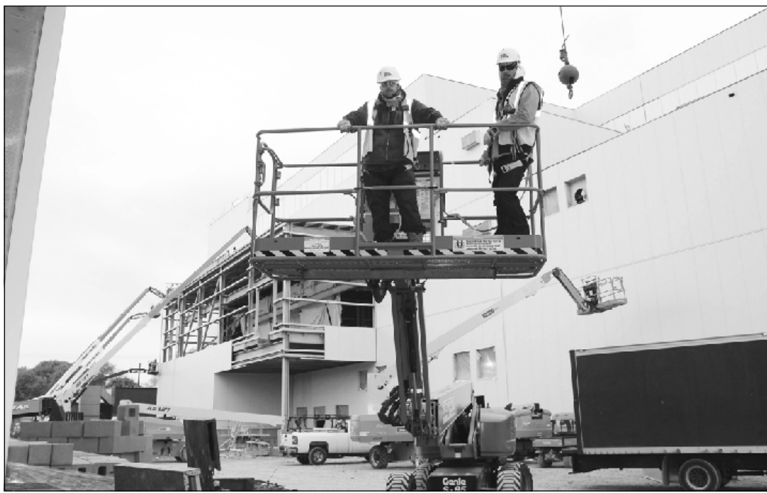
GETTING A LIFT outside the new Graphics Packaging boiler house in Kalamazoo are (l-r) Hunter Challender (UA Local 551, southern Illinois) and Hunter Challender (Plumbers and Pipe Fitters Local 333). They're employed by Andy J. Egan. They're helping to build a $600 million coated recycled board mill for Graphics Packaging.
