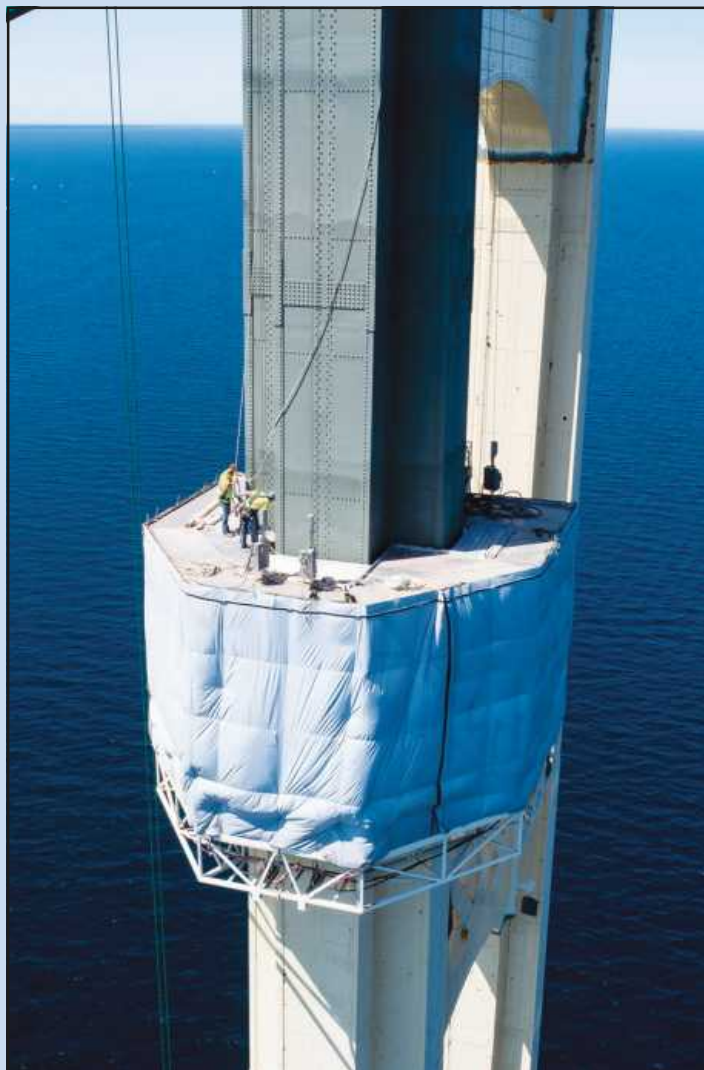
THE SCAFFOLD SYSTEM was designed to closely hug the 552-foot-tall Mackinac Bridge bridge towers, even as the towers taper as they rise. The enclosed 24-foot-tall scaffold helped allow the safe collection of old paint that was blasted off the towers. Cables suspended from new outriggers at the top of the towers allow the movement of the platform.
