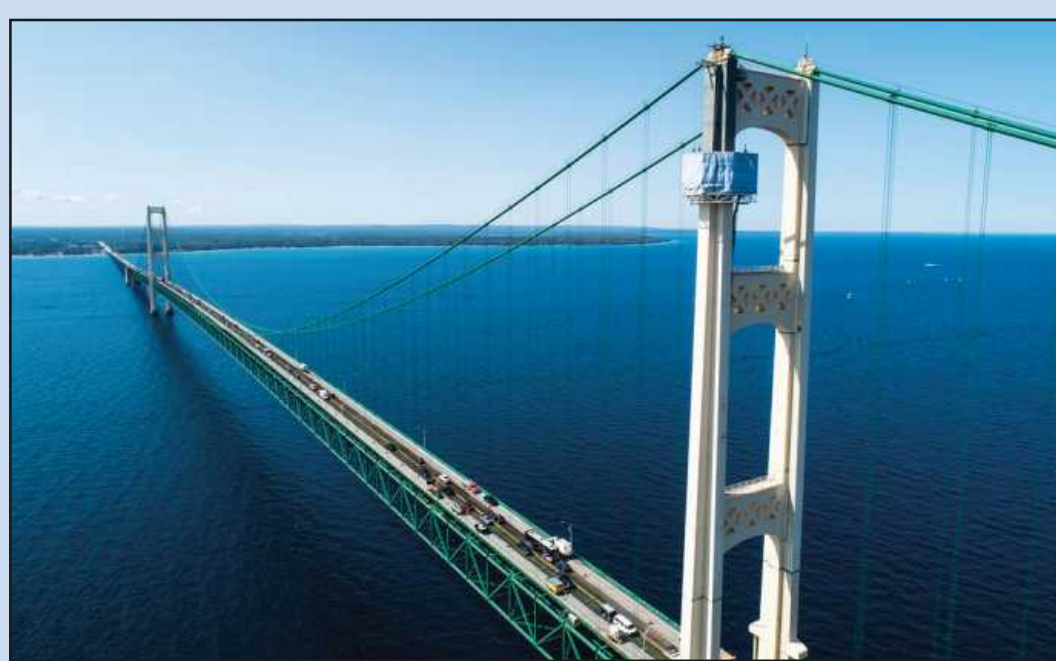
THE ONE-OF-A-KIND SCAFFOLDING used to support Seaway Painting painters on the Mackinac Bridge’s North and South towers over the past few years has been removed as the project nears completion. The platform not only allowed painters a safe and efficient base and enclosure to do their work, it was an engineering award-winner.
