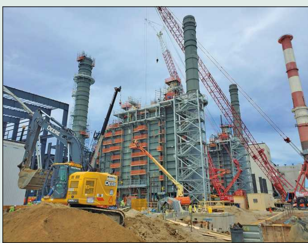
UNDER CONSTRUCTION on the grounds of the Erickson Power Station in Delta Twp. is the new Delta Energy Park, a natural gas-burning, 250-MW combined-cycle power plant. The project is managed by the team of Barton Malow and Clark Construction. At right is the signature red and white striped stack of the coal-burning Erickson plant, slated to be retired in 2025. Photo credits: Marc Crance
