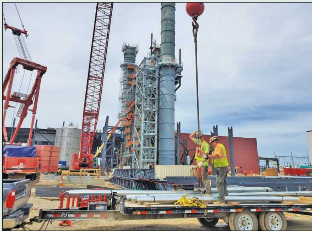
UNLOADING MATERIAL from a trailer at the Lansing Board of Water and Light's Delta Energy Park project are Pat Nichols and Josh Redinger of Iron Workers Local 25. They're employed by Redinger Steel.
