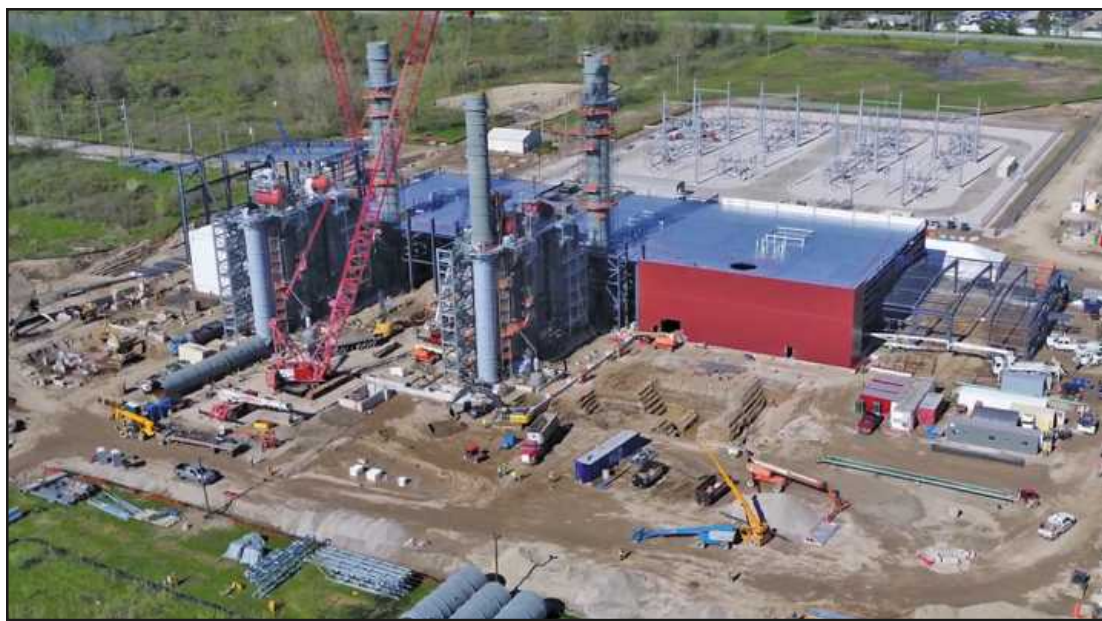
AN AERIAL VIEW from last month of Lansing Board of Water and Light's 250 megawatt Delta Energy Park in Delta Twp.
