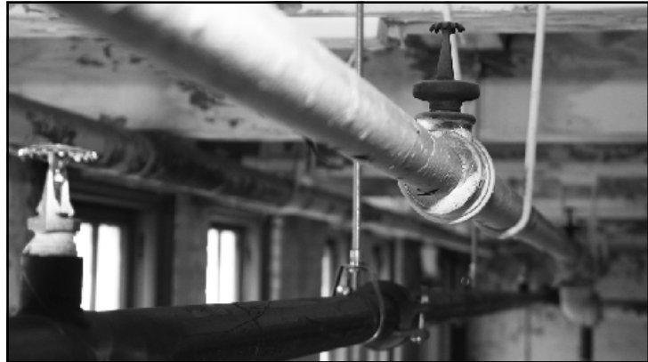
LOCAL 704 Sprinkler Fitters replaced the old sprinkler system at the Piquette Plant, at right, with new pipes and heads, at left. The old system was kept in place for display purposes.
