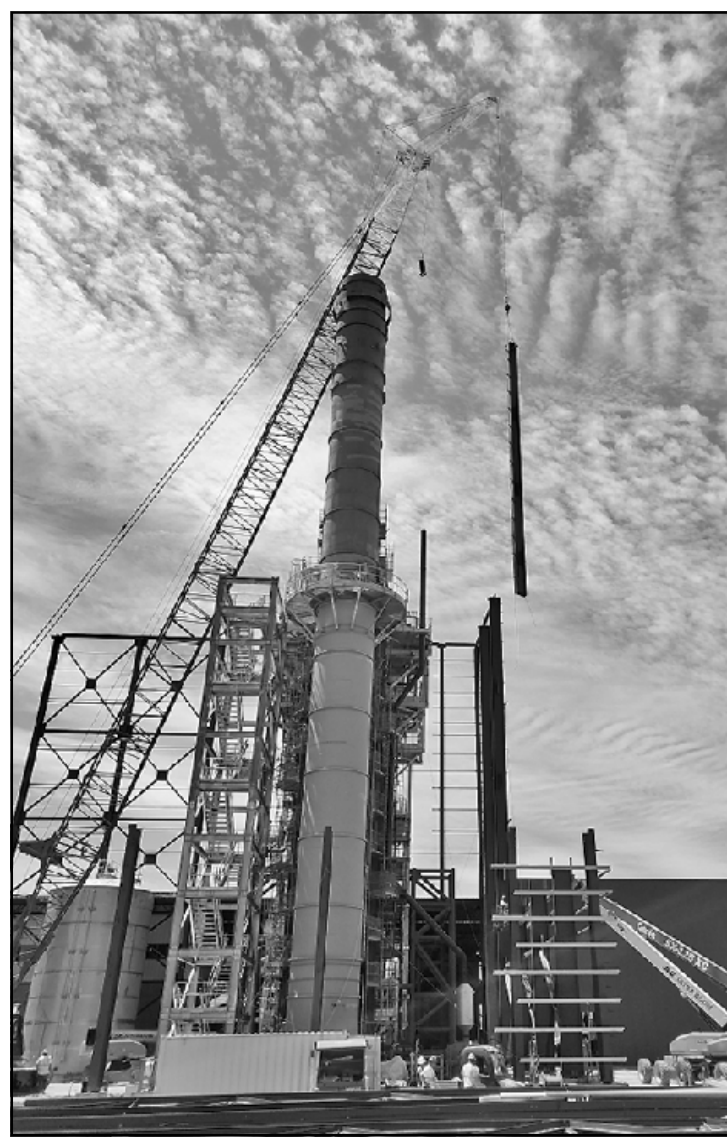
IRON WORKERS from Local 25 and Redinger Steel set iron at the Delta Energy Center project for the Lansing Board of Water and Light. Photo credit: Marc Crance
