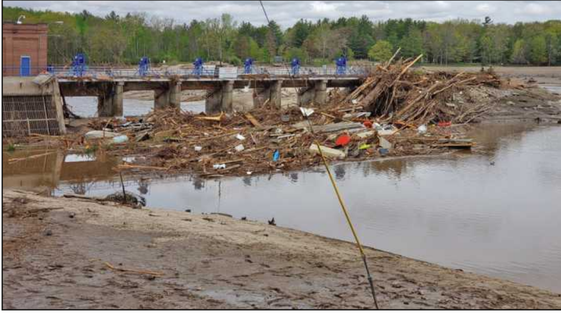
THE AFTERMATH OF the collapse of the Sanford Dam. Photo credit: Michigan Laborers
