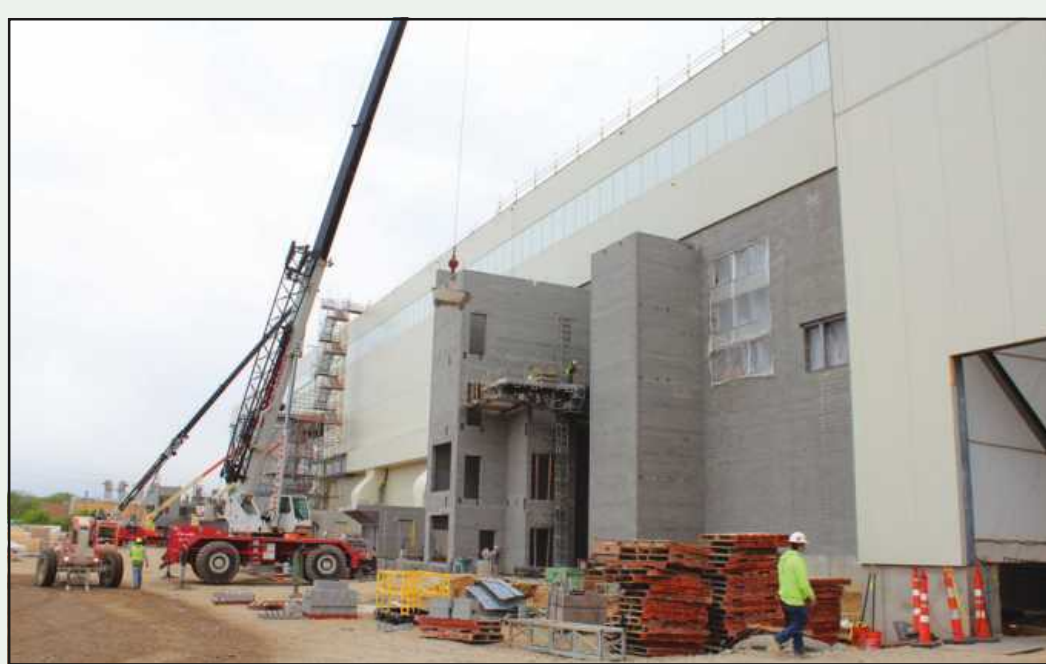
GRAPHICS PACKAGING in Kalamazoo and its building trades workforce is erecting a $600 million coated recycled board mill that will make the facility the largest producer of recycled paperboard in North America. The company makes folding cartons for food and beverage companies.
