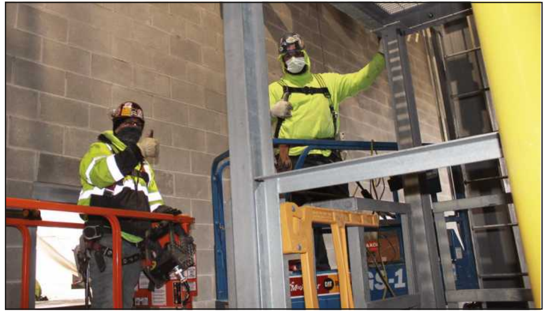
SETTING A PIPE RACK in the boiler building addition at the Graphics Packaging project in Kalamazoo are Alvin Vandergriff and Liam Knapp of Iron Workers Local 25. They’re employed by Barton Malow.
