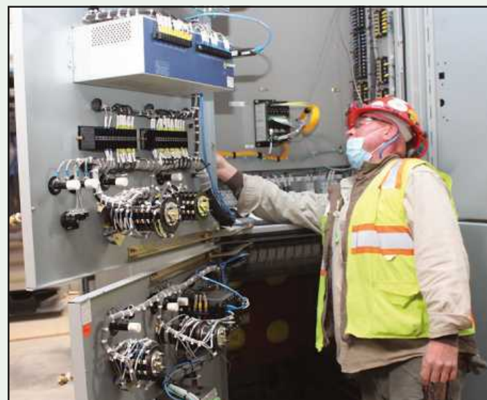
AT WORK SETTING UP 15,000-volt switchgear at the Graphics Packaging plant in Kalamazoo is Randy Williams of IBEW Local 131. The project steward is employed by Van Ert Electric Co./KEI Electrical Construction and Maintenance.
