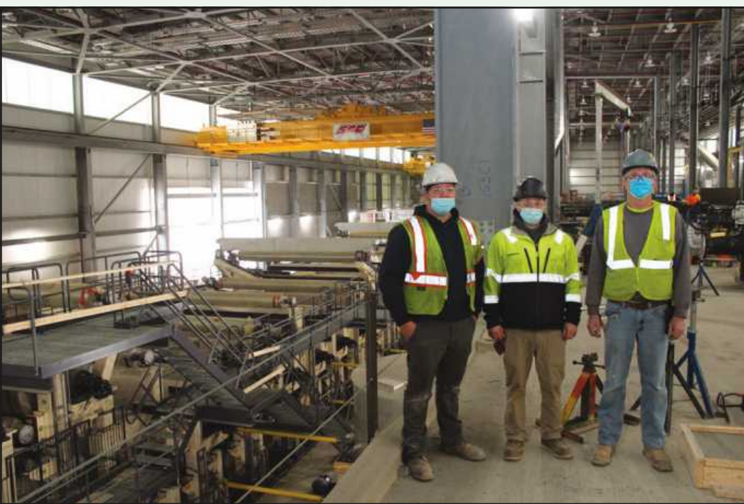
WE ASKED THIS GROUP of Plumbers and Pipe Fitters Local 357 members coming off their break to stand next to the massive new K2 Coated Recycled Board (CRB) machine at left, being installed at the Graphics Packaging plant in Kalamazoo. They are (l-r) Jarrett Nieboer, Alan Freund and foreman Greg VandeMaale. They are employed by R.W. Lapine.
