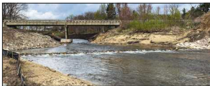
SITE OF THE FORMER Pucker Street Dam shown in April. A naturalized river rapids will be constructed at this location in late May-June. MDNR photo
