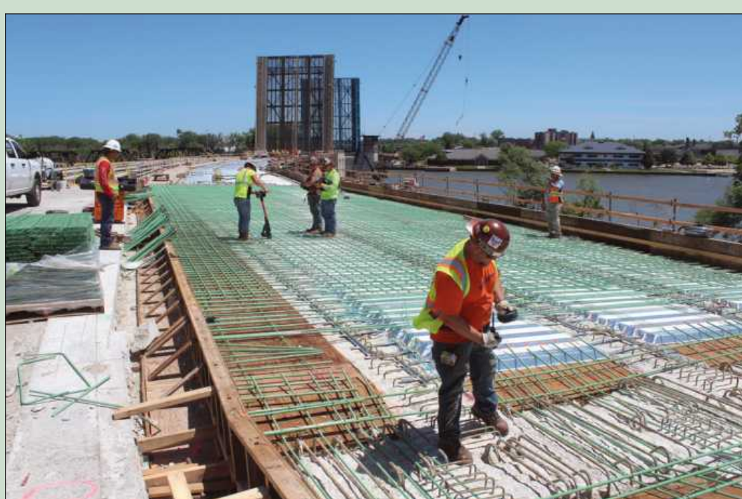
ON THE FIRST DAY (June 16) of reinforcing rod installation at the Liberty Bridge rehabilitation project in Bay City, Iron Workers Local 25 rodbuster Matt Walker unspools some wire. He's employed by Flatrock Bridge Group. Field Supt. Ben Meyer reports that the rodbuster crew will install about 2 million pounds of the green re-bar on both sides of the bridge.
