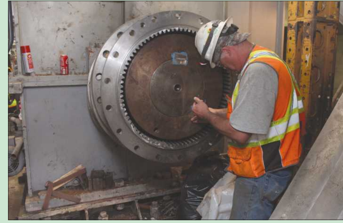
APPLYING SILICONE to a pinion gear that drives a leaf at the Liberty Bridge rehabilitation project in Bay City is Chad Atwell of Millwrights 1102. He's employed by Granite Kraemer North America.
