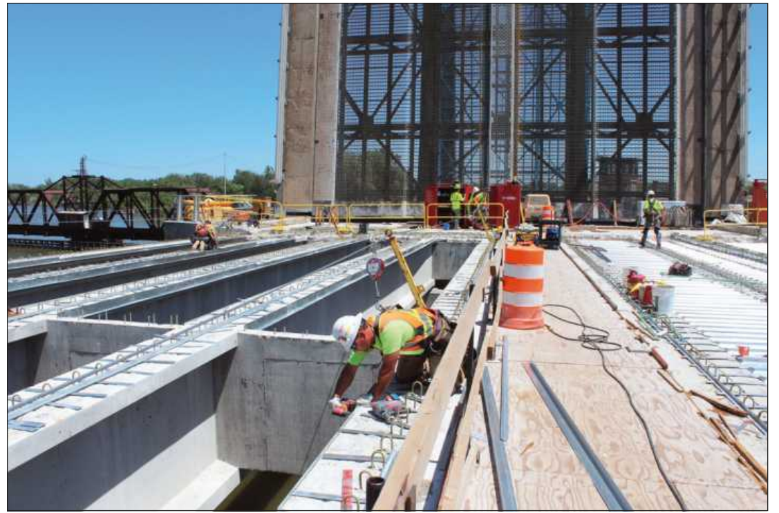
SETTING RAILS TO SUPPORT PANS in preparation for concrete placement is Carpenter Nick Revord of Michigan Regional Council of Carpenters and Millwrights Local 706. He's employed by Granite Kraemer Joint Venture.
