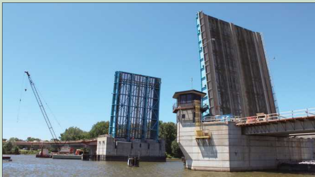
A WHOLESALE RENOVATION of the Liberty Bridge in Bay City over the Saginaw River is ongoing. About 100 tradespeople are working at the bascule drawbridge this summer, working with the Bay City Bridge Partners, Granite Kraemer Joint Venture, and several subcontractors.
