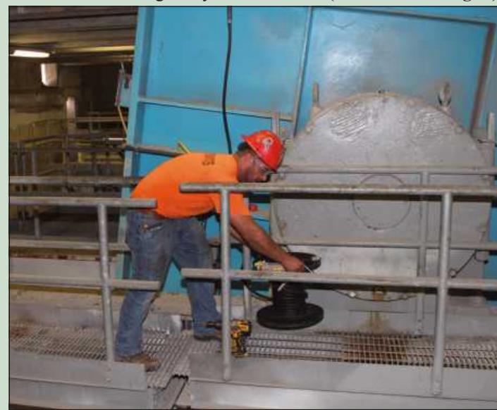
UNSPooling WIRE for a junction box in front of the west counterweight under the deck of the Liberty Bridge is Chris Gangler of IBEW Local 692. He's employed by Clements Electric.
