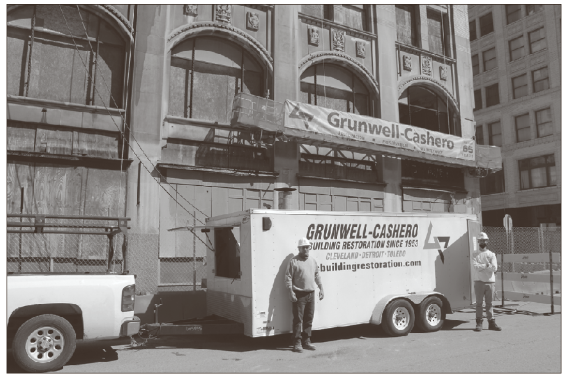
PAUSING FOR A PHOTO in front of the Park Avenue Building in Detroit that's under renovation are Project Supt. Jeff Cusin and mason Bob Pugno Jr. Both are Bricklayers and Allied Craftworkers Local 2 members employed by Grunwell Cashero.
