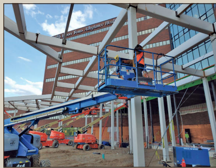
UNDERNEATH the new steel tube canopy at Henry Ford Allegiance-Jackson, Iron Workers Local 25 members employed by Douglas Steel weld joints for the new entrance. Leading the project are Local 25 foreman Dennis Douglas and steward Larry Lambaria.
