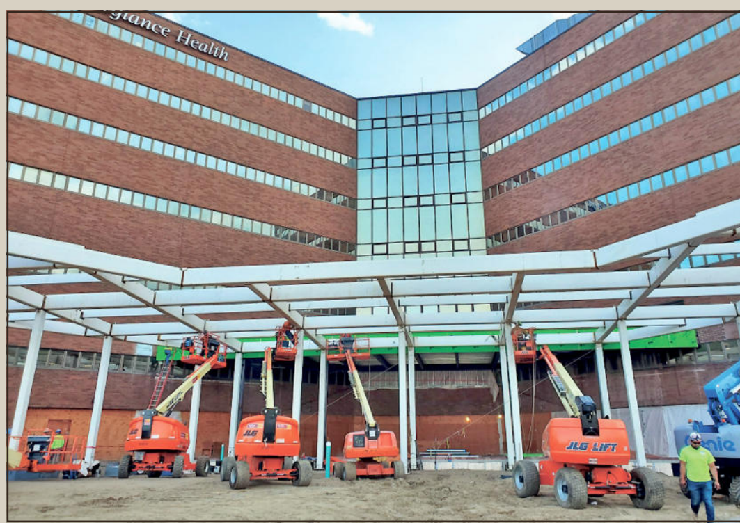
A TUBE STEEL CANOPY is erected last month at Henry Ford Allegiance Hospital in Jackson by members of Iron Workers Local 25, employed by Douglas Steel. Photo credits: Marc Crance
