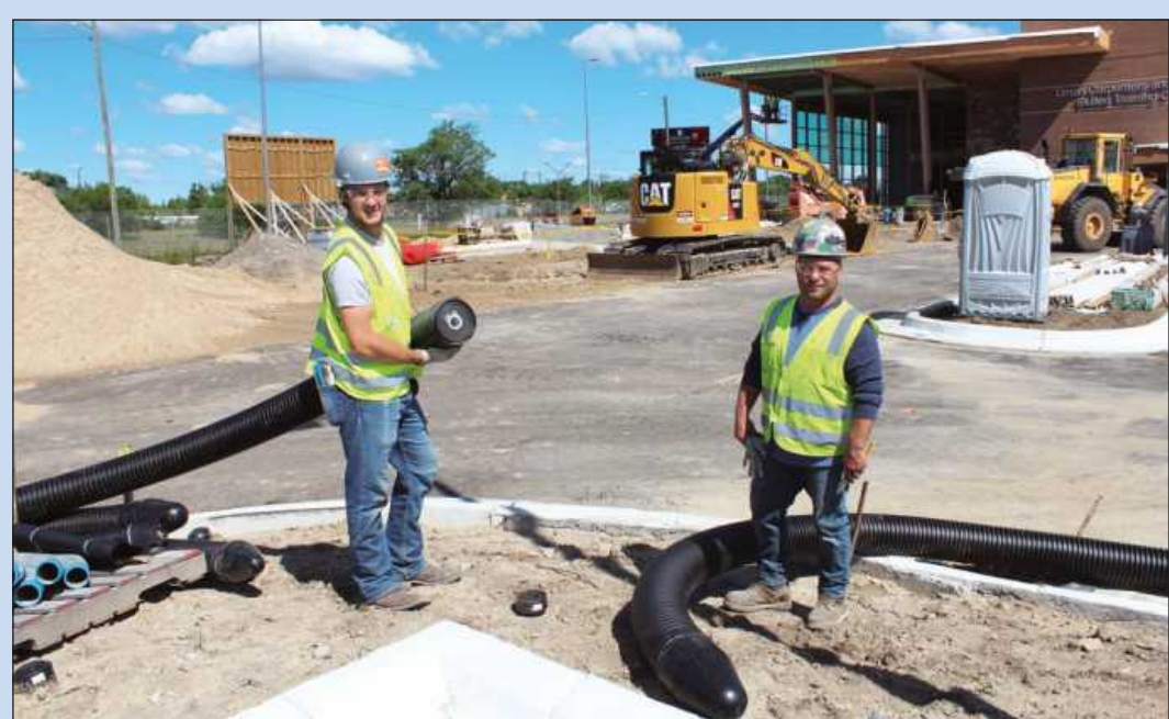
SNOWMELT TUBING that will be buried under pavement outside the Union Carpenters and Millwrights Detroit Training Center is handled by (l-r) Shawn Martin and Daryl Burke of Pipe Fitters Local 636. Employed by John E. Green, they are working with 13,000 feet of three-inch, insulated PEX tubing that will have glycol circulating through it.
