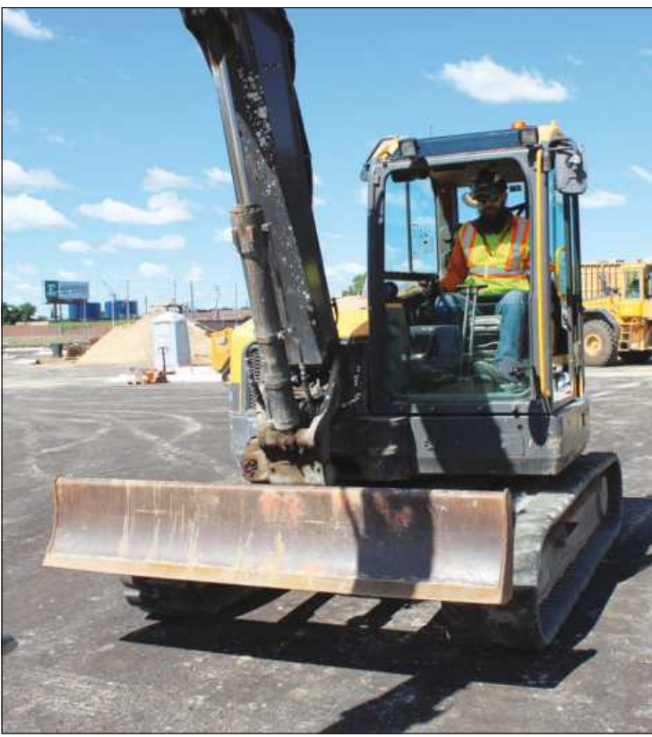
AT WORK IN his Volvo excavator "office" is Christopher Smith of Operating Engineers Local 324, working at the Michigan Carpenters Training Center in Detroit. He's employed by Blaze.
