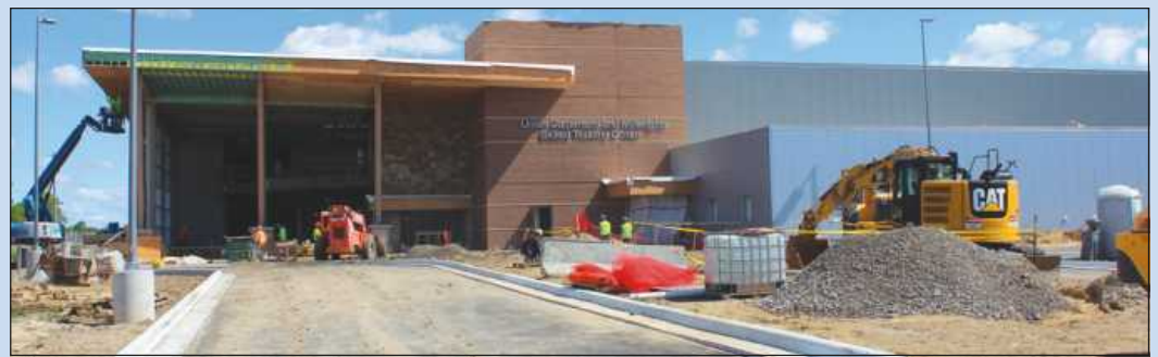
A NEW 144,000-SQUARE-FOOT facility that will house training and union offices for the Michigan Regional Council of Carpenters and Millwrights is nearing completion in Detroit. The project is being managed by Christman Construction. "Our new joint training center in Detroit will be our largest school in the state and will ensure Michigan's carpenters and millwrights are the most highly-skilled in the nation, ready to take on any job," said Tom Lutz, executive secretary-treasurer of the MRCC.
