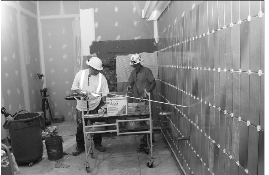
A FIRST FLOOR BATHROOM's tile is installed at the Michigan Carpenters Training Center in Detroit by (l-r) Tony Ramirez and John Lipka of Bricklayers and Allied Craftworkers Local 2. They're employed by Master Craft Tile.
