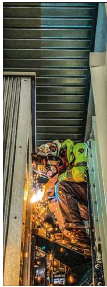
WELDING THE BURNER BOX to the boiler at Graphics Packaging in Kalamazoo is a cramped Tyler Karoly of Boilermakers Local 169. He's employed by Barton Malow.
