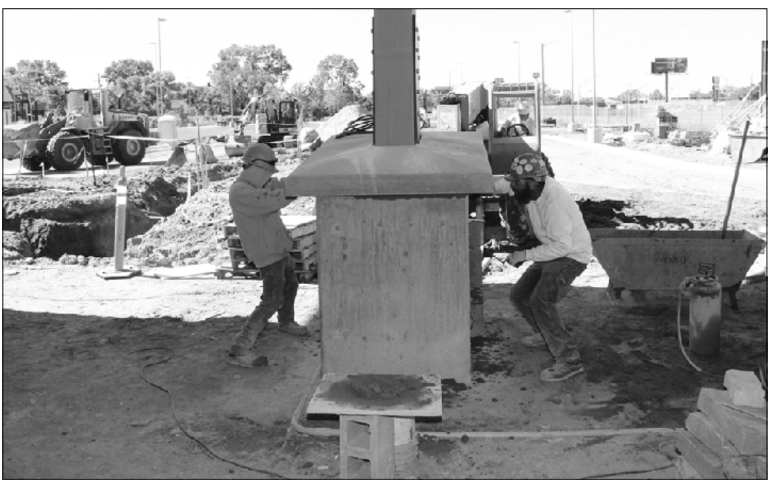
SETTING A CAPSTONE of "Castle Stone" to decorate a pier in front of the Carpenters Training Center in Detroit are (l-r) C.J. King and Shawn Fox. The Bricklayers and Allied Craftworkers Local 2 members are employed by Leidel and Hart.
