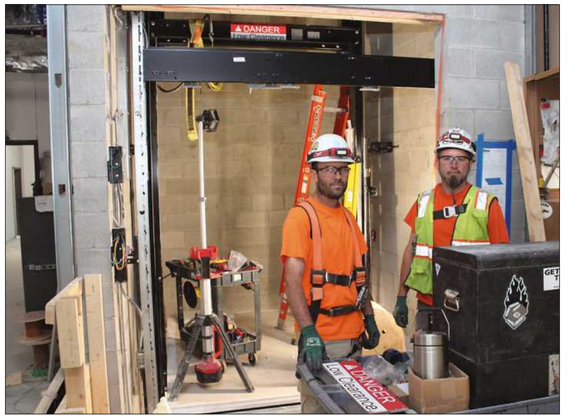
OUTSIDE THE CAB they're installing on the first floor of the Michigan Regional Council of Carpenters and Millwrights Training Center in Detroit are (l-r) Justin Mckoan and Jud Burns of Elevators Constructors Local 36. They're employed by TK Elevator.
