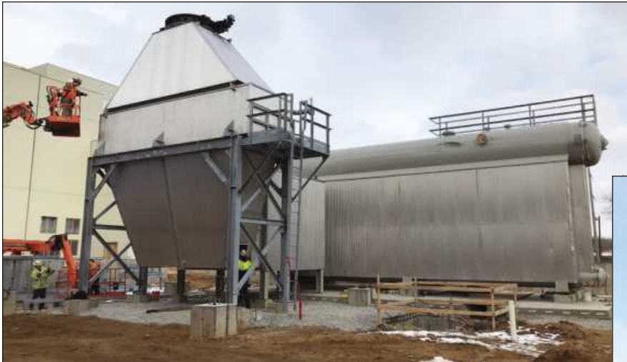
ASSEMBLING THE ECONOMIZER for the boiler at Graphics Packaging in Kalamazoo are Superintendent Russ Lewis, Foreman Sean Mckellip and Steve Toman and Jeremy Seaman. The Boilermakers Local 169 members are employed by Barton Malow.
