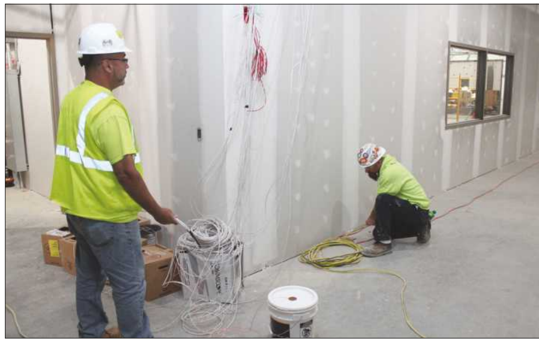
PULLING CARD ACCESS CABLE at the Detroit Carpenters Training Center are (l-r) Rick Torres and Loneal Oliver. The IBEW Local 58 members are employed by Bluestone Communications.
