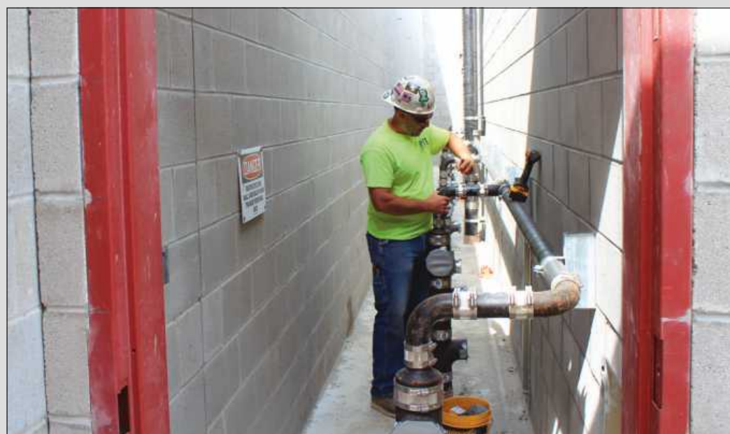
SETTING A TWO-INCH vent line that serves four-inch drains at the back of a cell block at the Genesee County Juvenile Justice Center is Jon Cook of Plumbers and Pipe Fitters Local 370. He's employed by Platinum Mechanical.
