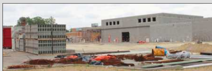
BLOCKLAYERS from BAC Local 2 and Davenport Masonry are extremely active at the Genesee County Juvenile Justice Center, building much of the facility's structure out of reinforced concrete block.
