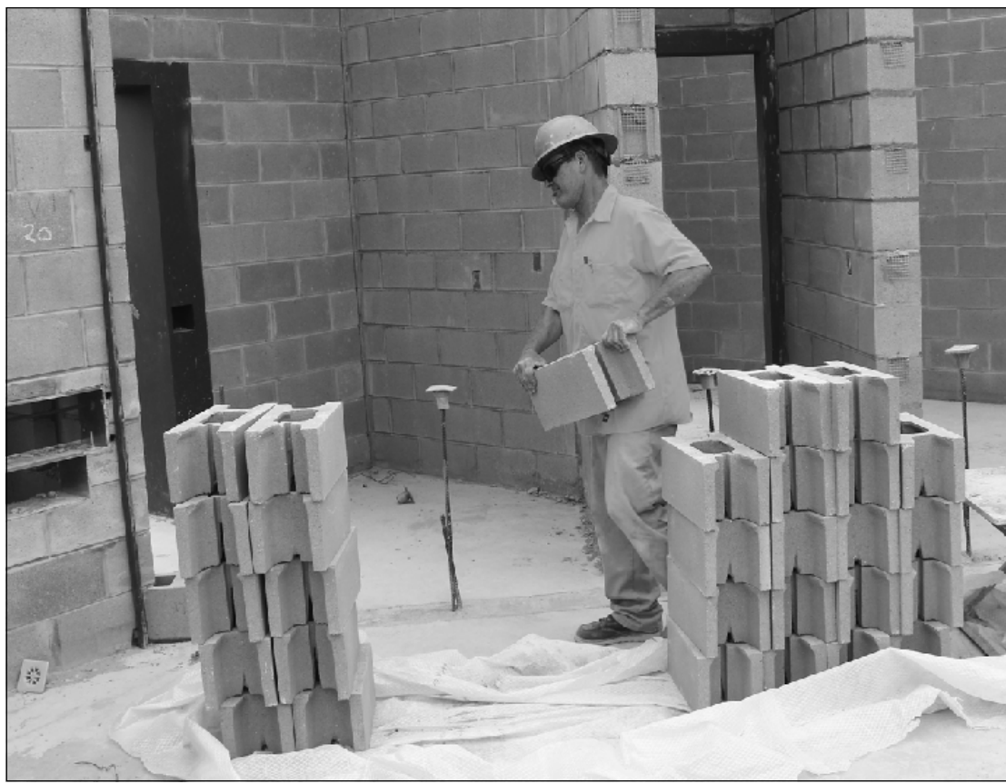
HEFTING A BLOCK while working at the Genesee County Juvenile Detention Facility in Flint Twp. is Mike Piazza of Bricklayers and Allied Craftworkers Local 2. He's employed by Davenport Masonry.
