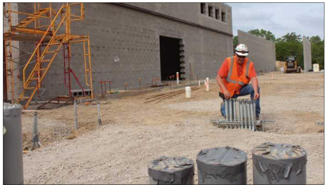
ELECTRICIAN Amos Knapp measures conduit stubs that will go into electric panels at the Genesee Juvenile Justice Center. The IBEW Local 948 project foreman is employed by Superior Electric.
