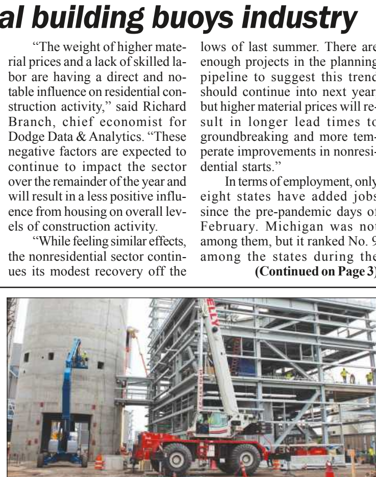
IN 2013, THE BUILDING TRADES installed spray dry absorbers onto Consumers Energy's Karn Units 1 and 2 in order to reduce sulfur dioxide emissions at the plant, in a $250 million project. The coal-burning units will be retired in 2023. Tradesman file photo
