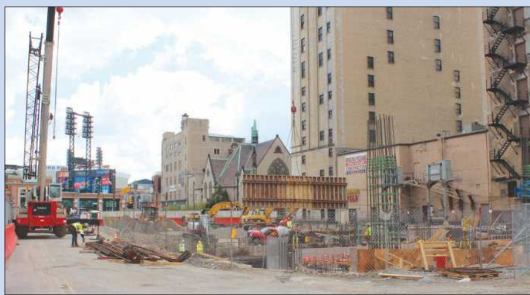
A COMERICA PARK light tower looms in the background across Woodward Avenue in Detroit, as building trades workers toil on the underground work for a new TCF Bank building.
