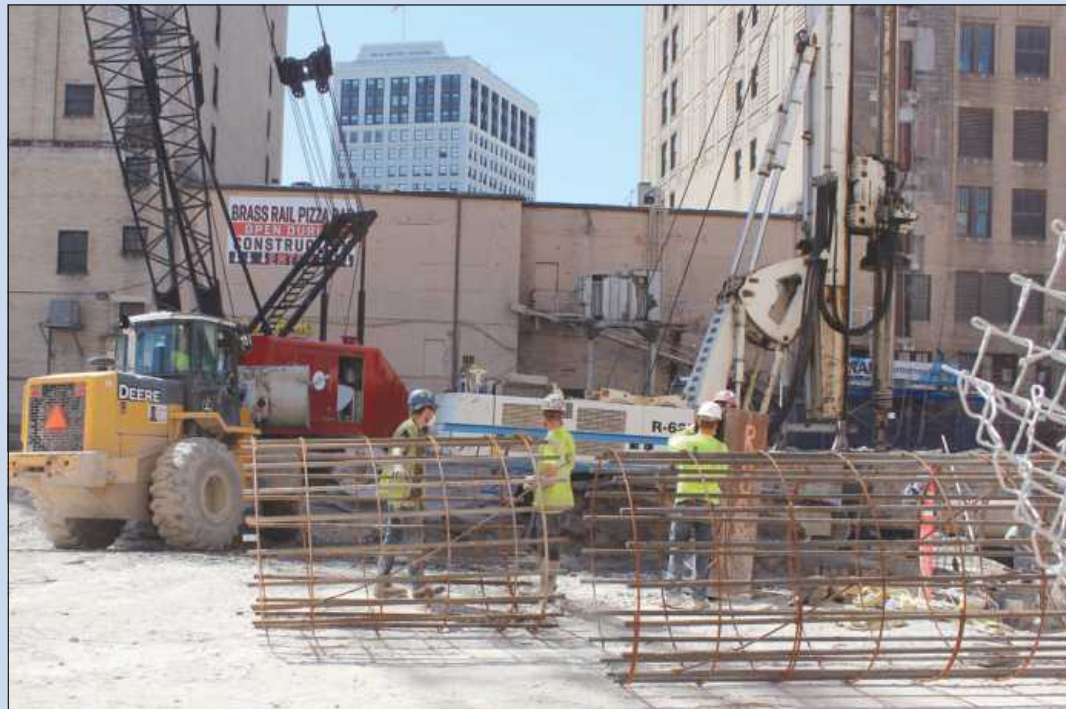
AT WORK AT THE TCF Bank project in Detroit at Woodward and Elizabeth are Laborers Charles Blasidell (Local 1076) Kent Laskowsky and Dave Cotcher (both Local 1191). They're employed by Rohrscheib Sons Caissons, Inc.
