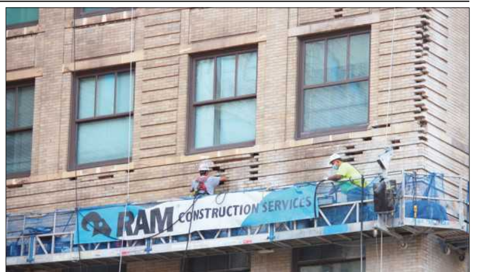
BRICKLAYERS and Allied Craftworkers Local 2 members employed by Ram Construction repair the facade of the 19-story Grand Park Centre Building in Detroit's Grand Circus Park.
