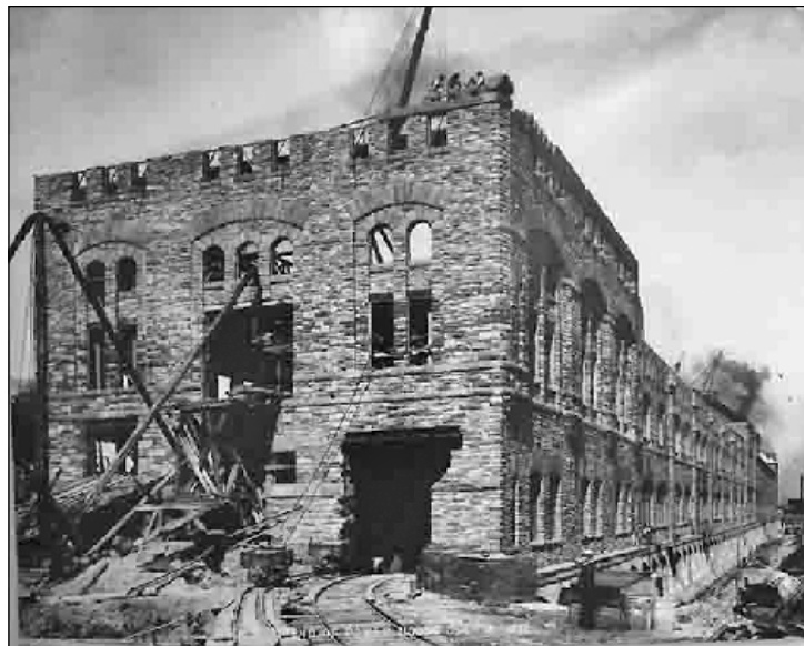
CONSTRUCTION OF quarter-mile long Edison-Sault Electric Co.'s hydroelectric plant began in 1887 in Sault Ste. Marie. Masons erecting the beautiful structure using sandstone they were excavating nearby from the St. Mary's River. Operational since 1902 and capable of 25-30 megawatts of electricity, the plant was erected with a hopeful "if you build it they will come" business plan for attracting employers to the region. The plan largely failed — but the plant has remained functional since it was built. Photo credit: Power
