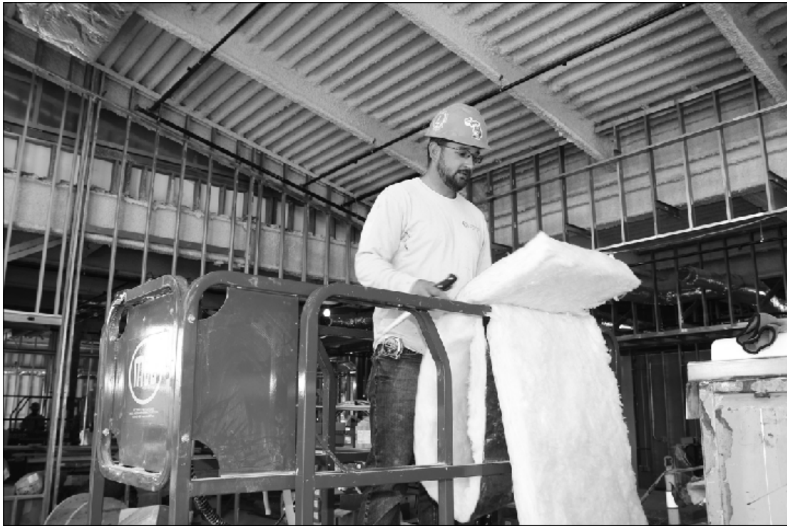
CUTTINGAN INSULATION BATT to insulate ductwork at the Mary Free Bed project at Saginaw's Coventant Health campus is Curtis Grigonis of Heat and Frost Insulators Local 47. He's employed by T & C Insulation.
