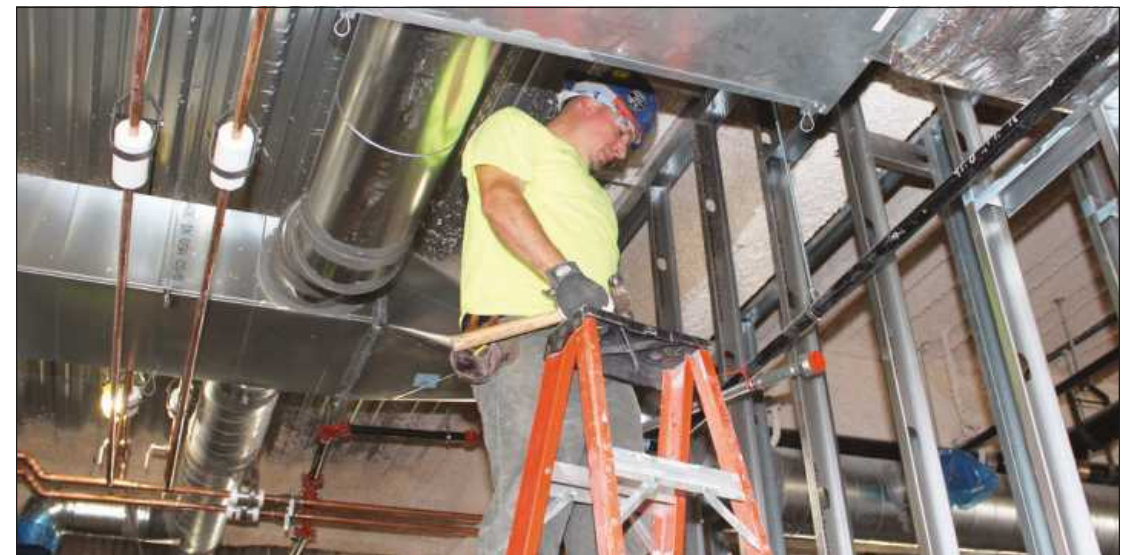
SETTING PIPE HANGERS on the first level of the Mary Free Bed project in Saginaw is Greg Donahue of Plumbers and Steamfitters Local 85. He's employed by Johnson and Wood.
