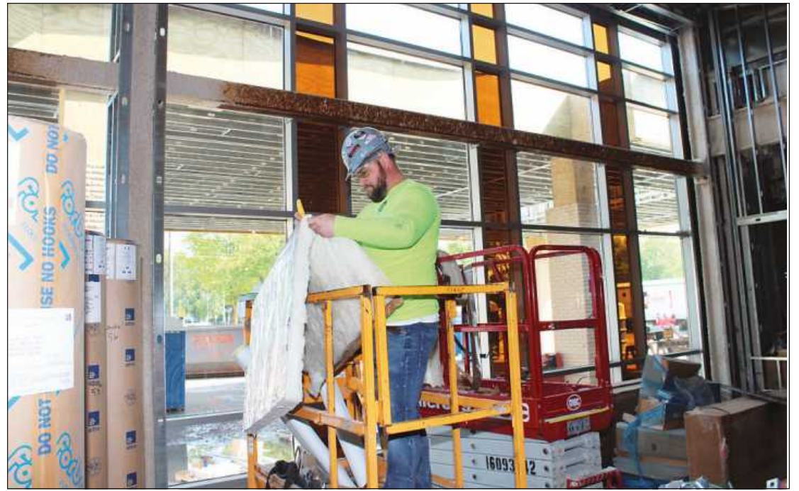
CUTTING AN INSULATION BATT to wrap a duct at the Mary Free Bed project at Covenant Health in Saginaw is Jason Jones of Heat and Frost Insulators Local 47. He's employed by T & C Insulation.
