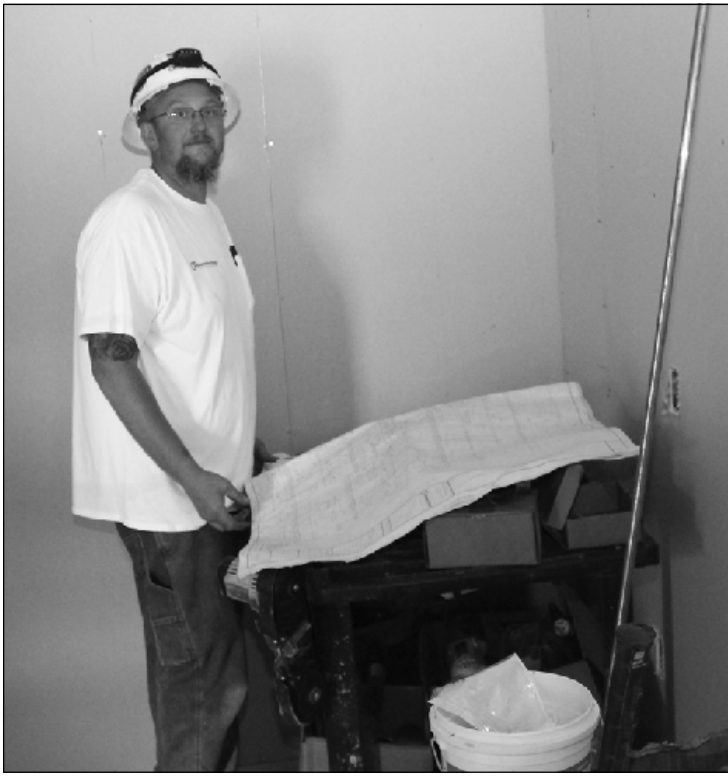
CHECKING BLUEPRINTS at the Mary Free Bed Project in Saginaw is Matt Nietling. The Plumbers and Steamfitters Local 85 member is a foreman for Johnson and Wood.
