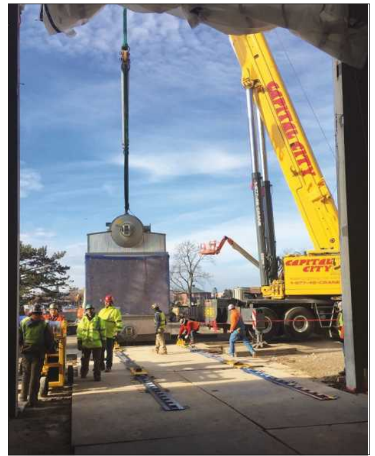
THE BOILERMAKERS Local 169/Monarch Welding and Engineering crew line up the boiler for transfer into the building at the Ford Central Energy Plant in Dearborn.
