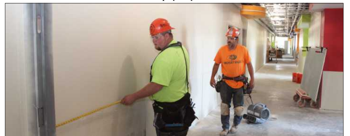
SETTING UP VINYL wall protection product on a second-floor hallway at the Mary Free Bed project in Saginaw are (l-r) carpenters Grant Lentner and Jeremy Cleary, both of Michigan Regional Carpenters Council Local 706. They're employed by Spence Brothers.
