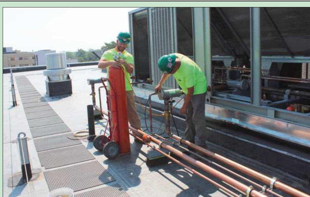
ON THE ROOF of the Mary Free Bed building on Saginaw’s Covenant Hospital campus are Brad Bolzman and Jeff Greaves of Plumbers and Steamfitters Local 85. Employed by Johnson and Wood, the mechanical equipment service journeymen are pressure-testing the 100-ton air conditioning unit with nitrogen.
