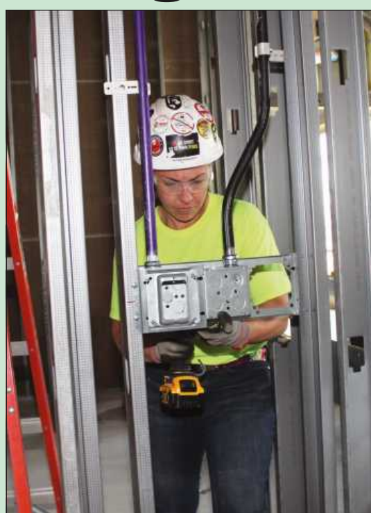
SETTING A CARD READER box on the first floor of the Mary Free Bed building in Saginaw is electrician Breanna DePottey of IBEW Local 557. She’s employed by Clements Electric.
