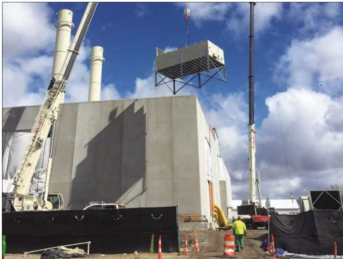
SETTING THE TURBINE fresh air inlet filter box at the Ford Central Energy Plant project in Dearborn are Local 169 Boilermakers employed by Monarch Welding and Engineering.
