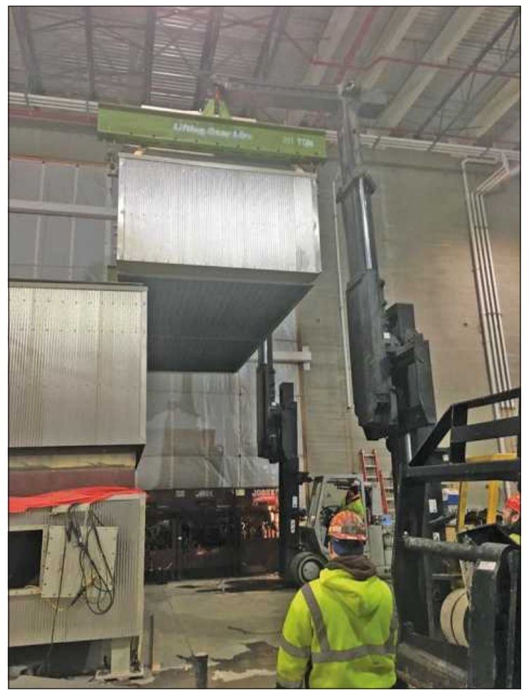
SETTING THE ECONOMIZER section at the Ford Central Energy Plant are Local 169 Boilermakers, including Jason Beaudin.
