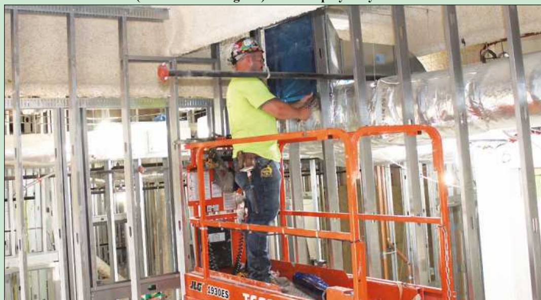
SETTING A REGISTER on the first floor of the Mary Free Bed project in Saginaw is Ricky Berwick of Sheet Metal Workers Local 7. He’s employed by U.S. Sheet Metal.
