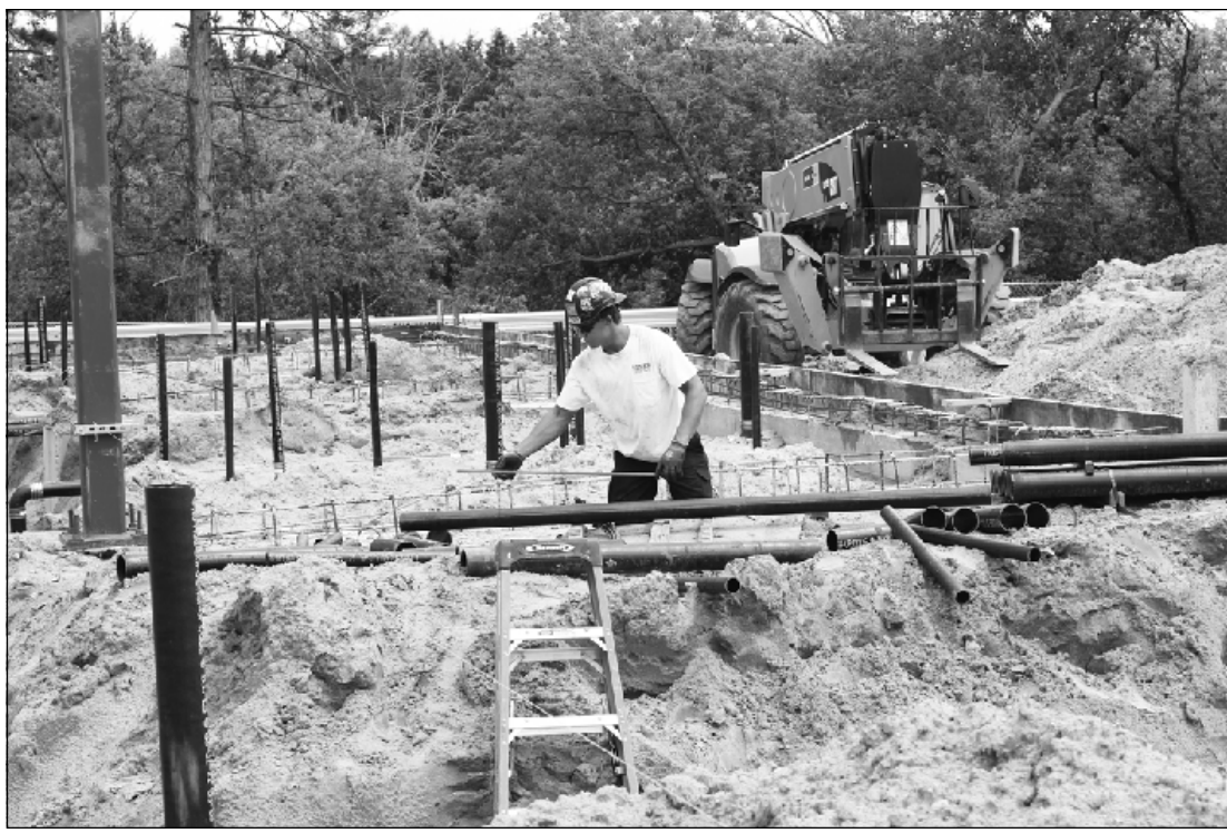
TAKING THE MEASURE OF cast iron pipe that will be buried at the Caro Psychiatric Hospital project is Bailey Hientz, a Plumbers and Steamfitters Local 95 apprentice. He's employed by Remer Plumbing, Heating and Air Conditioning.
