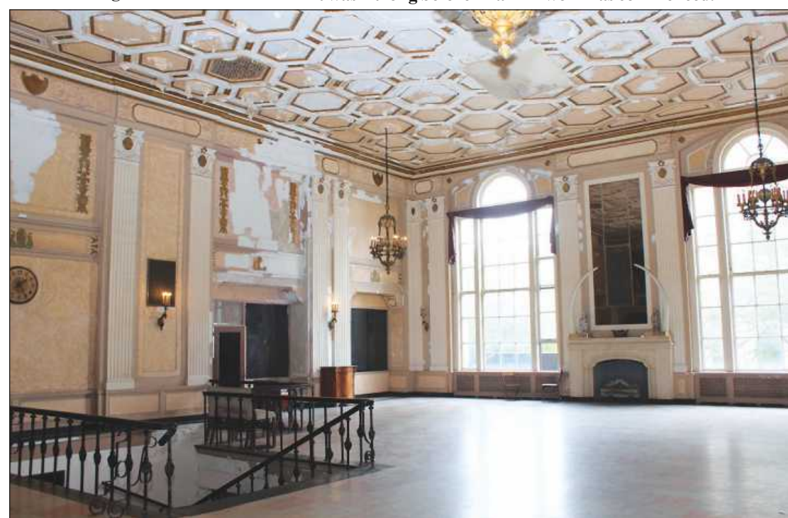
THE INTERIOR OF a ballroom at the Leland, last month. Aside from peeling paint and some cosmetic issues, it appears to be in good shape.
