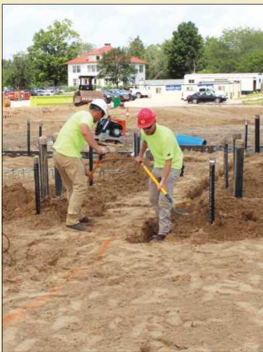
ELECTRICIANS (l-r) Garrett Link and Joe Waters create a trench for conduit while working at the Caro Psychiatric Hospital project. The IBEW Local 557 members are employed by Master Electric.
