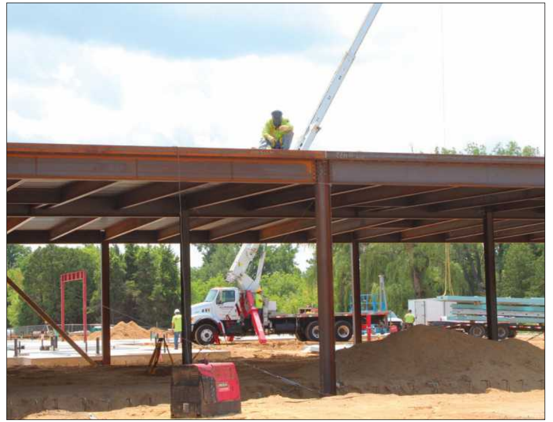
WELDING AT THE CARO Psychiatric Hospital is Ricky Oliver of Iron Workers Local 25. He's employed by Tri-Steel. The first structural steel on the project was coming out of the ground late last month.
