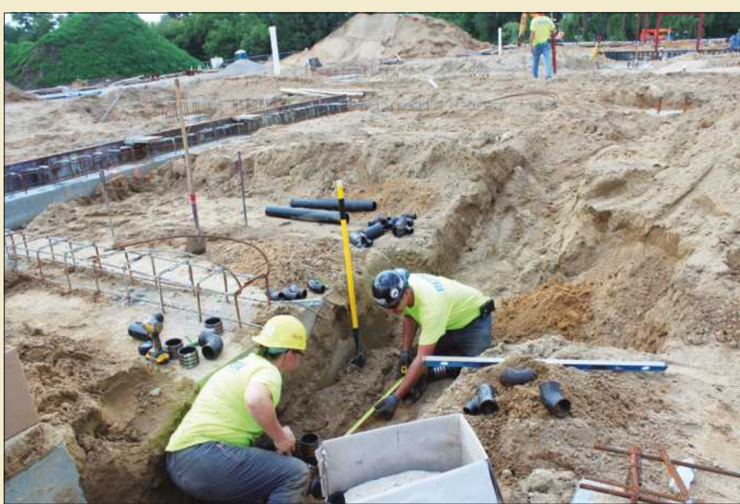
PLUMBERS Alicia Barr and Jason Golden place four-inch cast iron sanitary pipe while working at the new Caro Psychiatric Hospital project, which is obviously just coming out of the ground. The Plumbers and Steamfitters Local 85 members are employed by Remer Plumbing, Heating and Air Conditioning.
