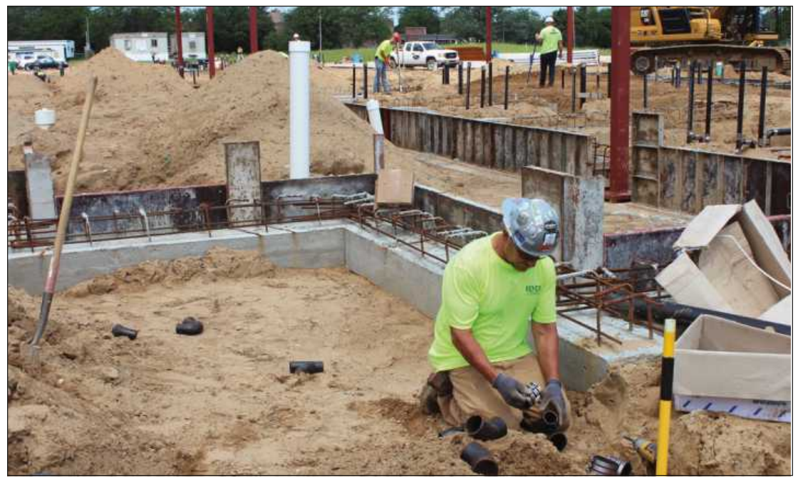
SETTING THREE- AND FOUR-INCH pipe sections while working at the Caro Psychiatric Hospital project is Terry Kubczak of Plumbers and Steamfitters Local 85. He's employed by Remer Plumbing, Heating and Air Conditioning.
