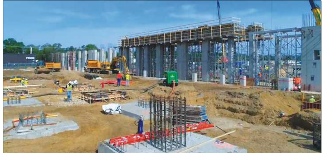
THE GRAPHICS PACKAGING project is being erected on the old Checker Motors plant site in Kalamazoo. Photo credit: Graphics Packaging
