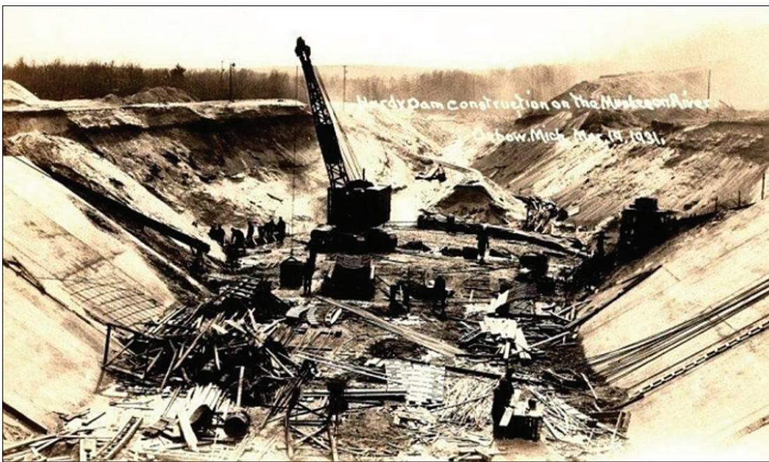
CONSTRUCTION OF THE Hardy Dam on March 19, 1931. At one point the embankment stretches 2,600 feet across the Muskegon River. Photo credit: Bentley Library, University of Michigan
