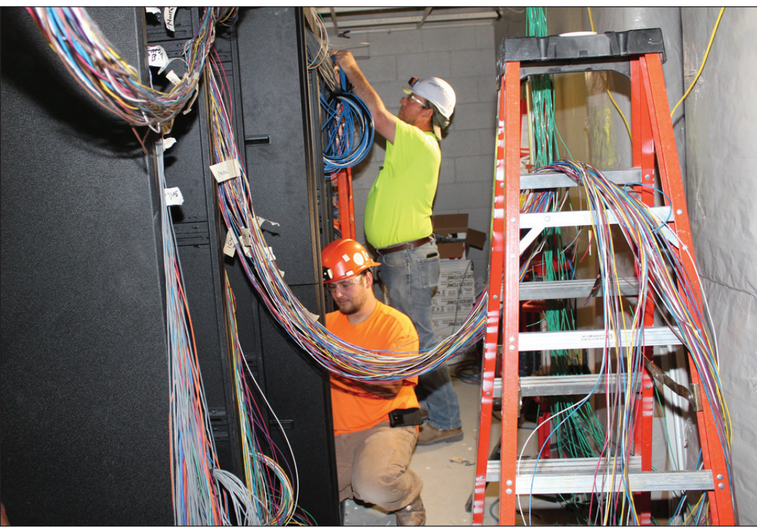
BUNDLES OF programmable logic control wiring at the Branch County Jail project are organized and terminated by electricians Brandon Hillman and Tom Densmore. The IBEW Local 445 members are employed by Hayes Electric.
