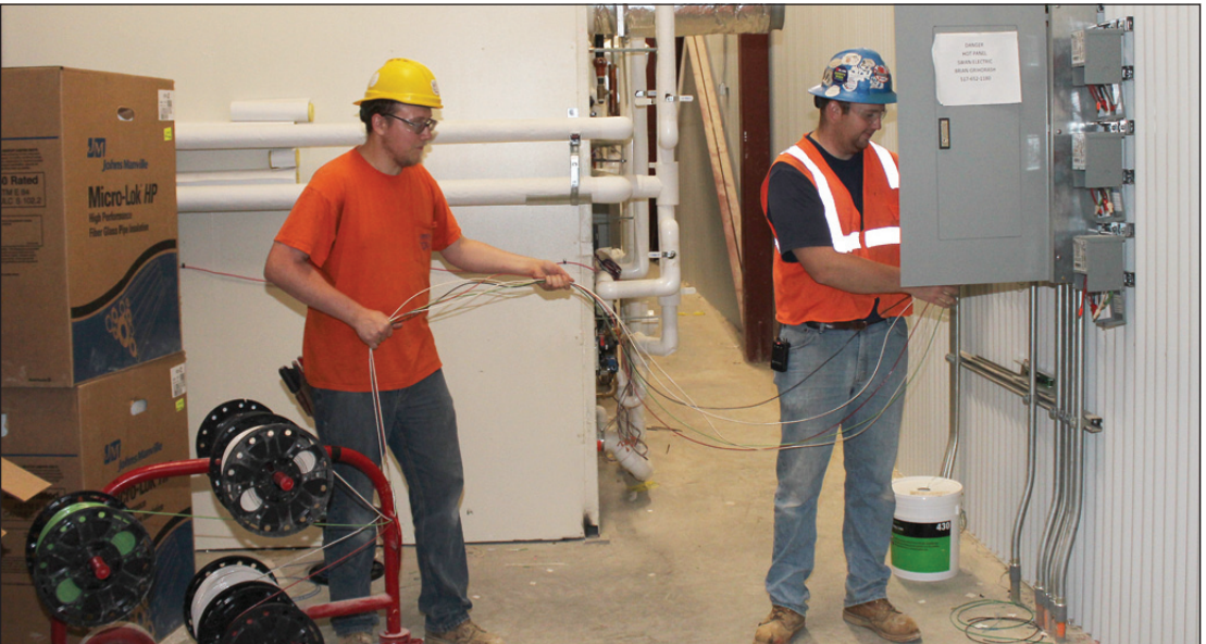
PULLING NO. 12 THHN cable to a panel at the Branch County Jail project in Coldwater are (l-r) Forrest Frantz and foreman Chad Beuerle of IBEW Local 445. They're employed by Swan Electric.
