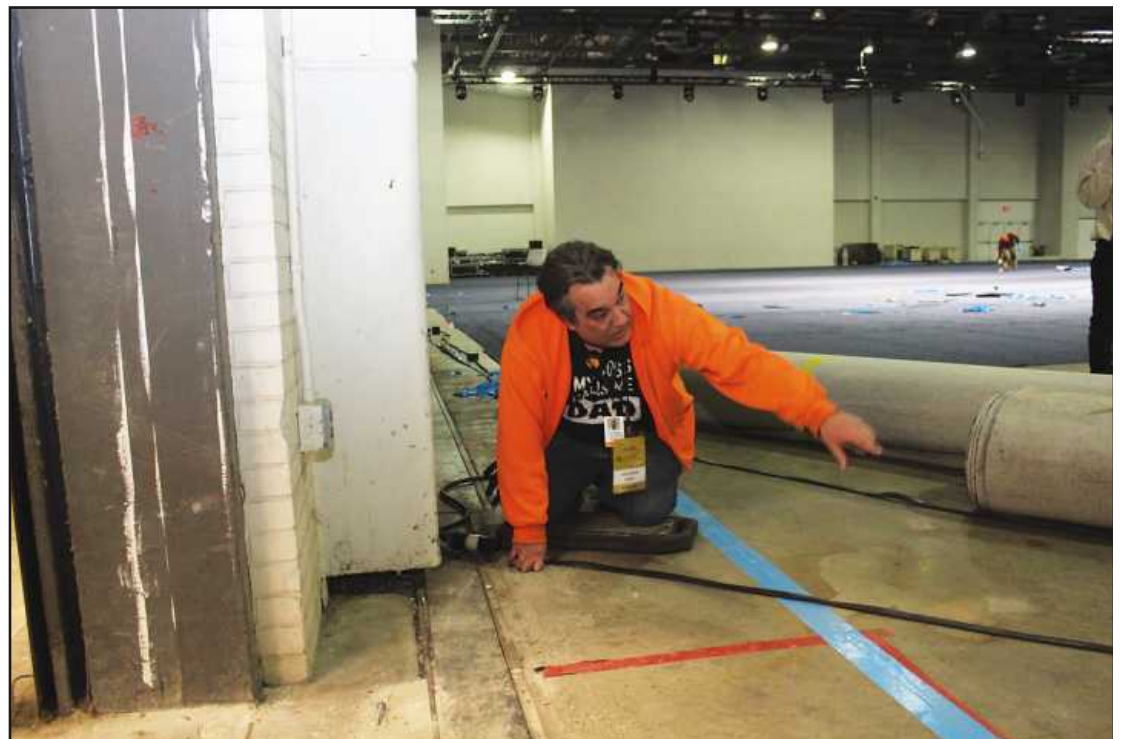
ELECTRICIAN Jeff Trimble sets temporary wiring in an annex at Huntington Place in Detroit while helping to set up the Detroit Auto Show.
