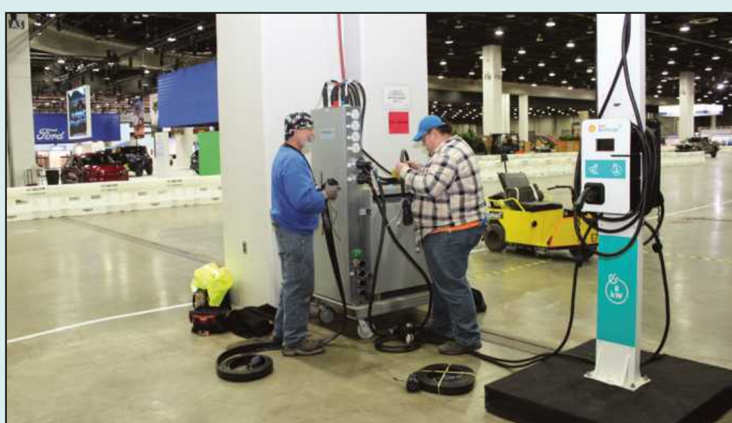
SETTING UP an electric vehicle charging station at Huntington Place in Detroit are (l-r) electricians Scott Reinbold and Michael Monterosso. The IBEW Local 58 members, employed by Freeman Electric, are working to set up the Detroit Auto Show. The chargers would be used to power up vehicles used on a track as part of the show.
